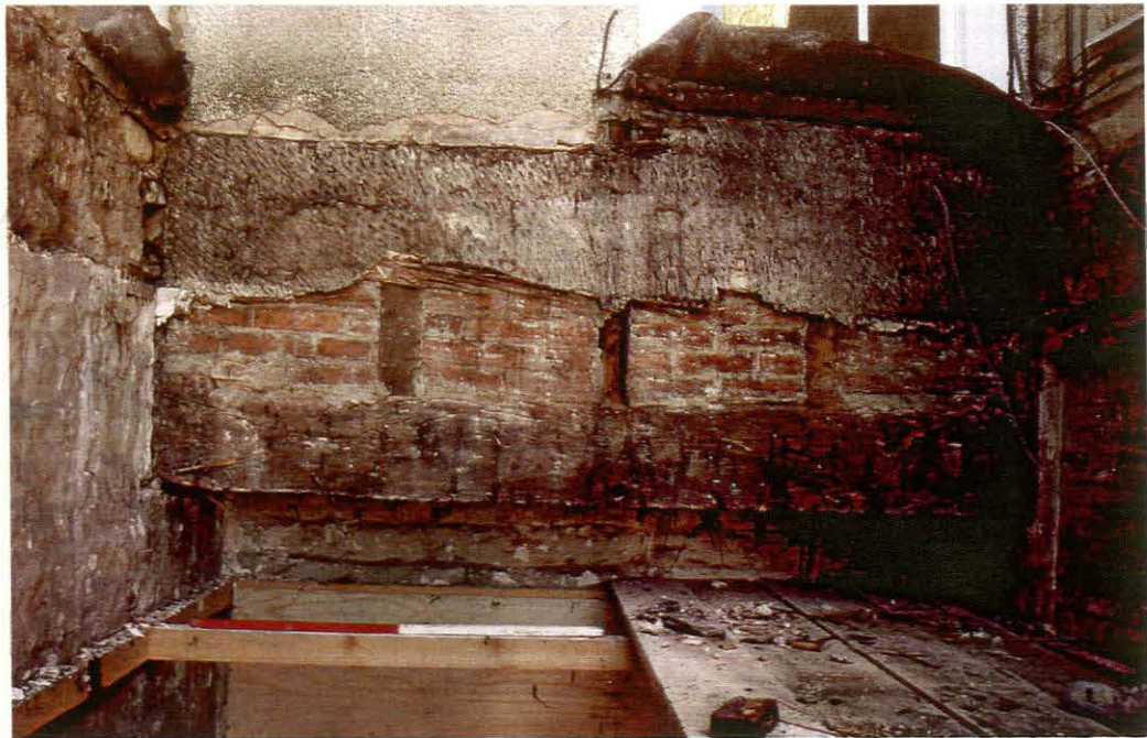
Plate 2 - View showing the bressumer, the timber studs and brick nogging, looking west
