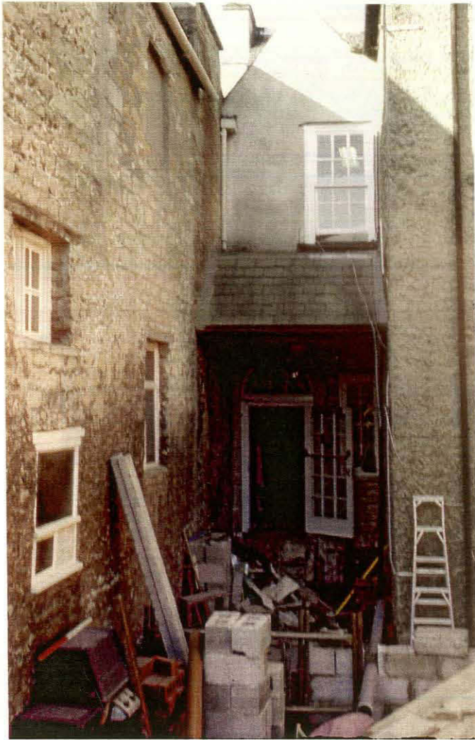
Plate 1 - View of the development area prior to the removal of the porch, looking west
