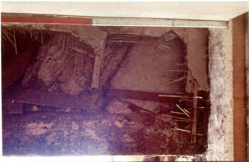
Plate 3 - View of the underside of the jetty showing floorboard and joist layout
