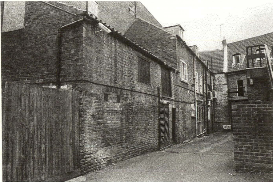
Plate 29 Centre and Western Part of North Side of North Wing, looking southwest
