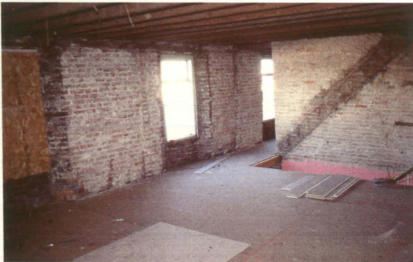
Plate 7 Upper Floor, area of West End Shop and Stairwell, showing scar of removed stairs, looking northeast
