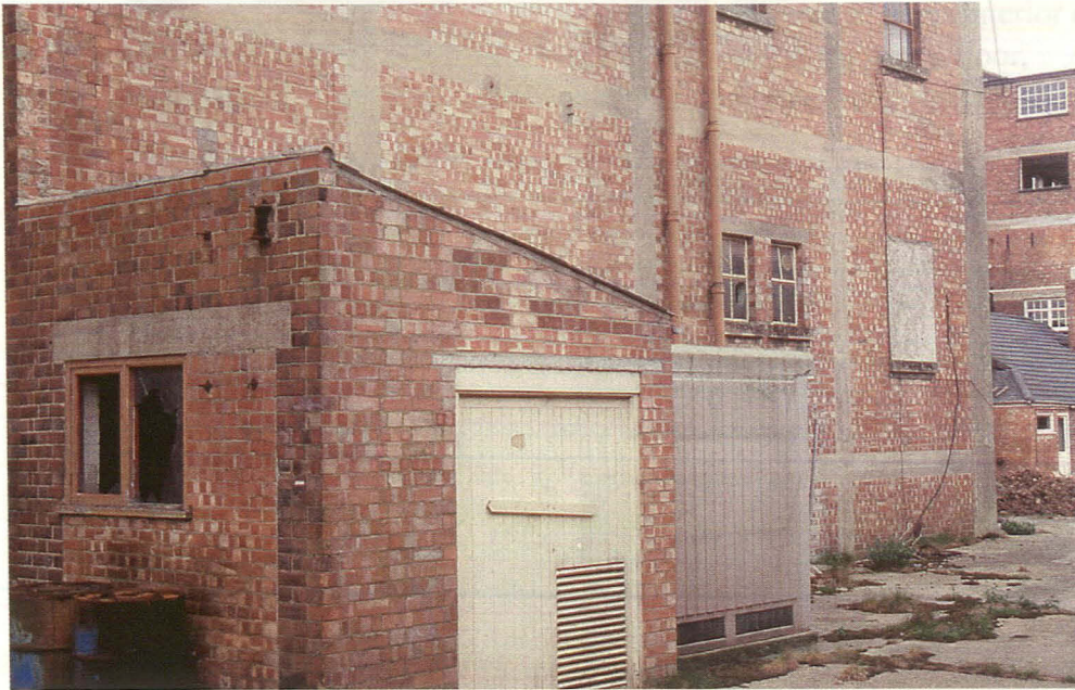
Plate 5 Detailed view of the additional structure and electric substation on east elevation of Warehouse 1.
