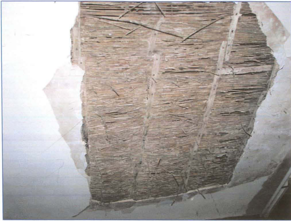
Plate 19: (057) The reed base, for lime ash flooring in Room 9, exposed in the ceiling of Room 6.
