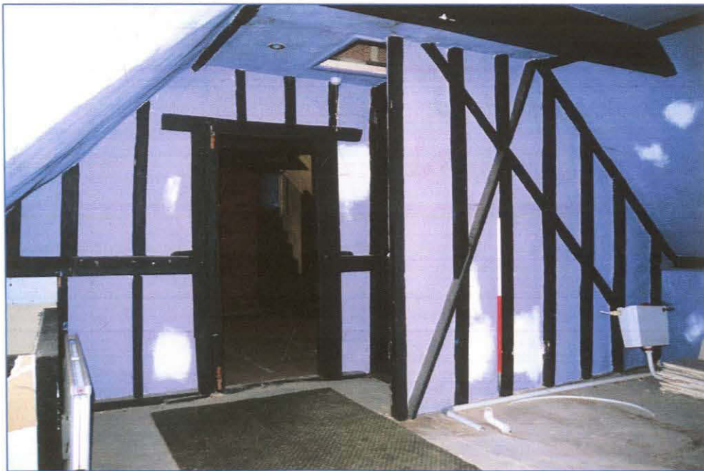
Plate 26: (085) Room 15. The 18 th century type doorframe in the southern wall of this room is constructed in heavy timbers that form part of the roof superstructure. It has an expanded lintel that is secured to the jambs with pegged mortice and tenon joints supporting timber studding to the apex of the roof. An original latch hoop is still attached to the north side of the frame. A partition wall of timber uprights with cross bracing may have enclosed what may have been the original internal staircase access. Looking south-east.
