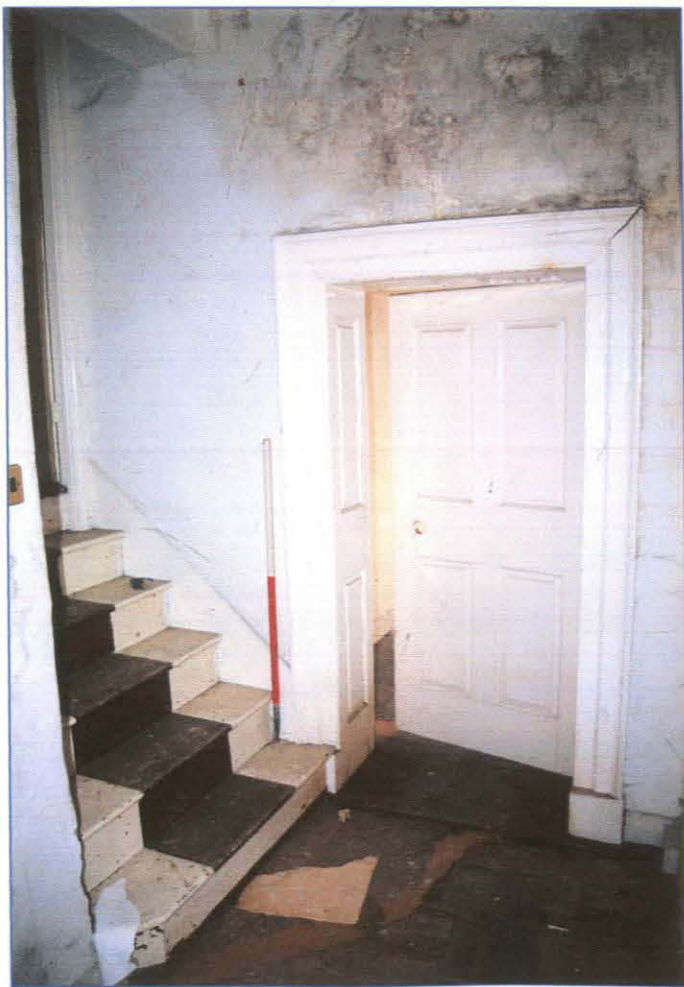
Plate 12: (074) On the first floor, rooms have doors that are four panel raised and fielded within a boxed, paneled frame with architrave. Shot depicts the door of Room 10 taken from the western half landing facing south.
