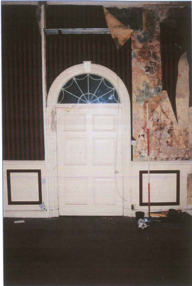
Plate 15: (036) The courtroom is accessed via a six panel door with an Adam Style fanlight header, framed by architrave with keystone detail on both sides of the door frame. This shot also demonstrates the level of water damage to the interior of the building. Looking east.
