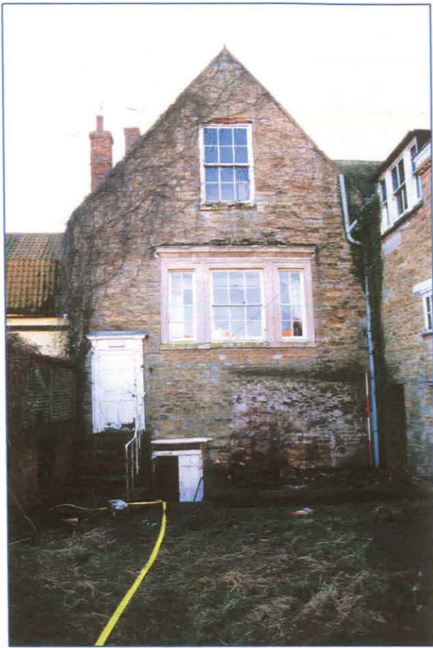
Plate 5: (014) North elevation of the courtroom showing the high level moulded stone window and rear access steps with steps down to the cellar doorway. Looking south
