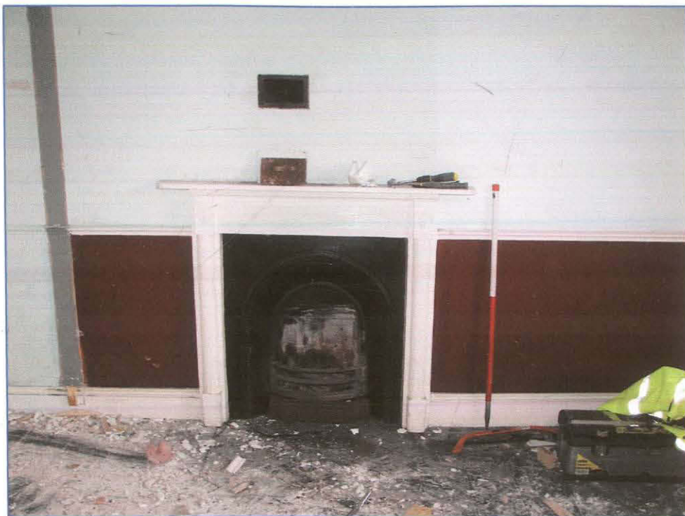
Plate 9: (shot 113) Room 16 retains a mid 19 th century cast iron arched register grate that has a Regency style fire surround with concentric bosses and reeded moulding. Looking east.
