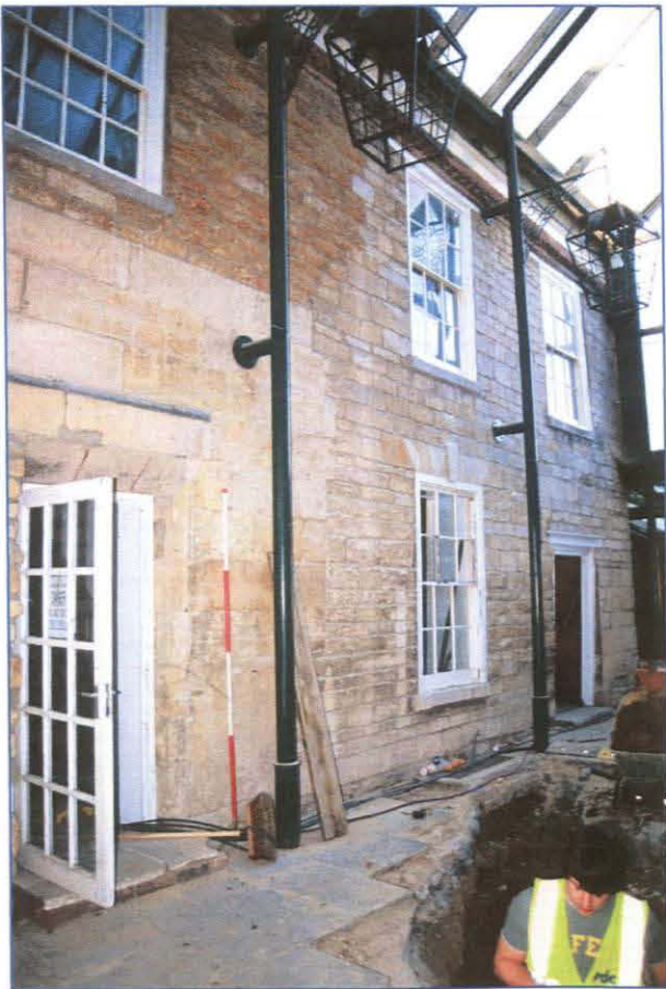
Plate 6: (026) Eastern elevation of the Western Range (South Block) illustrating the changes in wall fabric associated with phases of development. Looking north-west
