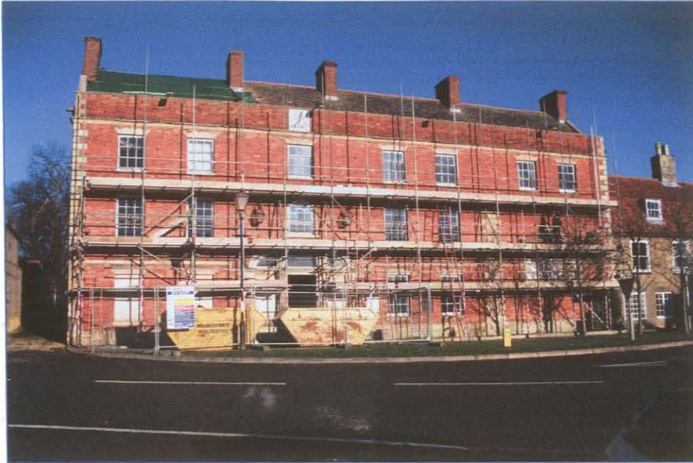
Plate 1: (001) Southern façade of the Greyhound Inn demonstrating the limitations upon photographic recording. Looking north.
