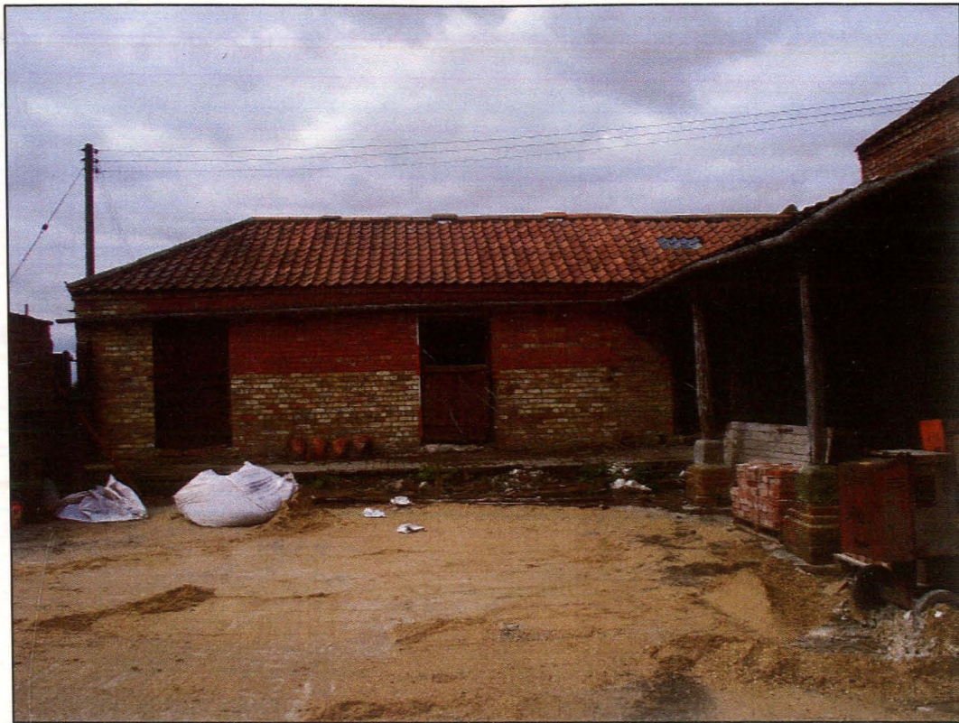
Plate 13 (Shot 30): East-north-east facing elevation with raised walkway of the western range of Block B, looking west-south-west
