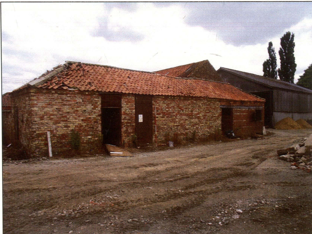
Plate 36 (Shot 23): East-north-east facing elevation of the eastern range of Block B showing openings to barn B10, store B11, access to crew yard and an opening to the grain dryer B7. Looking north-west
