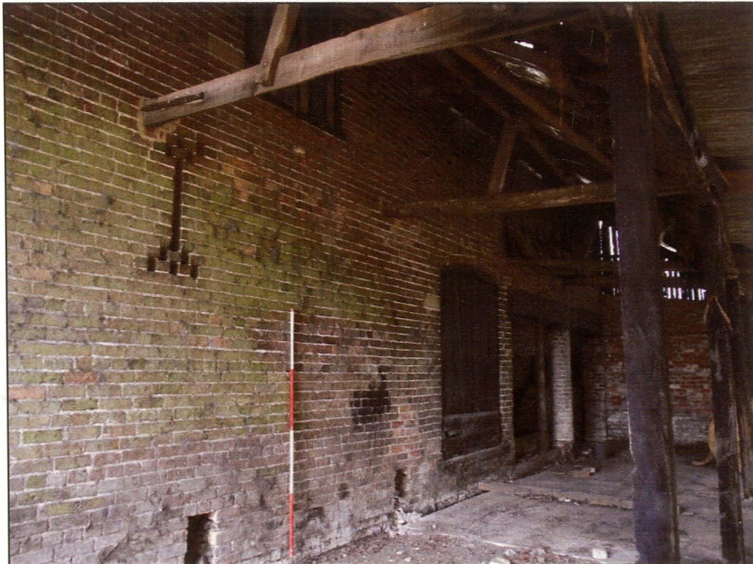
Plate 28 (Shot 66): North-north-west elevation of the middle range of Block B showing lean-to roof structure, northern entrance to the threshing barn and barn B6. Also note the pitching hole under the eaves of the threshing barn as well as the decorative ventilation slit
