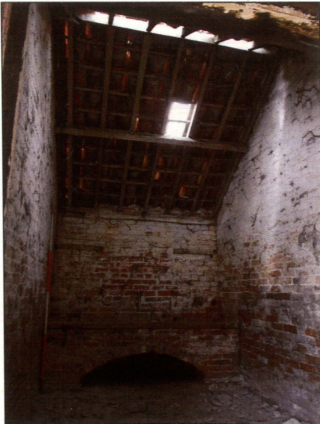
Plate 20 (Shot 46): Interior of barn B3 showing roof structure, broken cement floor and feeding trough. Looking west-south-west
