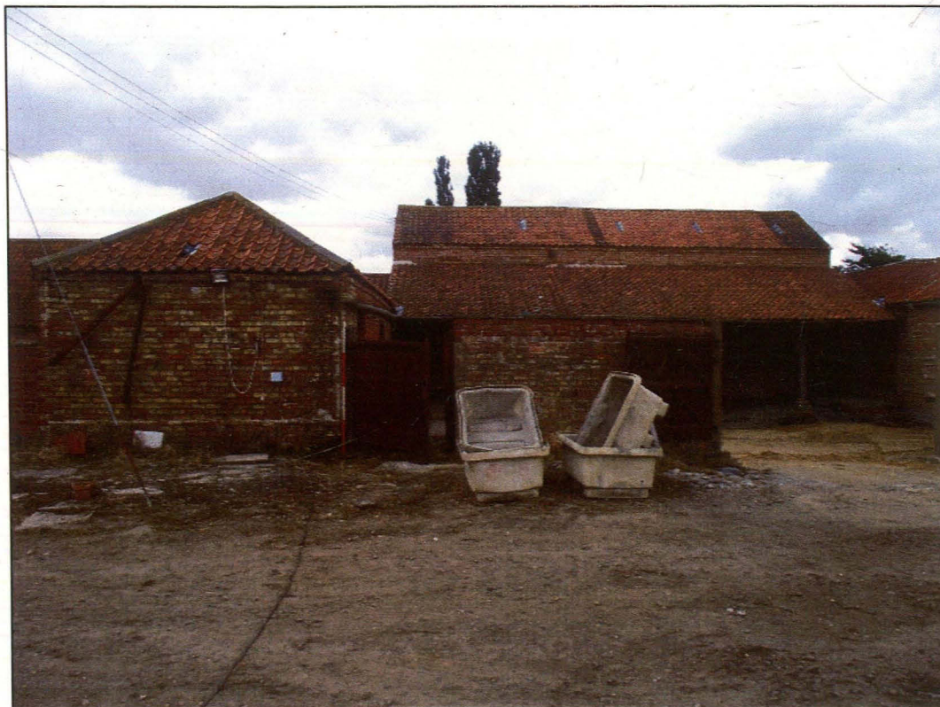
Plate 14 (Shot 21): General shot of south-south-east elevation of the western range. A clear glass pantile has been used to repair the roof. Looking north-north-west
