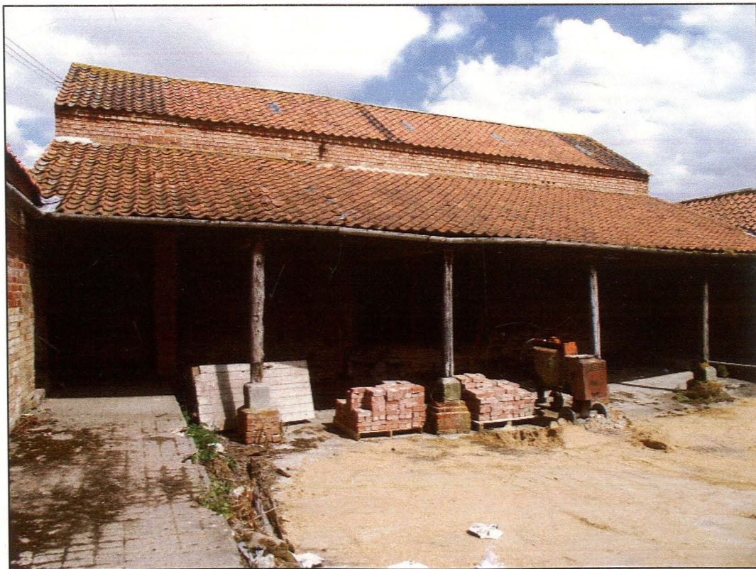
Plate 24: (Shot 37): South-south-east facing elevation with lean-to of the middle range of Block B. Looking north
