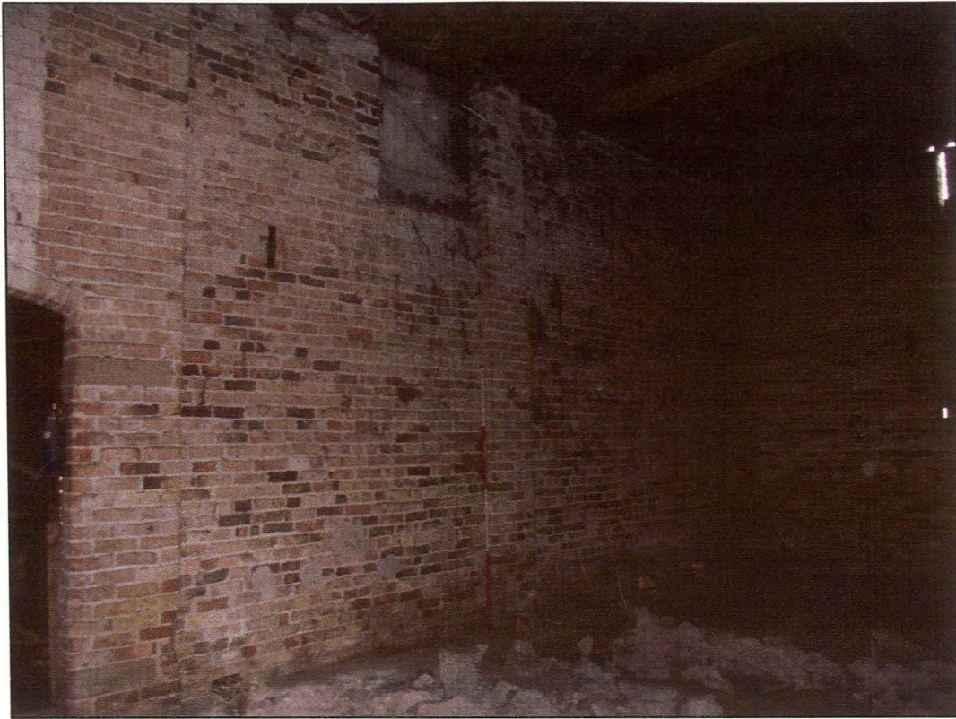
Plate 31 (Shot 57): North-north-east elevation of threshing barn with a pitching hole and a brick buttress to its right. Looking north-north-east
