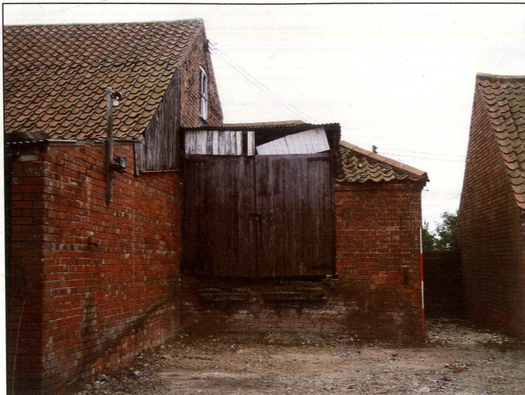
Plate 17 (Shot 27): North-north-west elevation of western range of Block B. The adjacent elevation of the lean-to shows scarring of a modern ramp that was recently removed. This shot also shows the recently raised roof above the double barn door. Looking south-south-east
