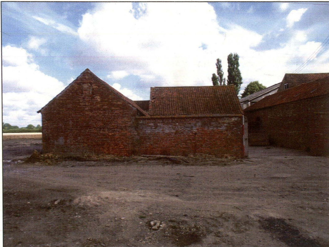
Plate 2 (Shot 8): South-south-east elevation of Block A with brick repair on the gable of A1, looking north-north-west
