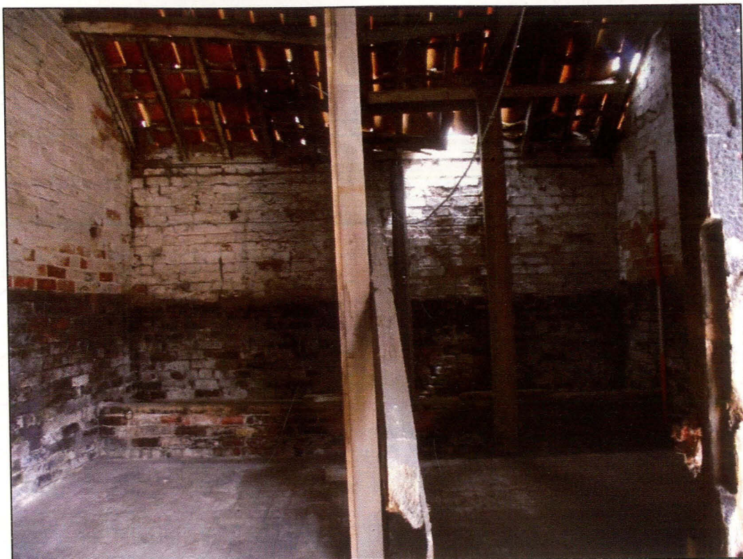
Plate 39 (Shot 75): Interior shot of barn B8 with broken roof structure and raised floor with a feeding trough at the far end. Looking east-north-east
