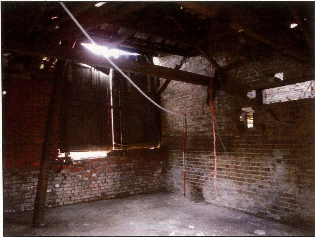
Plate 21 (Shot 48): Interior of barn B4 showing collapsing roof and machinery opening on the west-south-west facing elevation. Looking north-north-east
