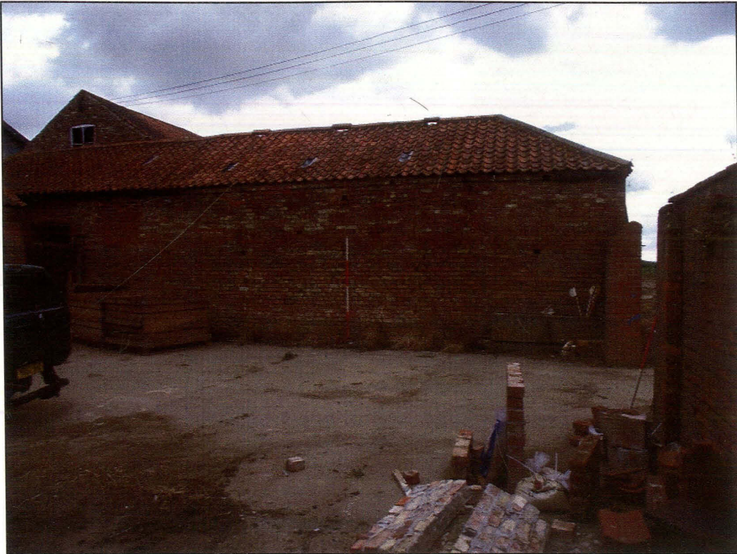
Plate 15 (Shot 20): West-south-west facing elevation of the western range of Block B showing recent brickwork repair adjacent to door, looking north-east
