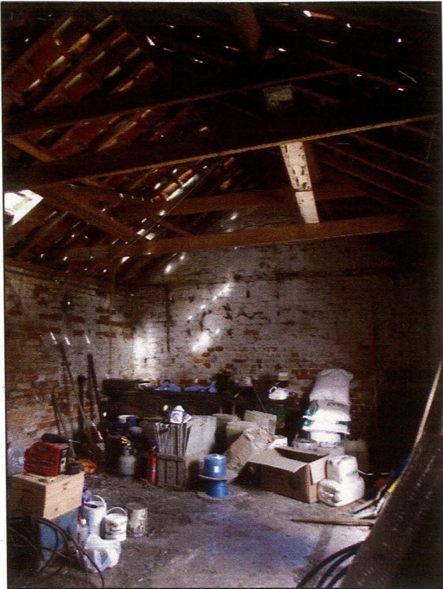
Plate 19 (Shot 44): General shot of store B2 interior showing roof structure and the north-north-west to south-south-east aligned floor gutter. Looking north-west
