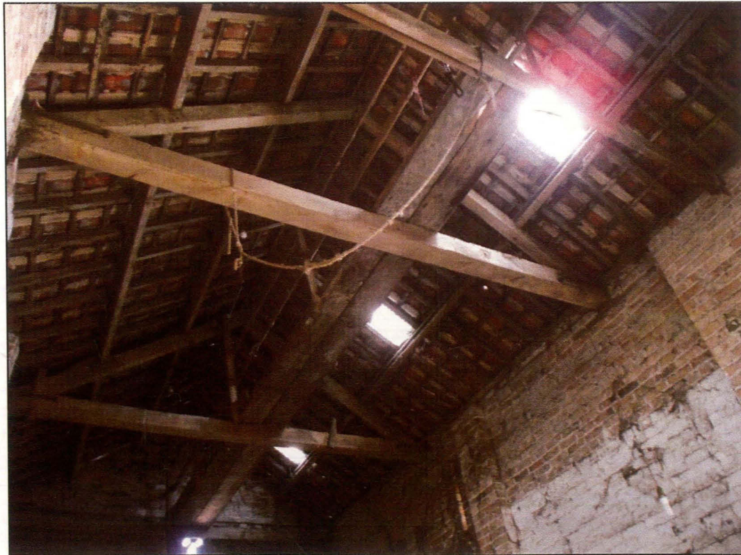
Plate 32 (Shot 54): Roof structure of threshing barn with a view of the roof walkway. Looking east-south-east
