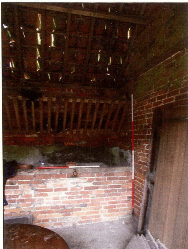
Plate 6 (Shot 14): Brick feeding trough and hay rack within animal shelter A1. Looking north-west
