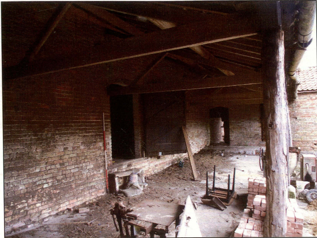
Plate 25 (Shot 38): Lean-to structure and south-south-east elevation of threshing barn B5. Looking north-east
