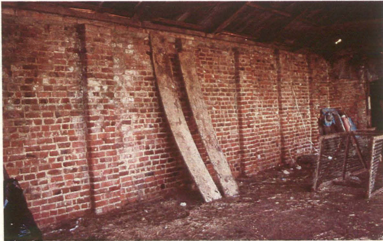
Plate 12 Brick buttresses plinth projecting from western wall of the open barn, looking west
