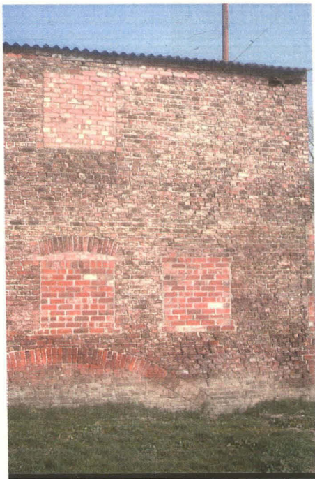
Plate 8 Detail, blocked windows toward eastern end of south side of mill, looking north
