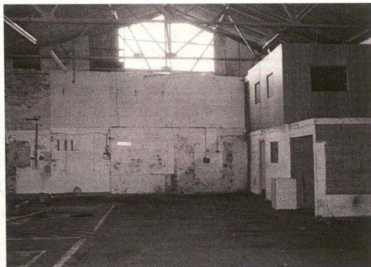
Plate 10 Interior Main Mill Building, west end, showing offices and blocked entries, looking west
