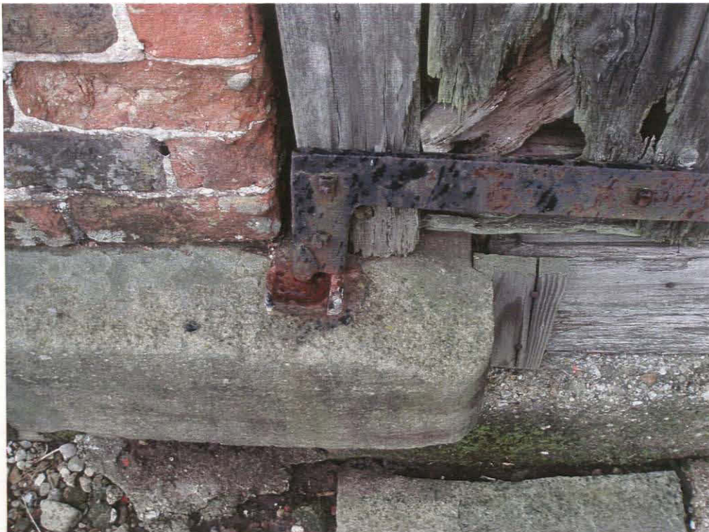
Pl. 12 Barn, east elevation. Detail of double door showing lower hinge and pintle inserted into granite block
