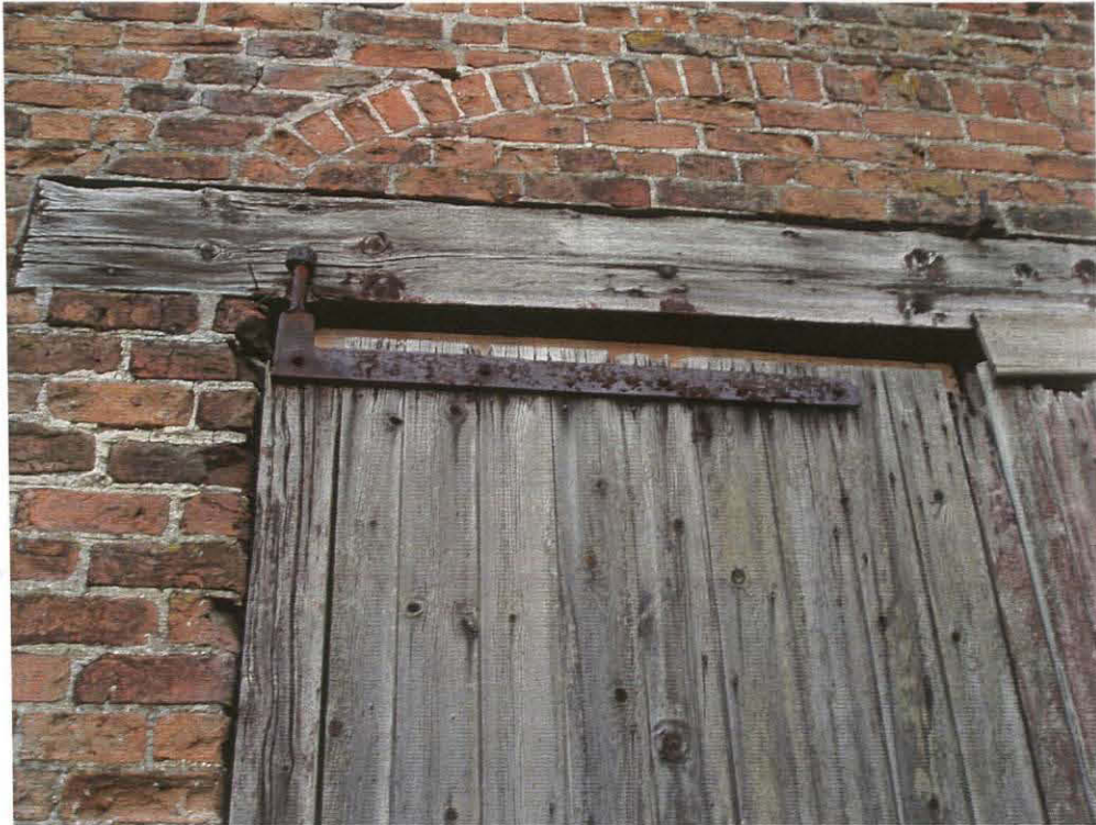
Pl. 11 Barn, east elevation. Detail of double door showing lintel with relieving arch over, and upper hinge and pintle
