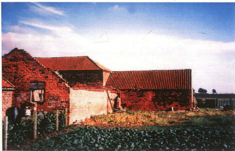
Pl. 6 Derelict stable block on south side of crew yard, looking east to cart shed (Photo, Mr Walker)
