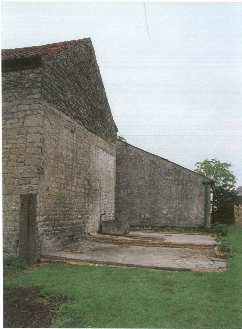
Pl. 41 Building 7. East elevation and base of later outbuilding with stone horse trough. Building 8 (tractor shed) to rear. View north.
