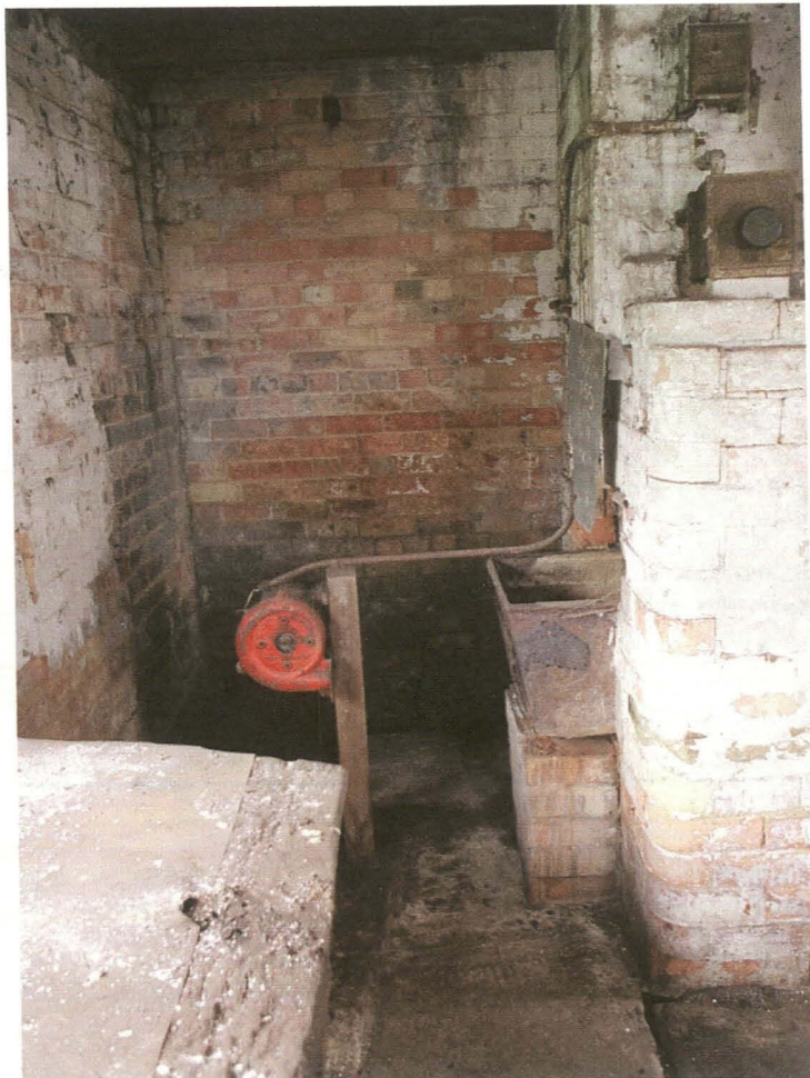
Pl. 14 Electric blower at rear of furnace.
