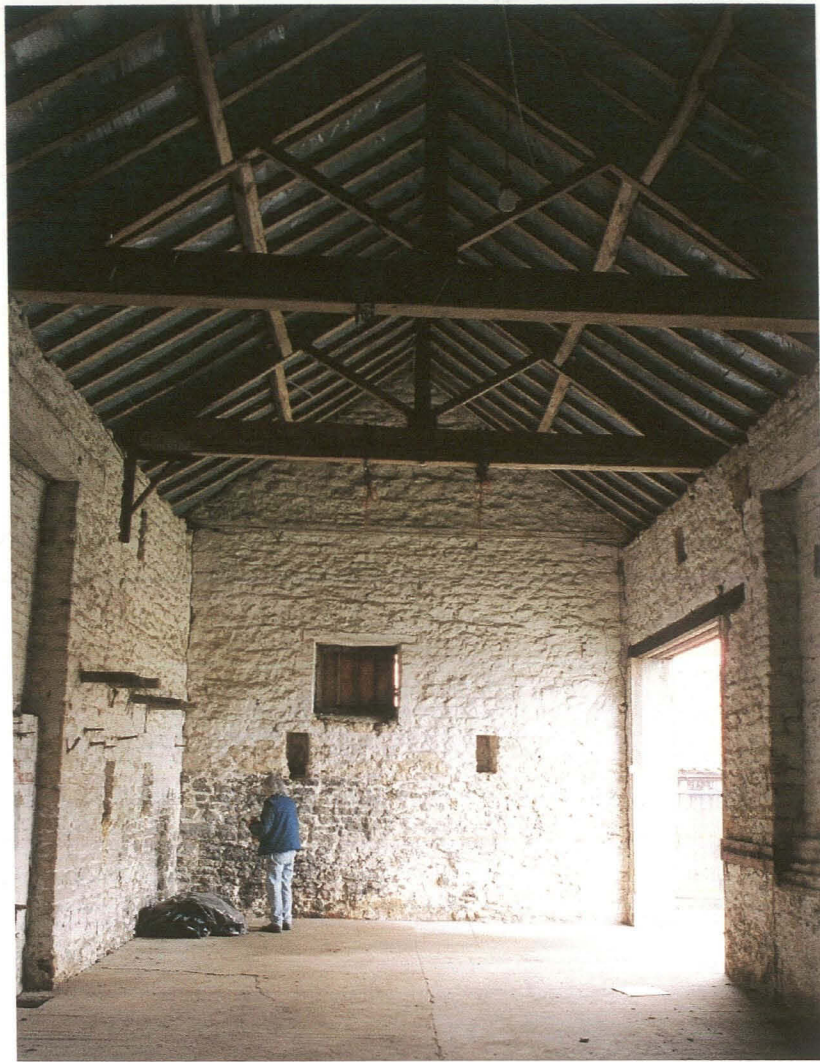
Pl. 45 Building 7 internal view looking west, showing blocked ventilation holes and window, inserted sliding door with blocked opposing doors.
