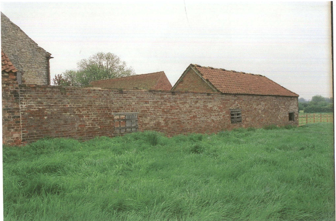
Pl. 19 Buildings 4 and 5. former cow shed Rear (west) elevation, showing ventilation holes at eaves height and three window openings.
