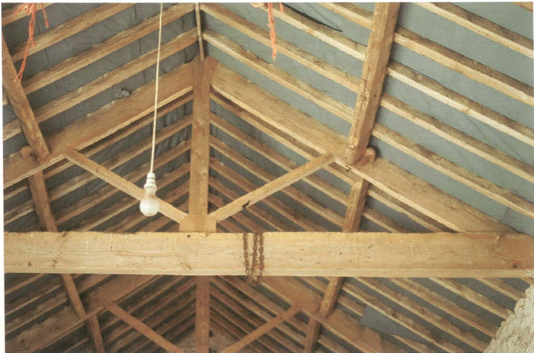
Pl. 46 Building 7. Truss II, showing numbered timbers (II) and pegged staggered purlins. Note chain round the cross timber
