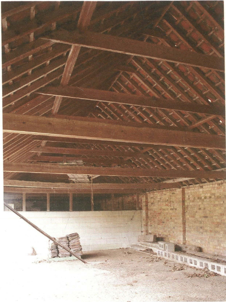
Pl. 7 Building 1 interior, showing internal pilasters on west wall, and roof structure, looking south.
