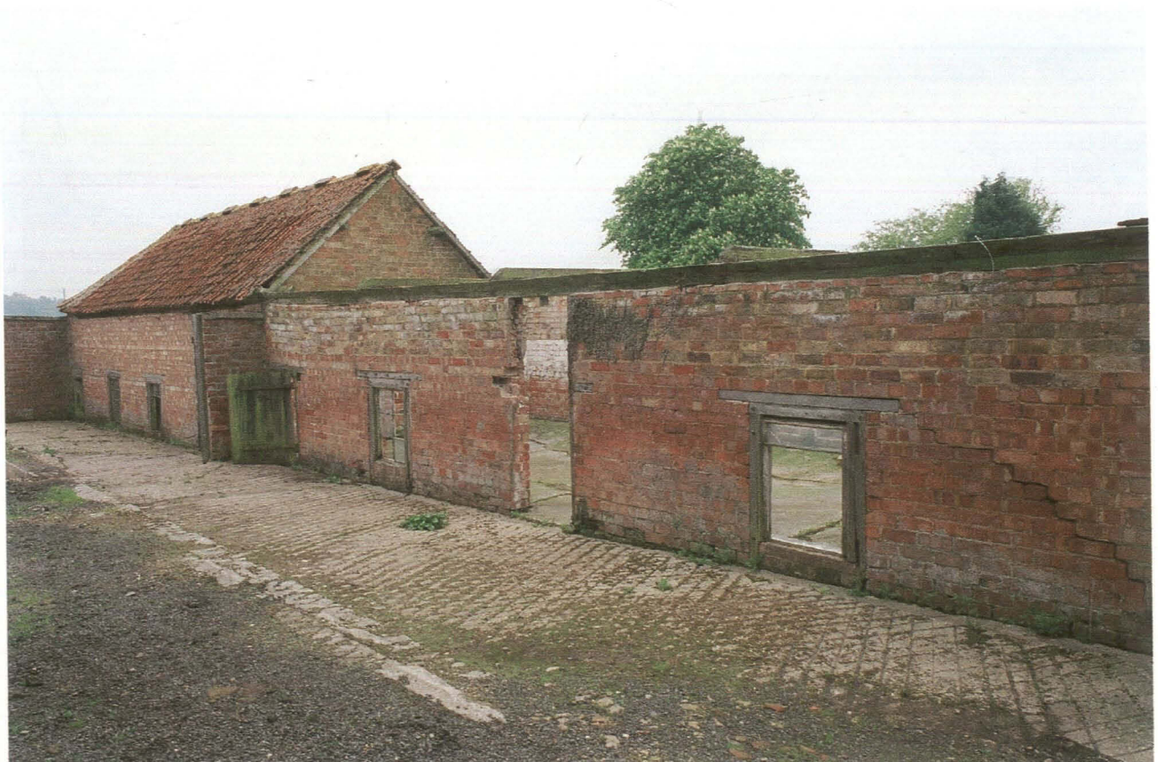
Pl. 20 Buildings 5 and 4. Front (east) elevation showing converted feeding hatches with door in Building 4. Not raised ridge tiles, providing ventilation to the building and concrete surfaces in front of the building.
