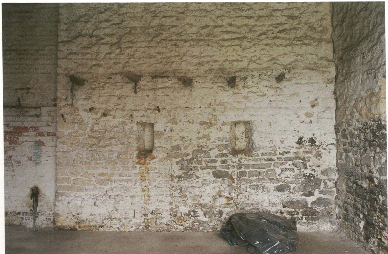
Pl. 44 Building 7. Internal elevation of south wall showing blocked ventilation holes with row of protruding timbers above.
