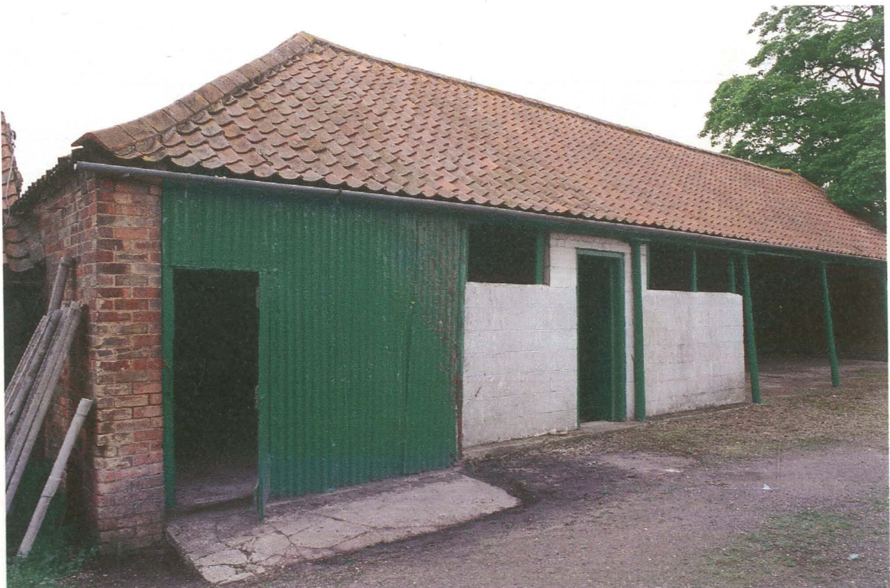
Pl. 10 Building 2 east elevation showing infill of corrugated iron and breeze blocks between the cast iron pillars.
