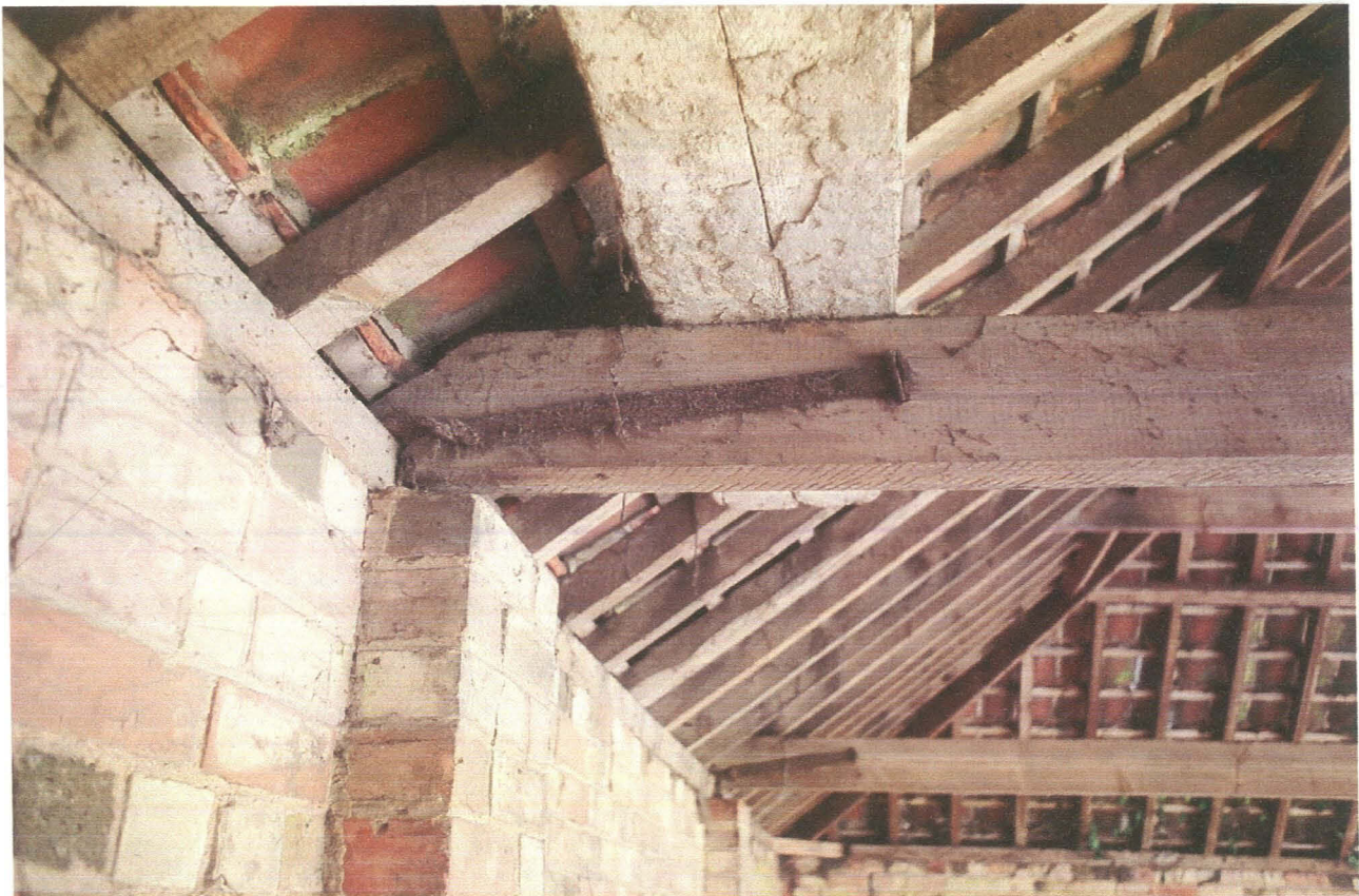
Pl. 9 Building 1 Iron straps secure the trusses to the eaves plate.
