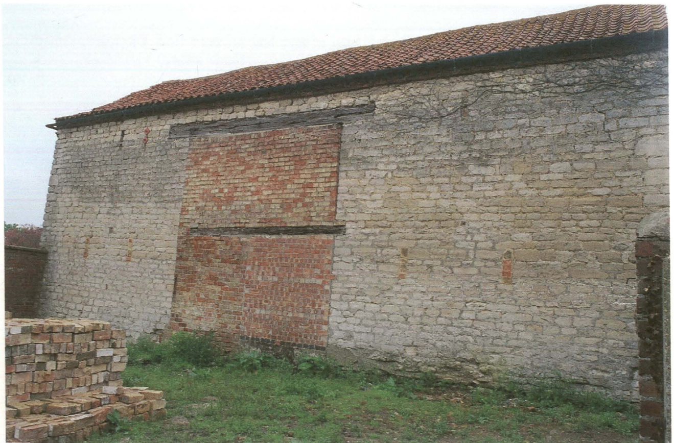
Pl. 40 Building 7. South elevation showing two phases of blocking of the main entrance, and two rows of bricked up ventilation holes.
