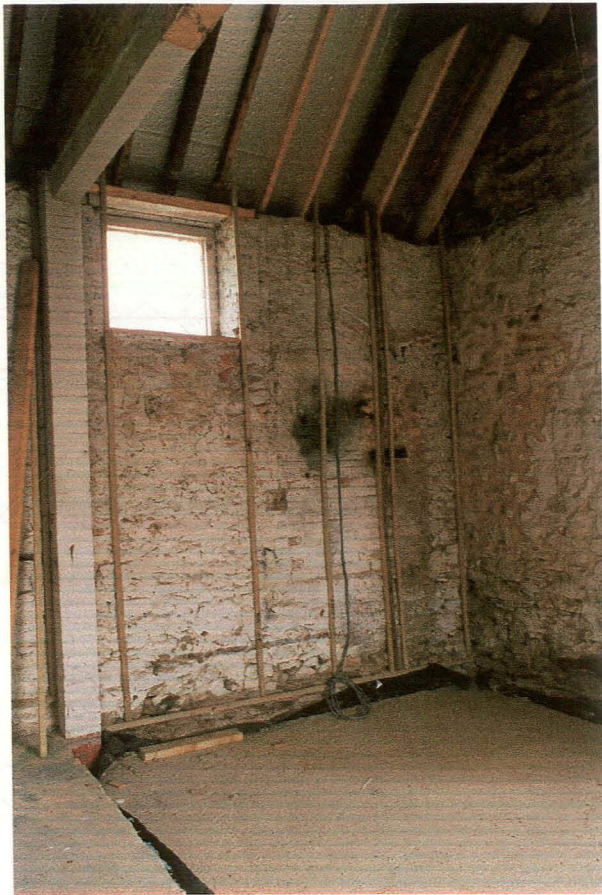
Plate 13: Interior north wall of Barn (2), showing inserted window (left) and blocked window behind pipes (right).
