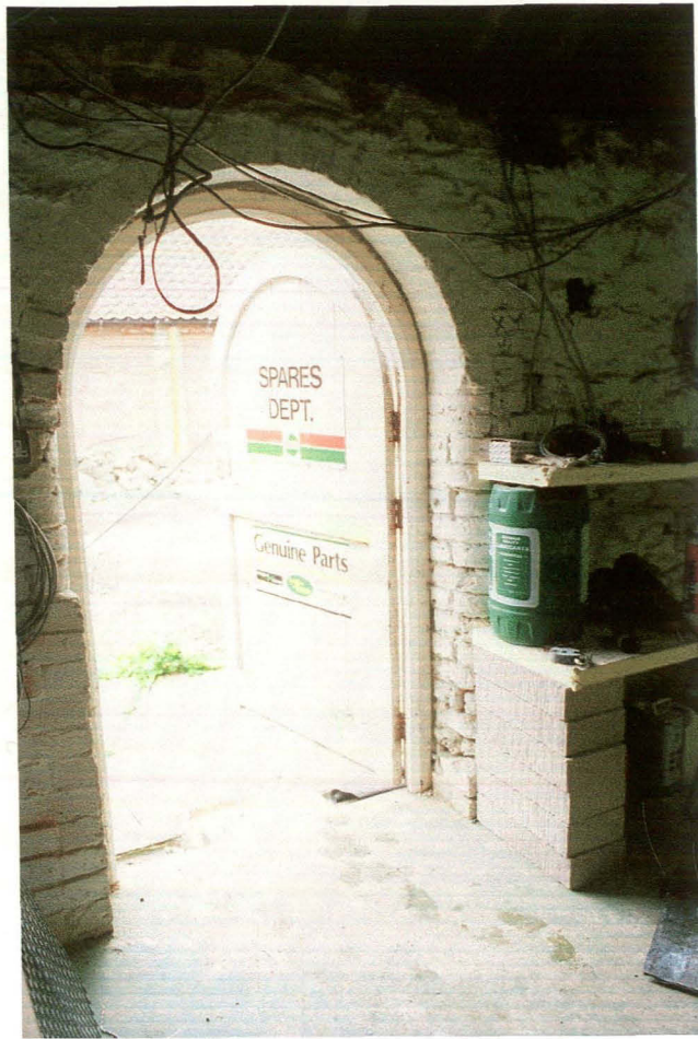
Plate 21: Stable block (4) - entrance in east elevation, showing bullnose brick detail on jambs.
