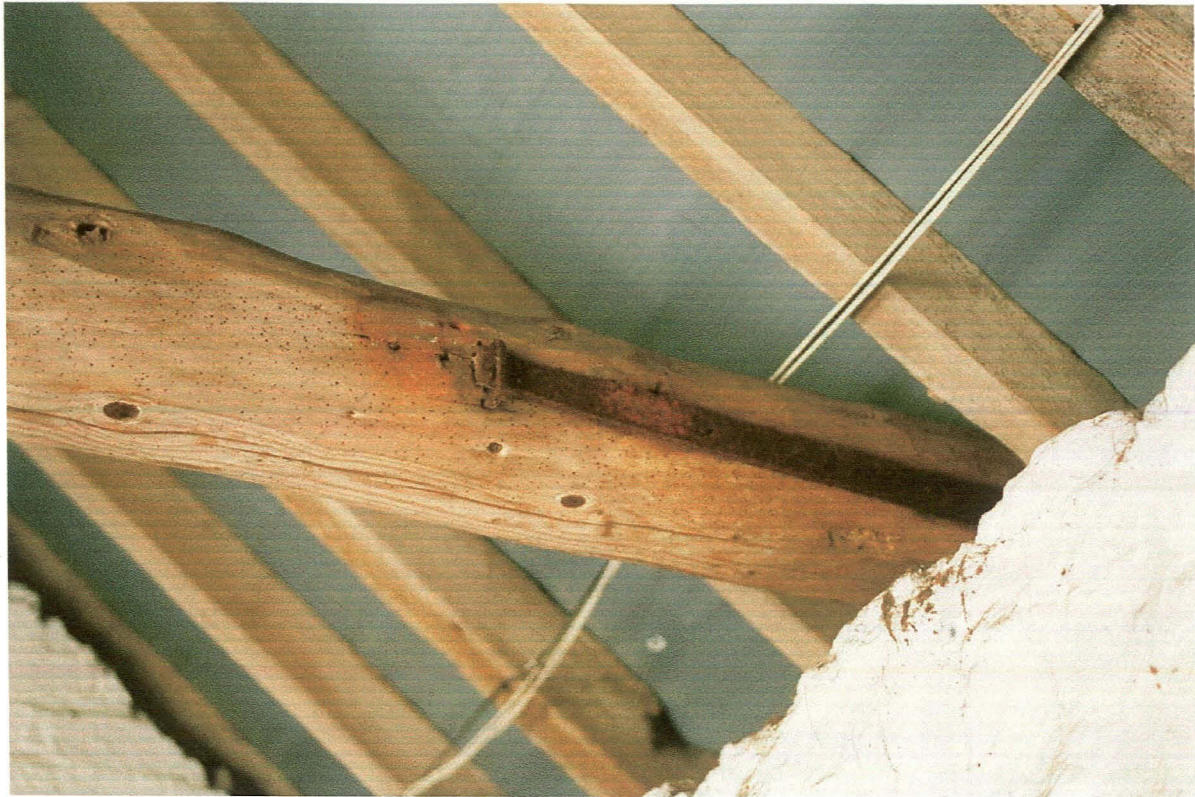
Plate 29: Cattle shed (5) - detail of iron strap used to secure tiebeam to wall.
