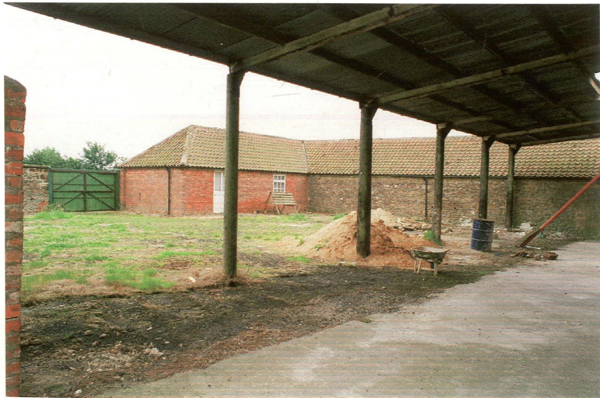
Plate 30: Eastern foldyard looking southwest, showing Store/office (6), and crewyard cross wall incorporated into the east elevation of Cattle shed (5). Dutch barn (7) in foreground.
