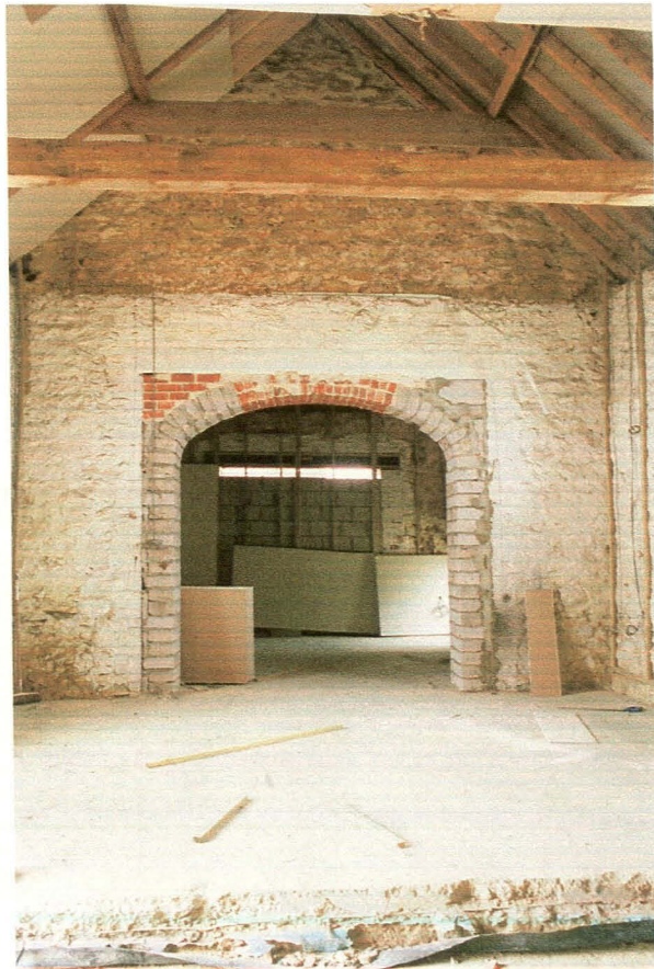
Plate 14: Interior of Barn (1) looking west. Note inserted breezeblock and brick archway inside larger rectangular opening.
