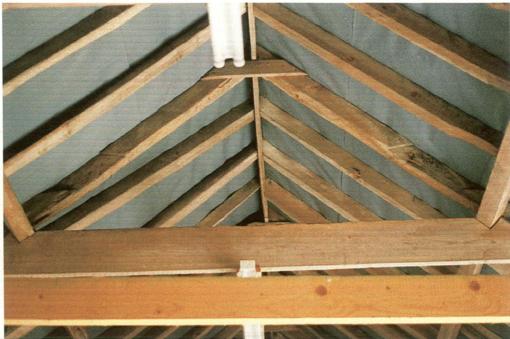
Plate 28: Interior of Cattle shed (5) - detail showing sawn rafters, ridge piece and collar.
