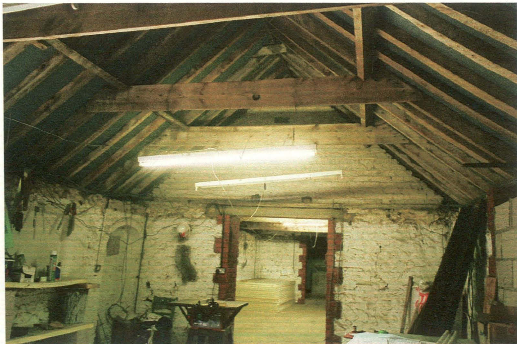
Plate 22: interior of Stable block (4), looking south. Note blocked door in front of cross-wall.
