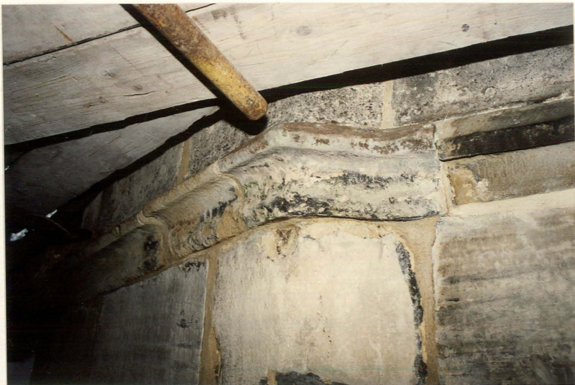
24. X5 wall deviation at string course 583 and block 567 (below).
