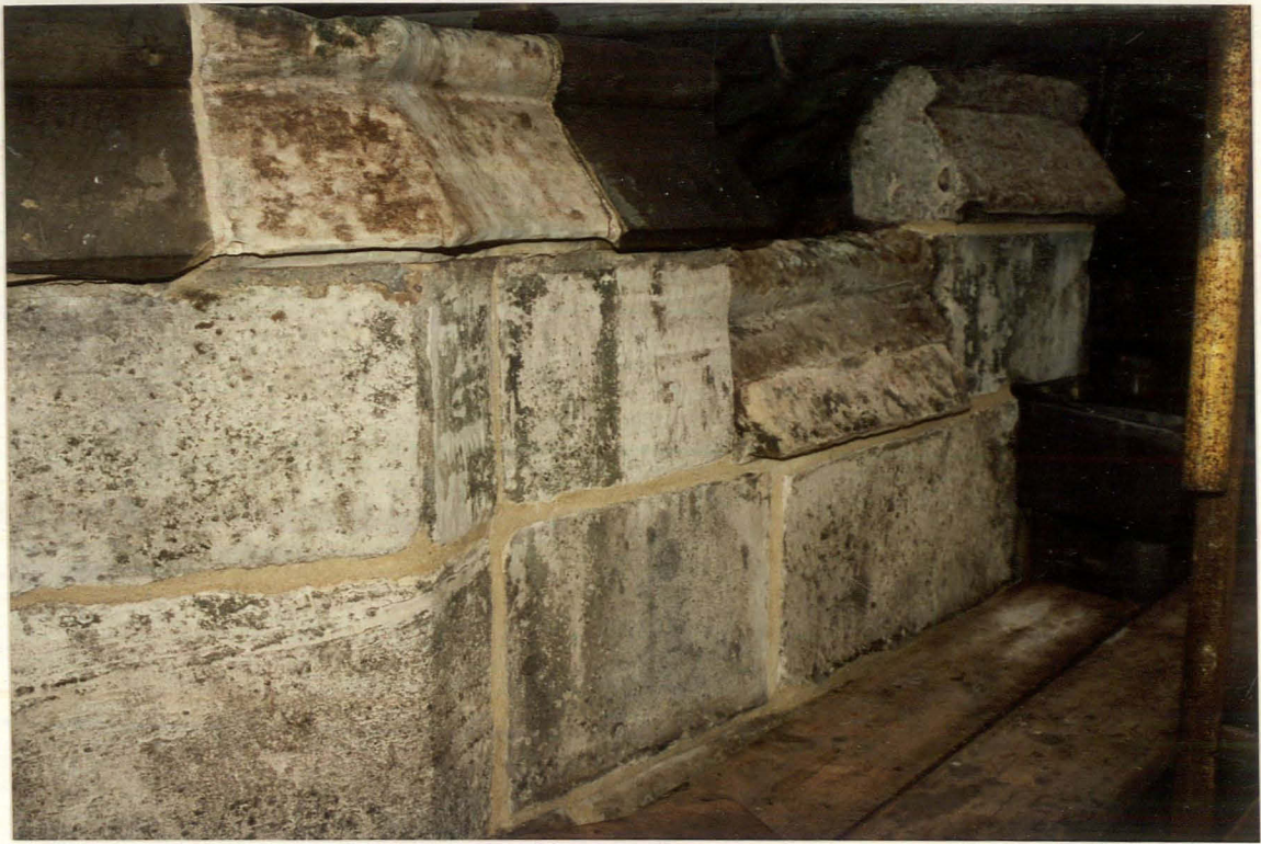
25. X5 wall deviation at parapet, from north-west.
