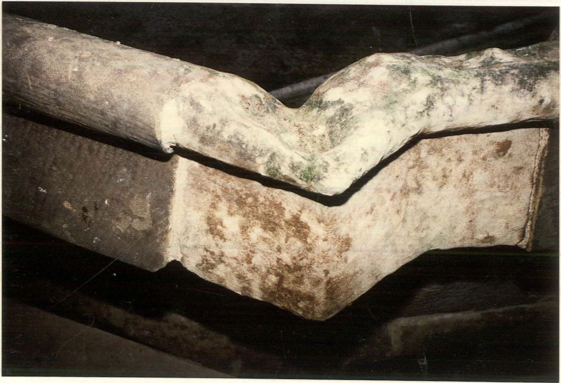
27. X5 wall deviation: parapet cope 632; replacement 632 to left.
