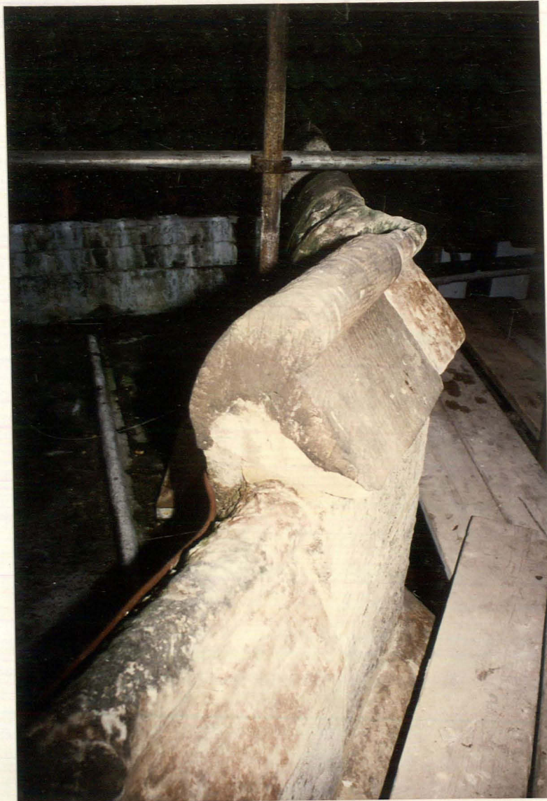
26. X5 wall deviation at parapet coping, from north.
