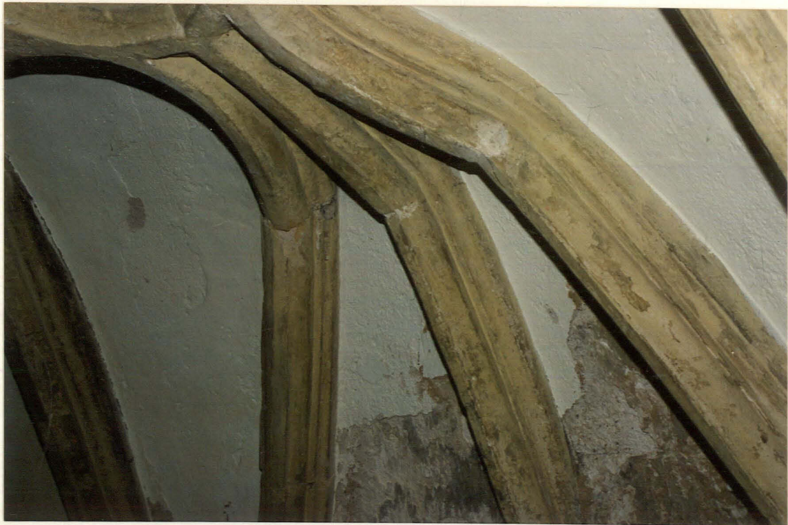
20. Vault, showing distortion at outer junctions.
