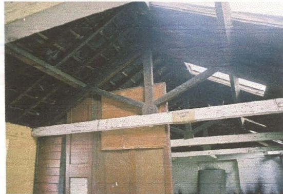
Short King Post roof trusses at the south end of the building
