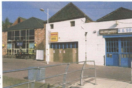
The South elevation - original window openings are evident on the first floor, but the original arrangement of the ground floor has been lost by the insertion of large framed and boarded doors
