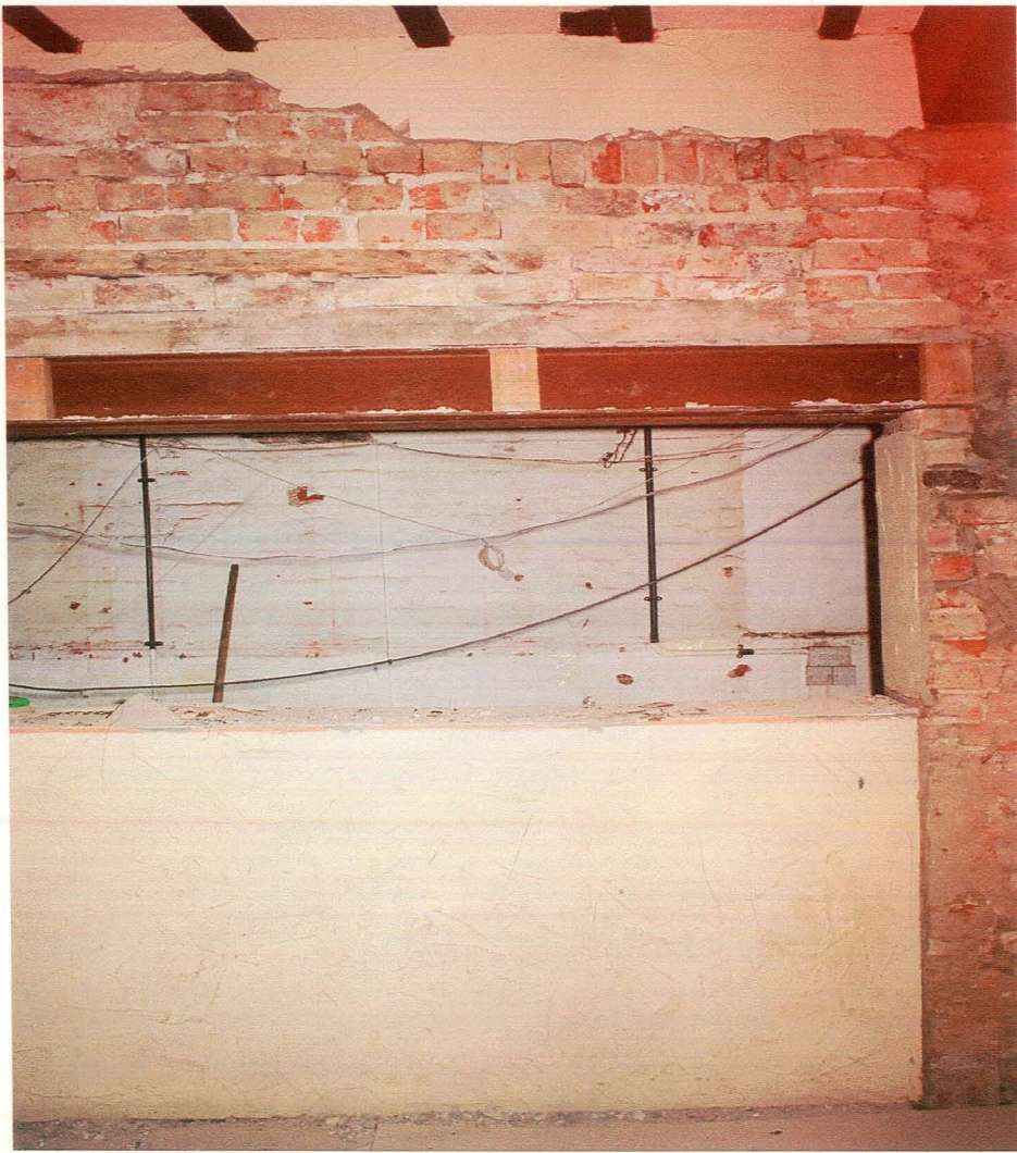
Pl. 7 Detail of vertical joint in brickwork above RSJ.
