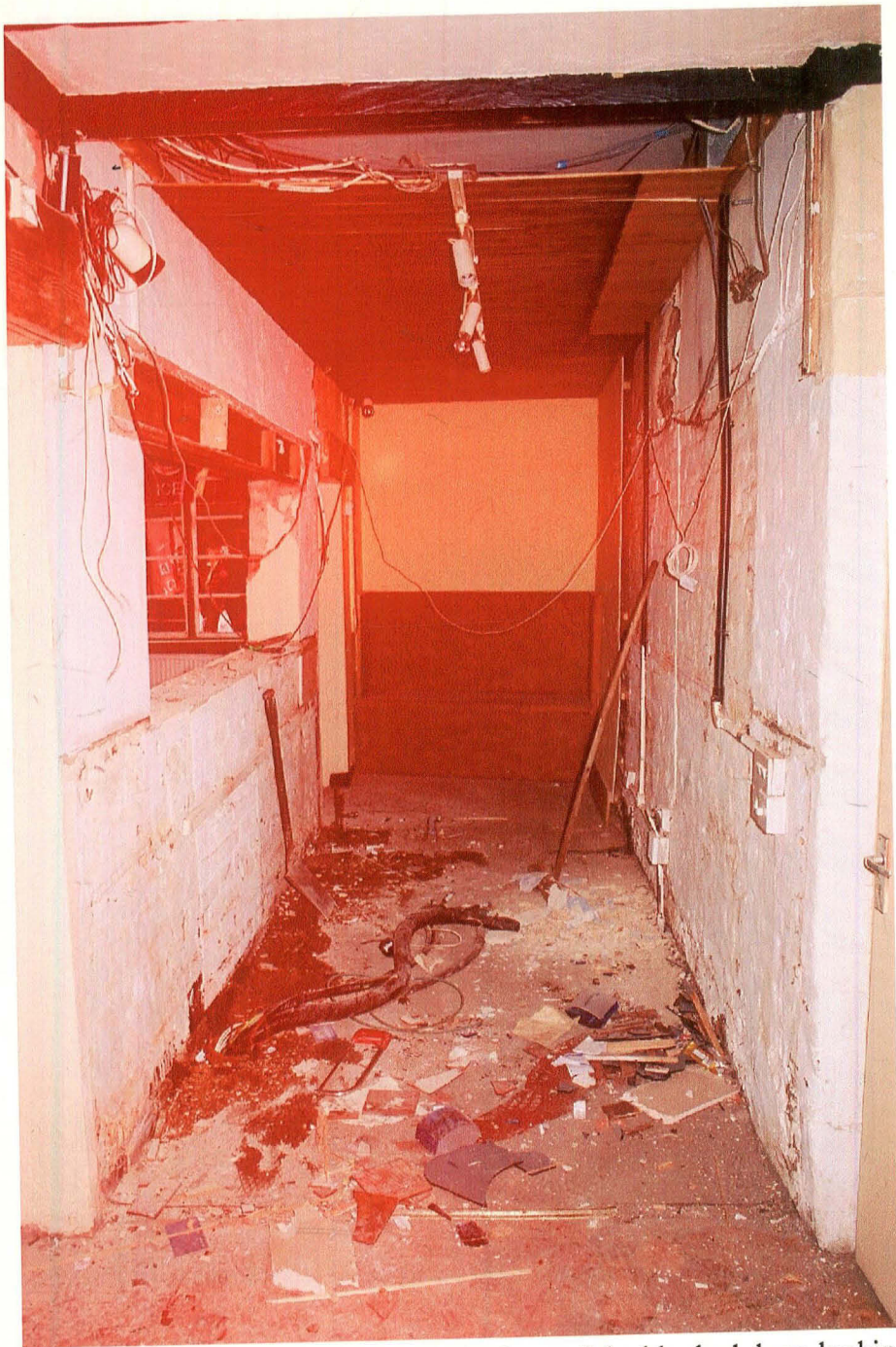
Pl. 3 Passageway showing new seat in front of the blocked door, looking north
