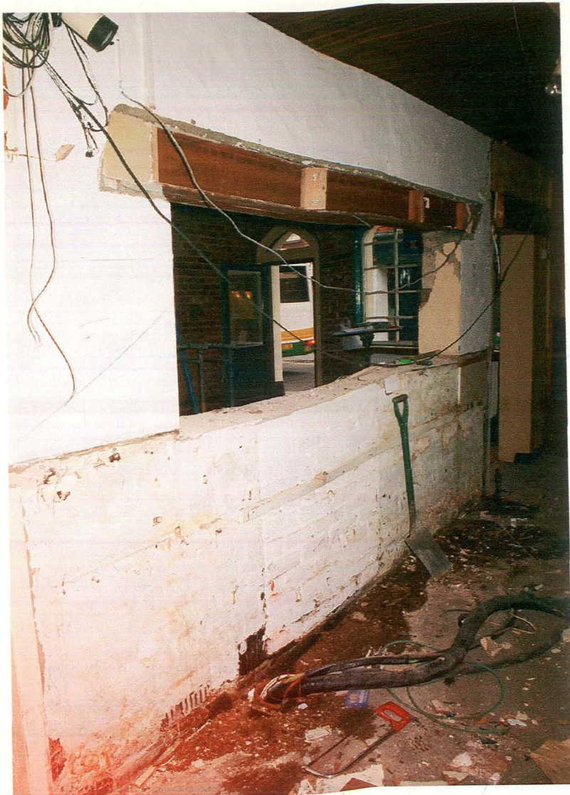
Pl. 5 Passageway, showing inserted bar opening in east wall with blocking beneath (to the left of shovel).
