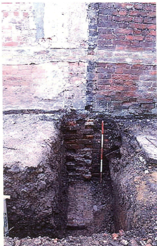
Pl. 2 Re-used foundation (012). The other re-used foundation (013) is visible behind the scale. Looking south.
