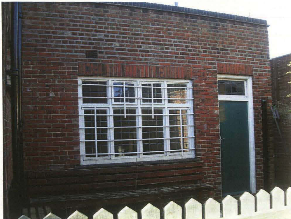
Pl. 14 West elevation of single storey block showing access to the pool room Note added parapet marked by change in mortar colour.
