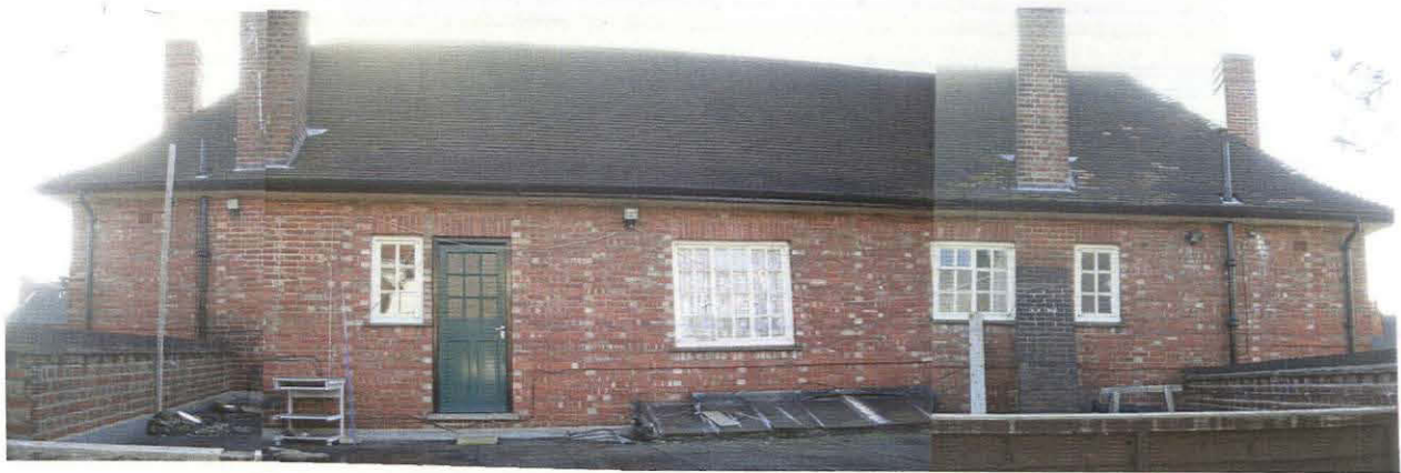
Pl. 15 North elevation showing inserted access to flat roof and chimney between the bathroom and toilet windows that serves the landlord's living room .
