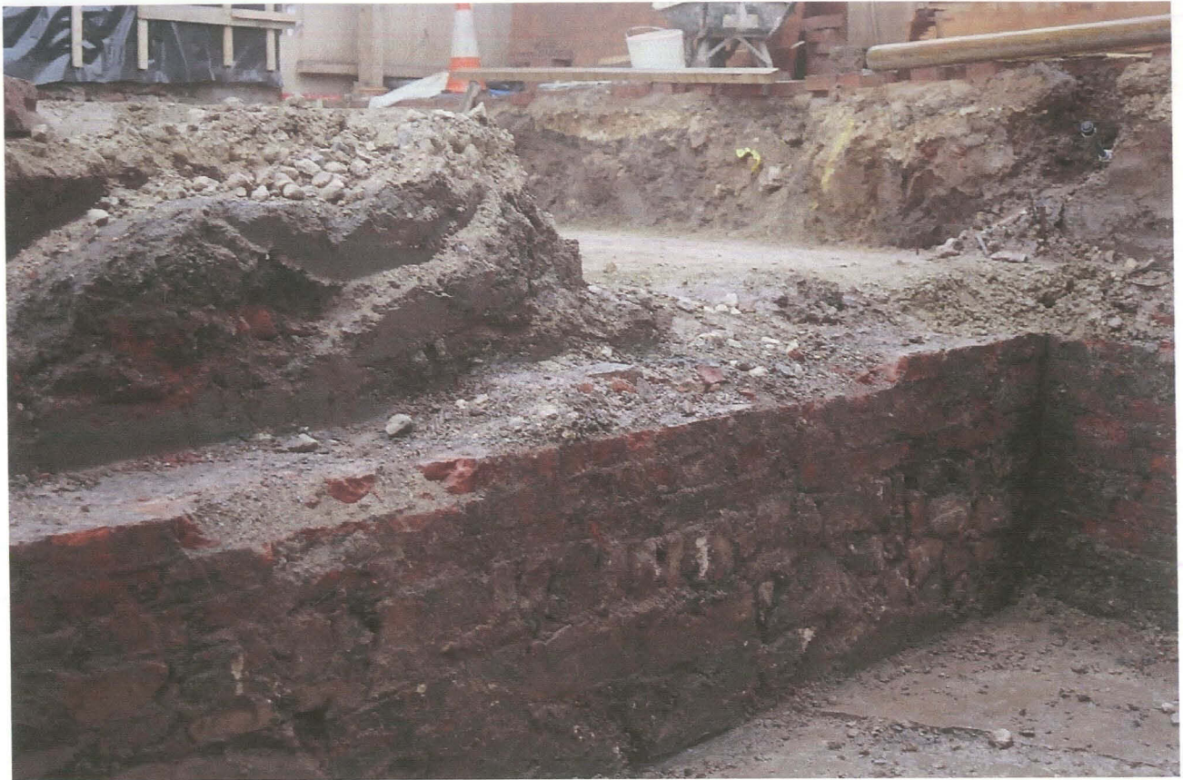
PI. 43 Brick and stone rubble cellar wall, No. 11 Market Street (looking north-west).
