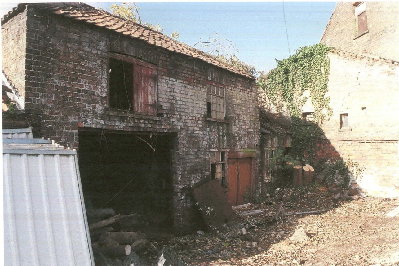
PI. 3 East elevation of Buildings 2 (left) and 1, with gable end of Building 4.
