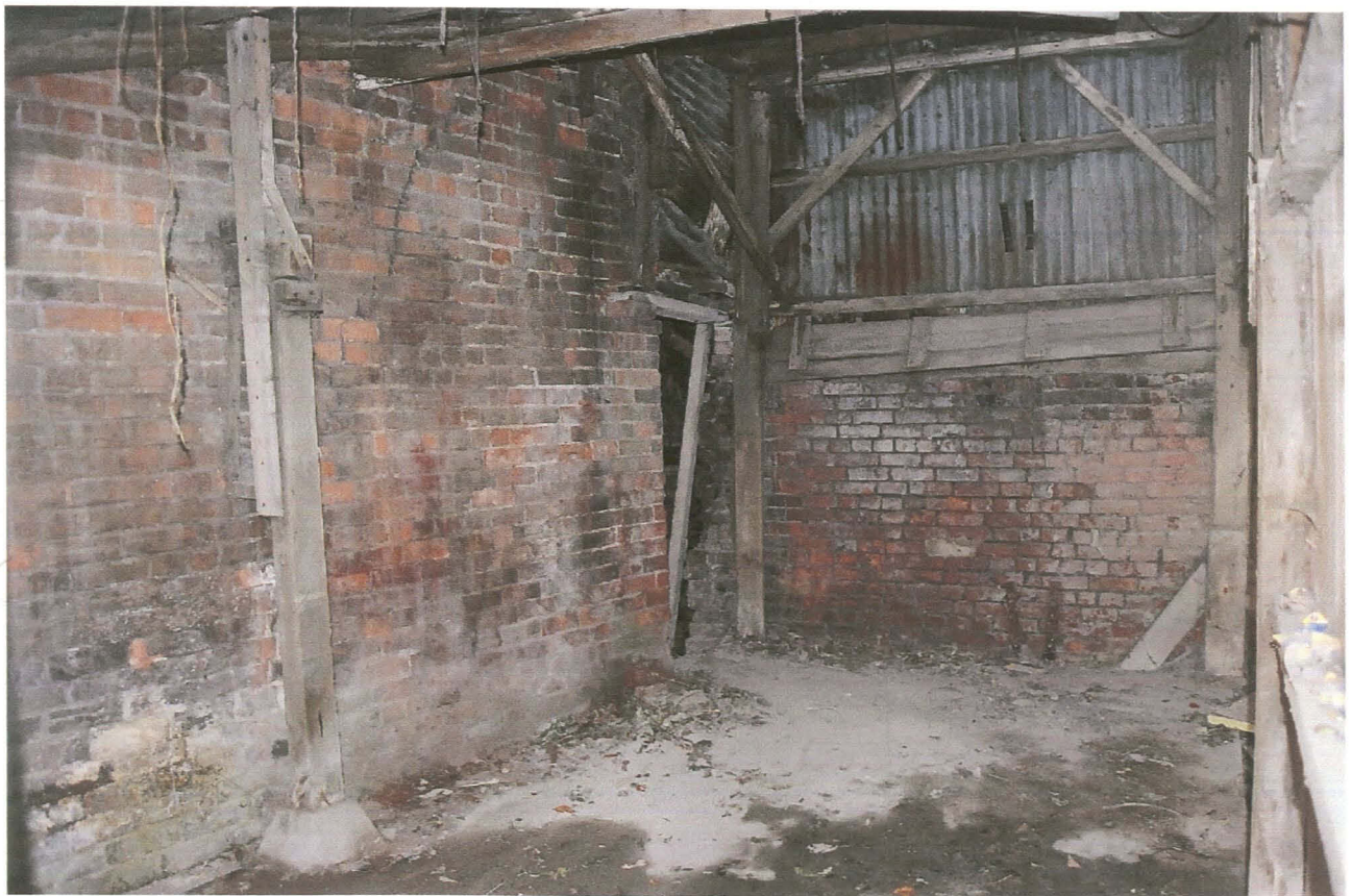
PI. 16 Inserted entrance in south-east corner of Building 5 giving access to Building 1.
