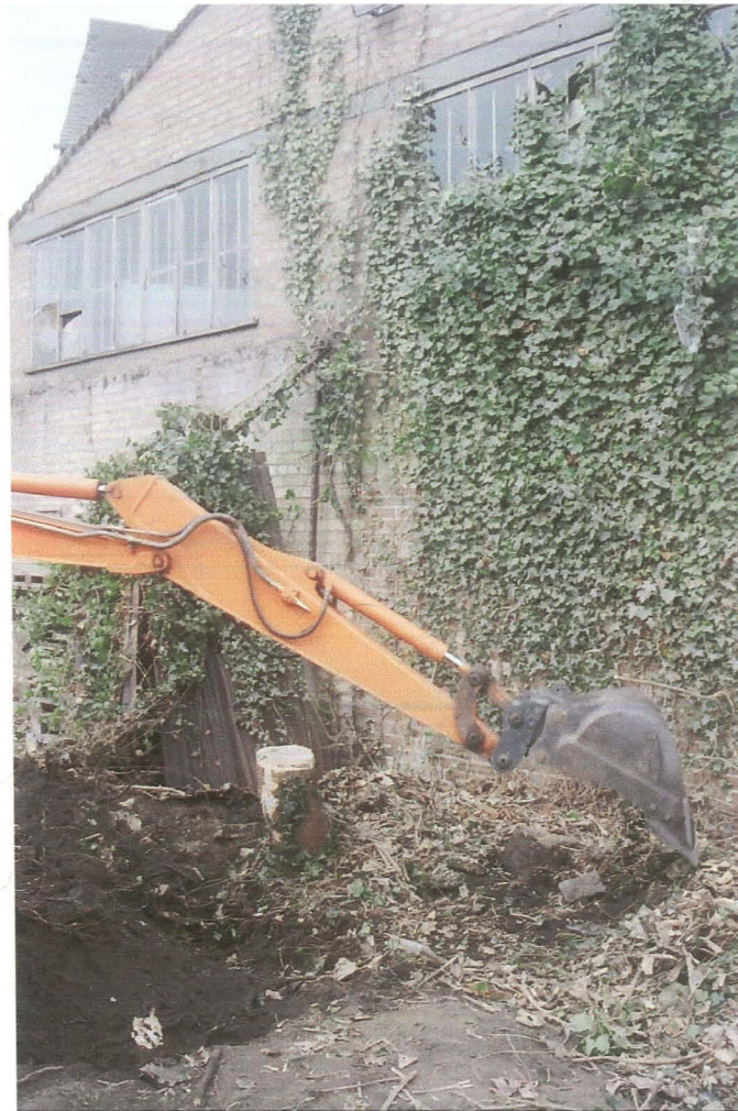
PI. 53 Location of buried wall foundation, behind No. 7 Market Street (looking north-west).
