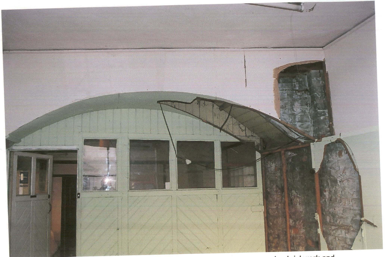
PI. 35 Building 11. Ground floor, east room, after removal of cladding, exposing brickwork and base of first floor fireplace.
