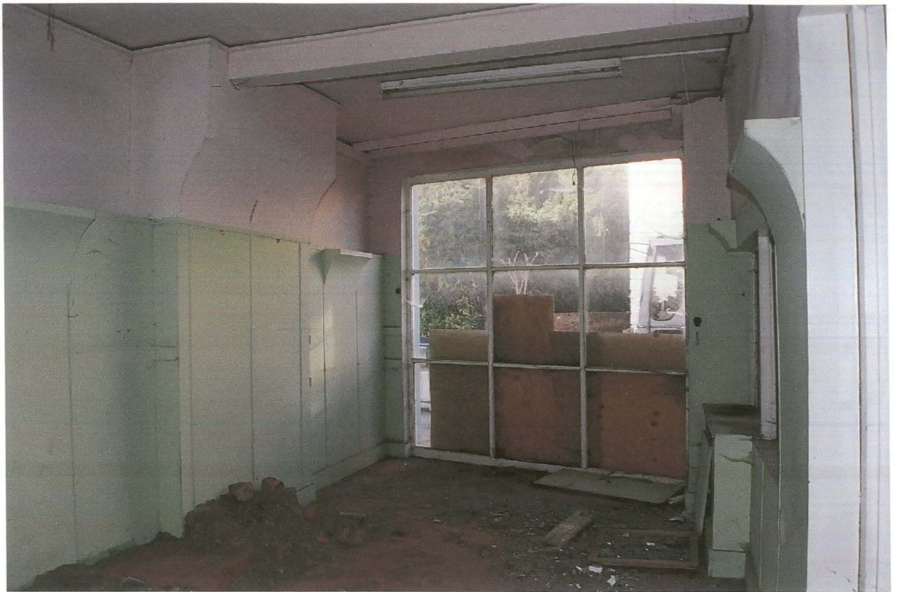
PI. 33 Building 11. Ground floor, east room, showing inserted window in north wall. Looking north.
