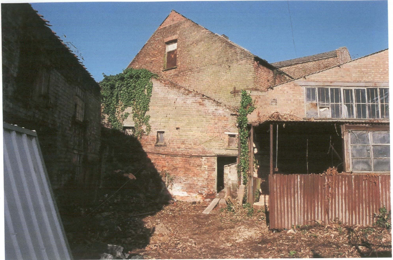
PI. 9. Building 4, with gable end of Corn Exchange to rear, looking north.
