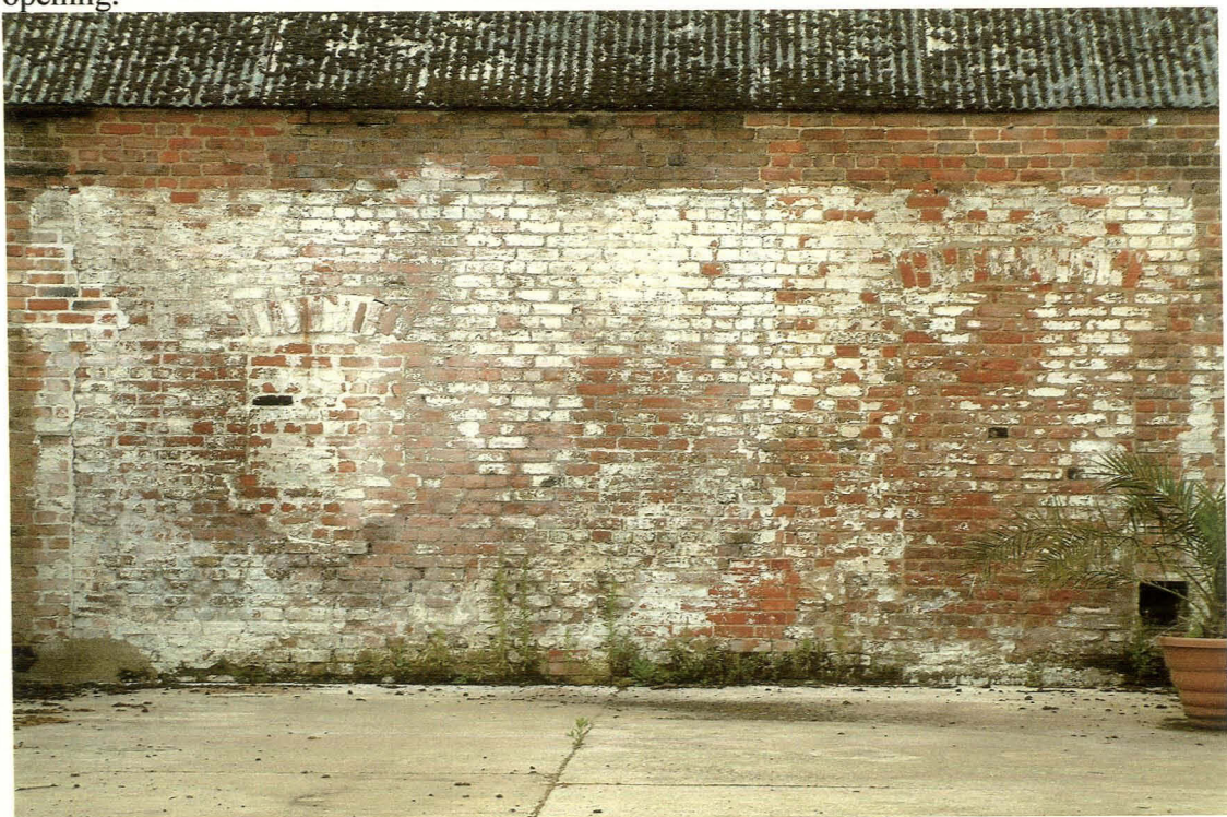
Plate 16. The western face looking onto the courtyard showing two bricked up openings, a doorway and a window.
