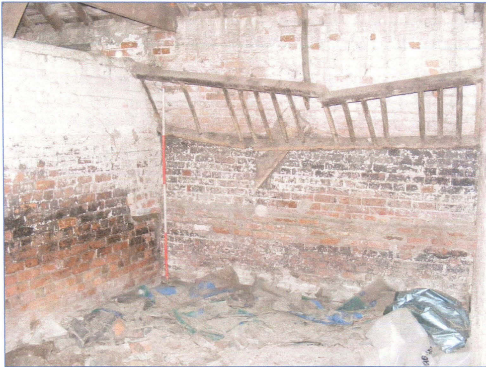
Plate 10 (Shot 33): Interior of Room A3, looking north-west from the doorway to Room A4. There is a wooden hay rick on the north wall, with a scar below indicating a former feeding trough. A curved recess on the western partition wall, immediately to the left of the scale as indicates the presence of the former trough.
