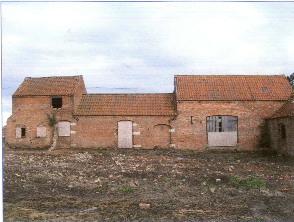
Plate 5 (Shot 11): South elevation of Block A, looking west-north-west. The roof scar of the former western range is visible to the left of the shot. Note the position of the pitching hole directly above the demolished structures
