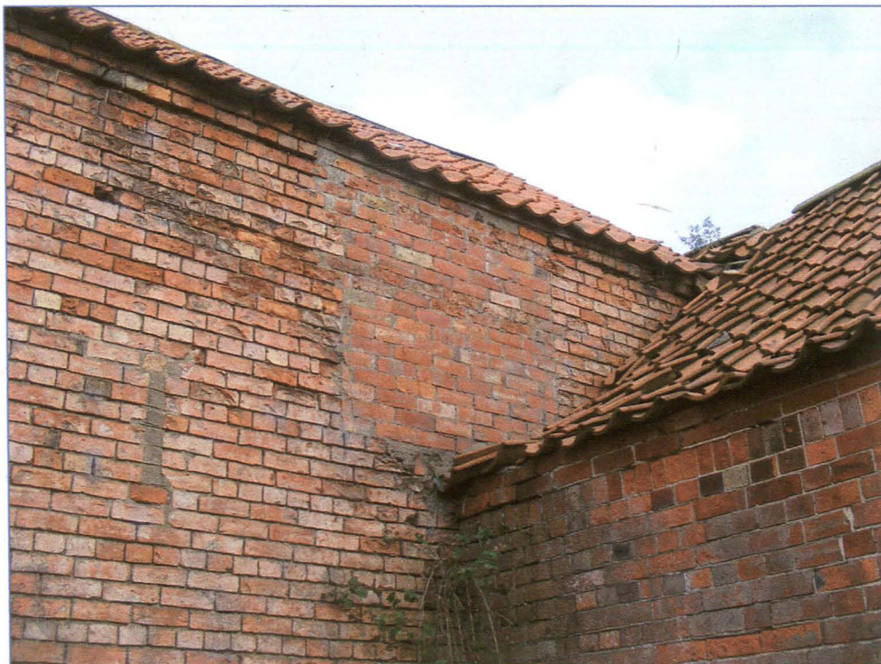
Plate 12 (Shot 20): Blocked pitching hole in the south elevation of the threshing barn. It seems likely that it was blocked during the construction of the adjacent Block B. This shot also shows a possible roof scar for a former covered yard.
