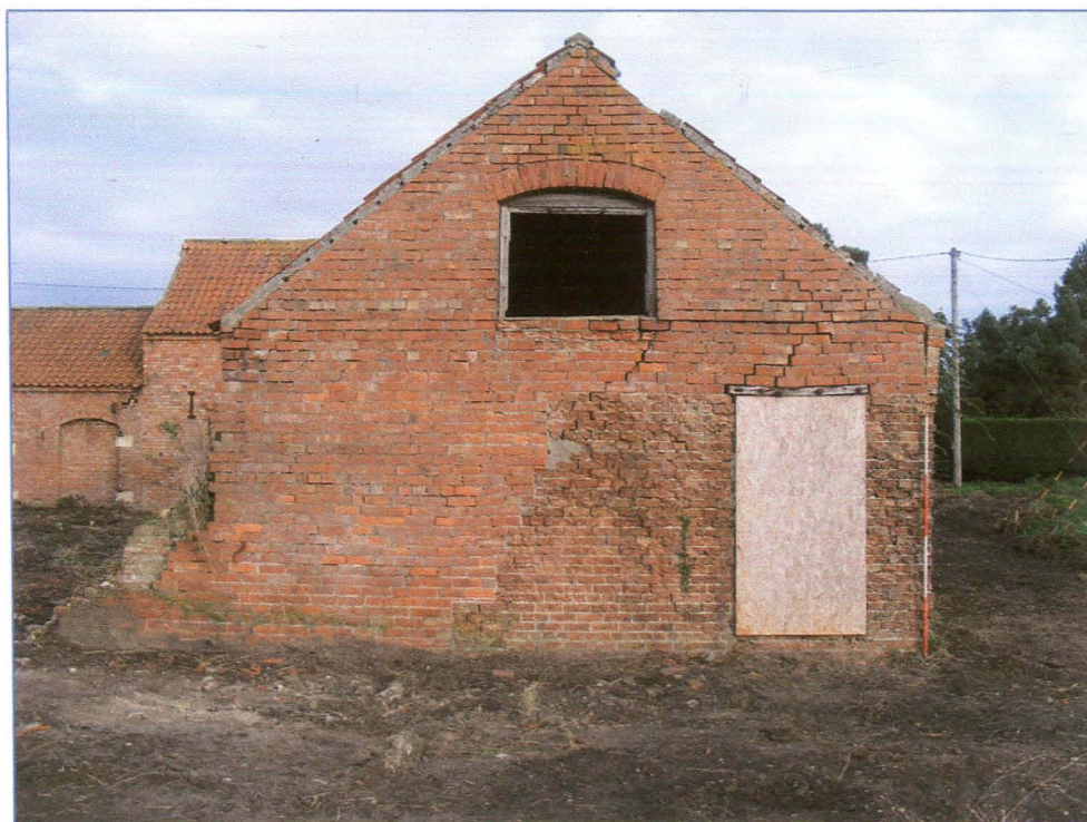
Plate 18 (Shot 9): South elevation of Block B, showing the pitching hole and the area of repair around the doorway. Note the area of collapse above the door.
