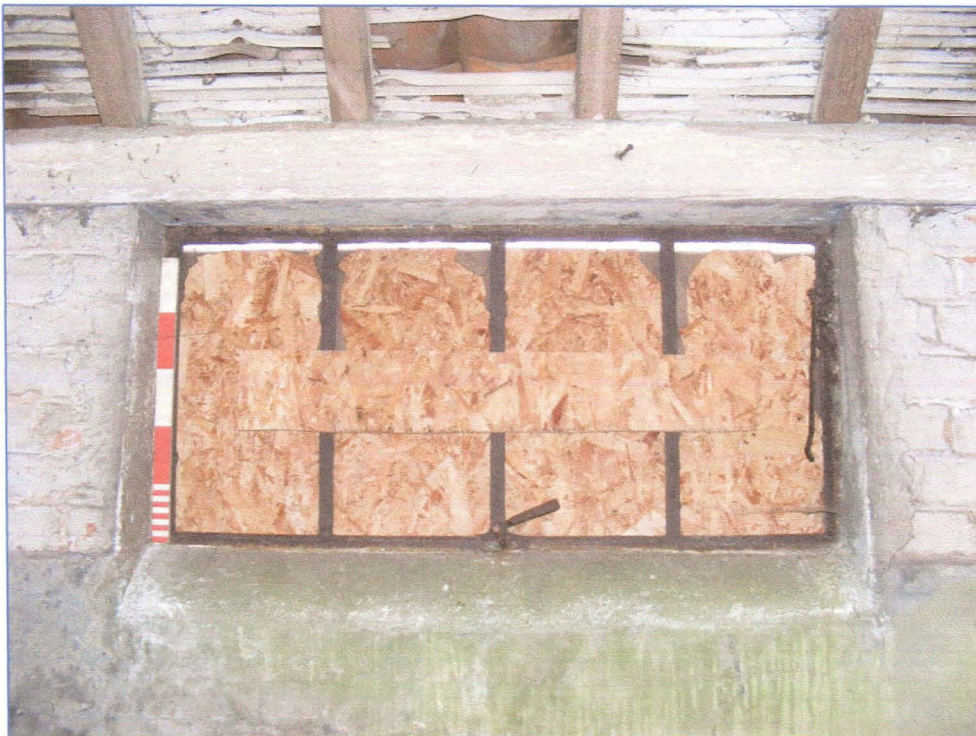
Plate 20 (Shot 48): Internal view of window in east elevation of Room B1, looking east-north-east
