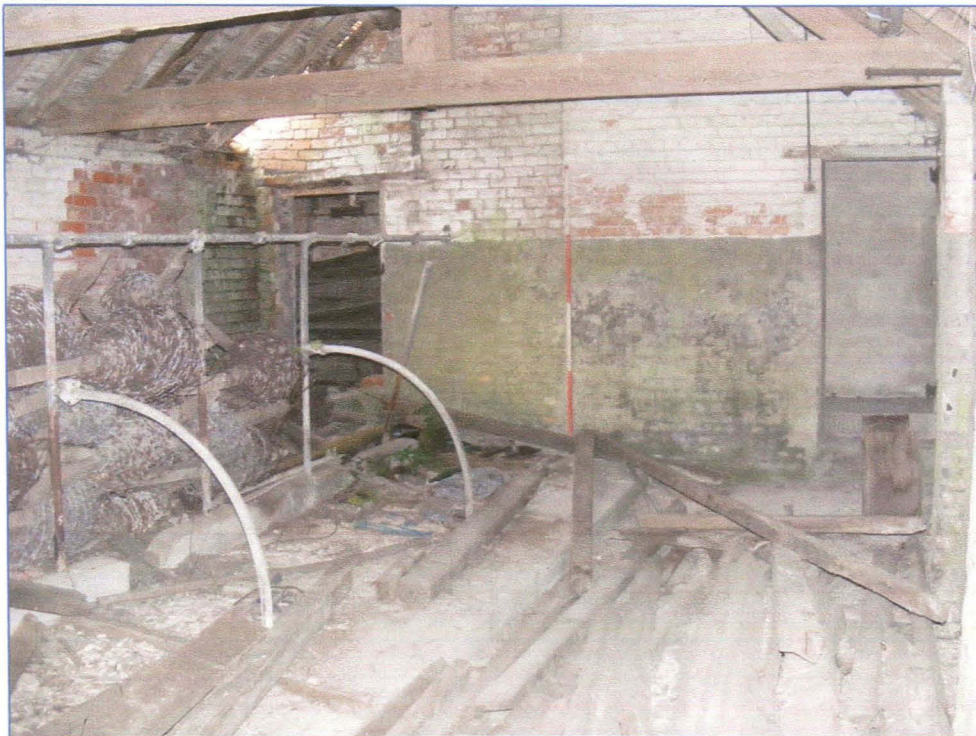
Plate 22 (Shot 27): Interior of Room B1, looking north-north-west from the eastern doorway into B2, showing the steel frame of the milking stalls to the left of shot and the concrete platform. At the far end of the room, adjacent to the scale can be seen the abutting walls of the threshing barn to the west and outbuilding B3 to the east.
