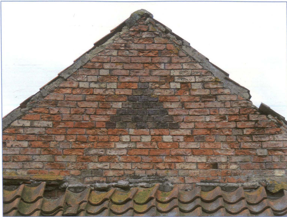
Plate 13 (Shot 47): Brick detailing below apex of east elevation of Block A, looking west-south-west
