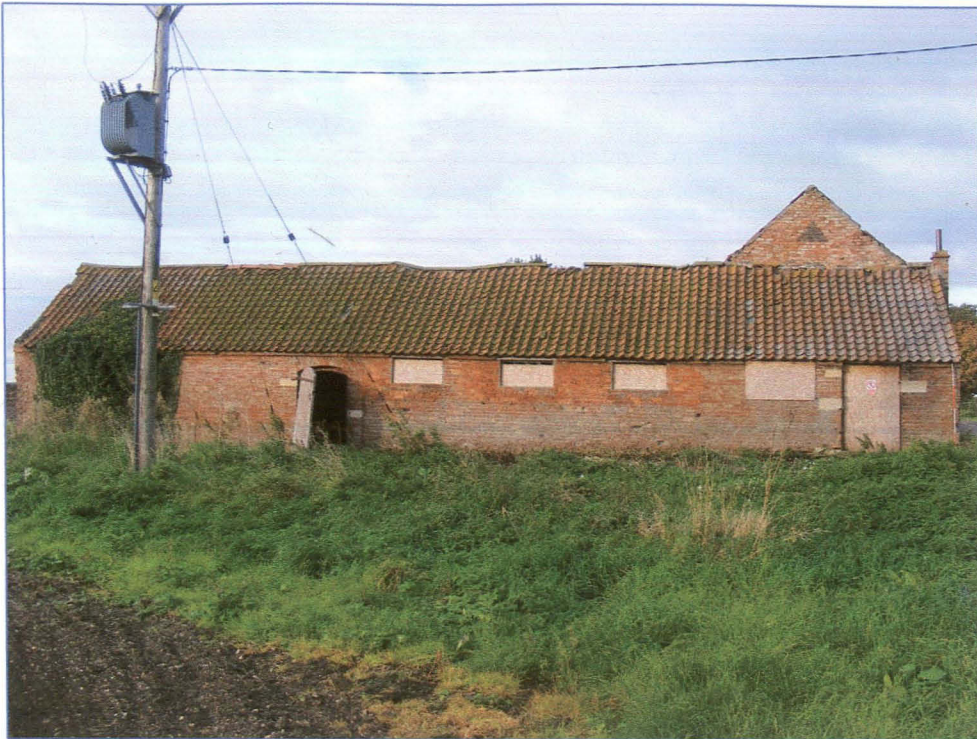
Plate 19 (Shot 8): East elevation of Block B, looking west-south-west. The area of brick rebuilding around the three identical windows in Room B2 suggests a single phase of redevelopment
