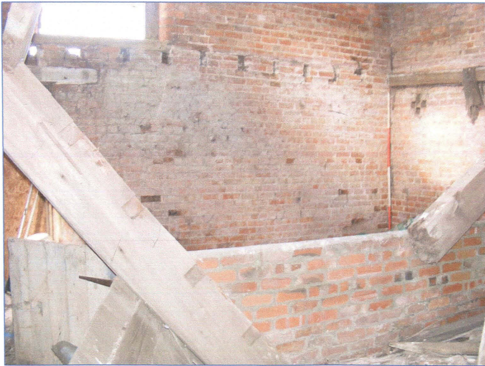
Plate 8 (Shot 36): Interior of Room A1, looking north-west from the doorway to Room A2.
