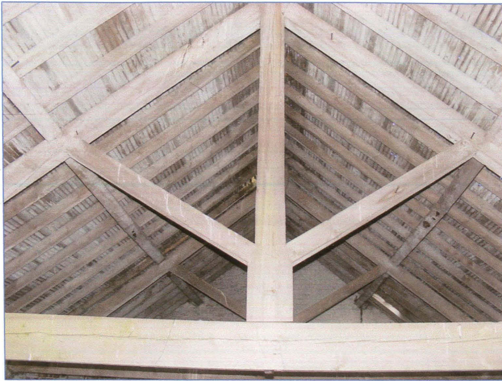
Plate 21 (Shot 26): Roof structure of Rooms B1 and B2, looking north-north-east from the south end of B2
