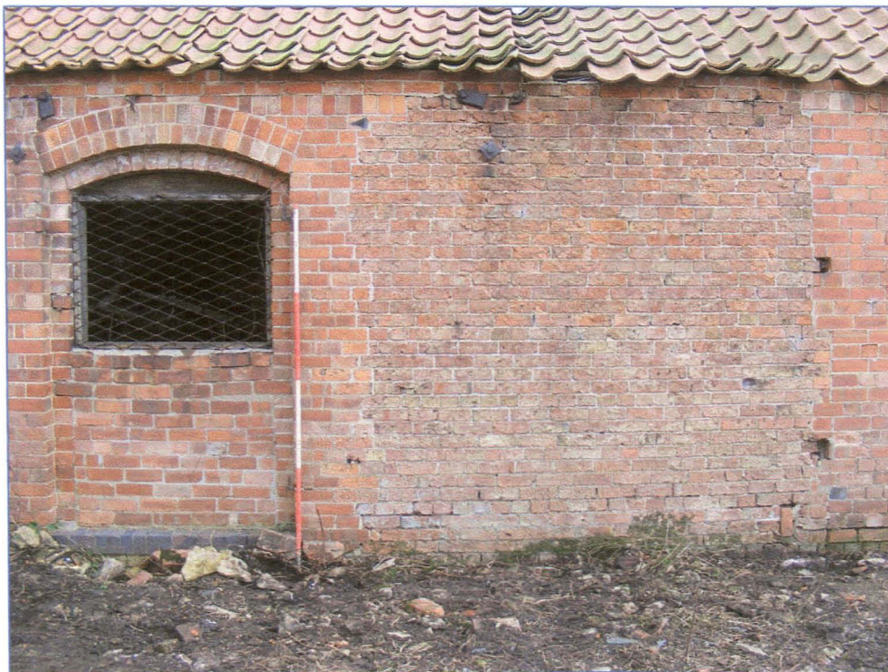
Plate 16 (Shot 19): Detail of repair to brickwork and blocked doorway in west elevation of Block B. Looking east-north-east
