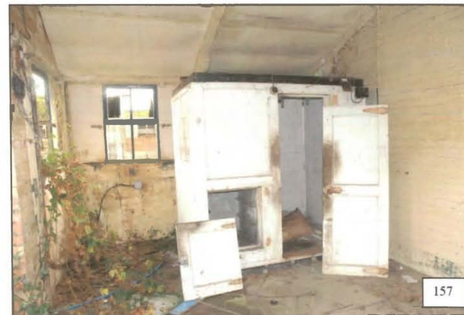
In the eastern part of the hut, the eastern two bays were divided from the central section and contained a large refrigerator, which may have been an original fixture. A central opening in the partition wall gave access to the central three bays of the building.
