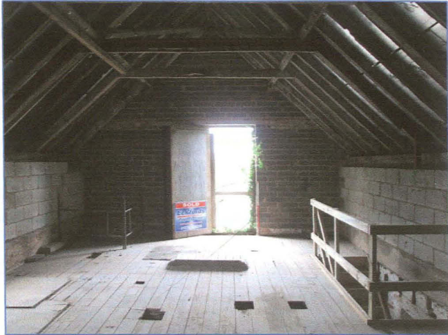
Plate 13: North end of the second floor, looking north to the door and repaired north wall.
