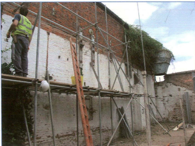
Plate 6: East elevation, looking north-north-west. Note the small chimney and the metal funnel at the north end of the elevation.
