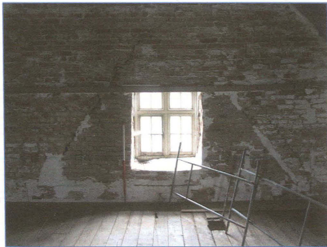
Plate 14: Window at the south end of the second floor, showing the cracks evidencing the subsidence of the south wall. Looking south.
