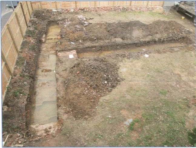
Plate 1: The evaluation trenches, looking north from the second floor of the cornmill.
