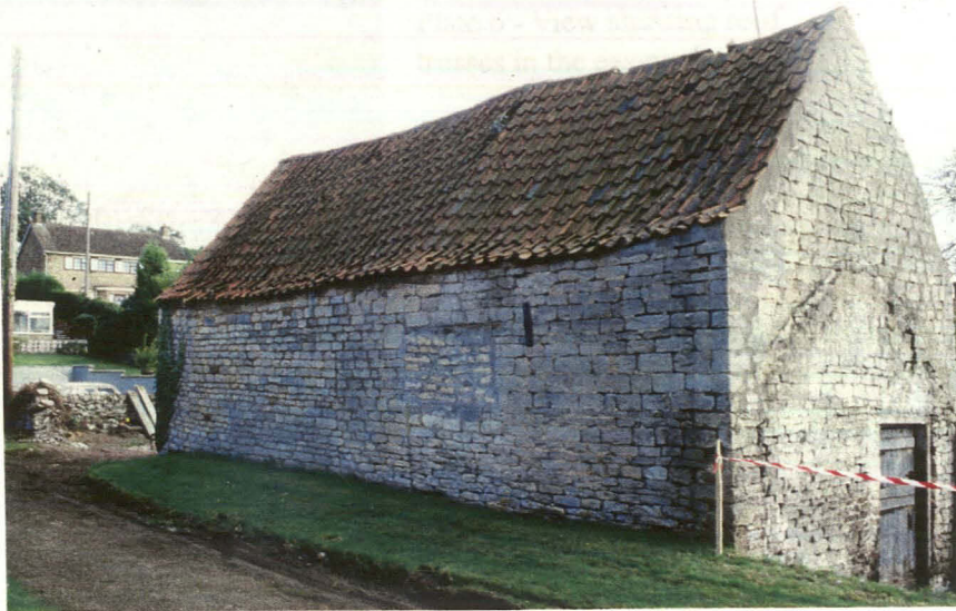
Plate 4 - View showing the barns from the northwest, showing the join between the two and the scar outline of a further outhouse
