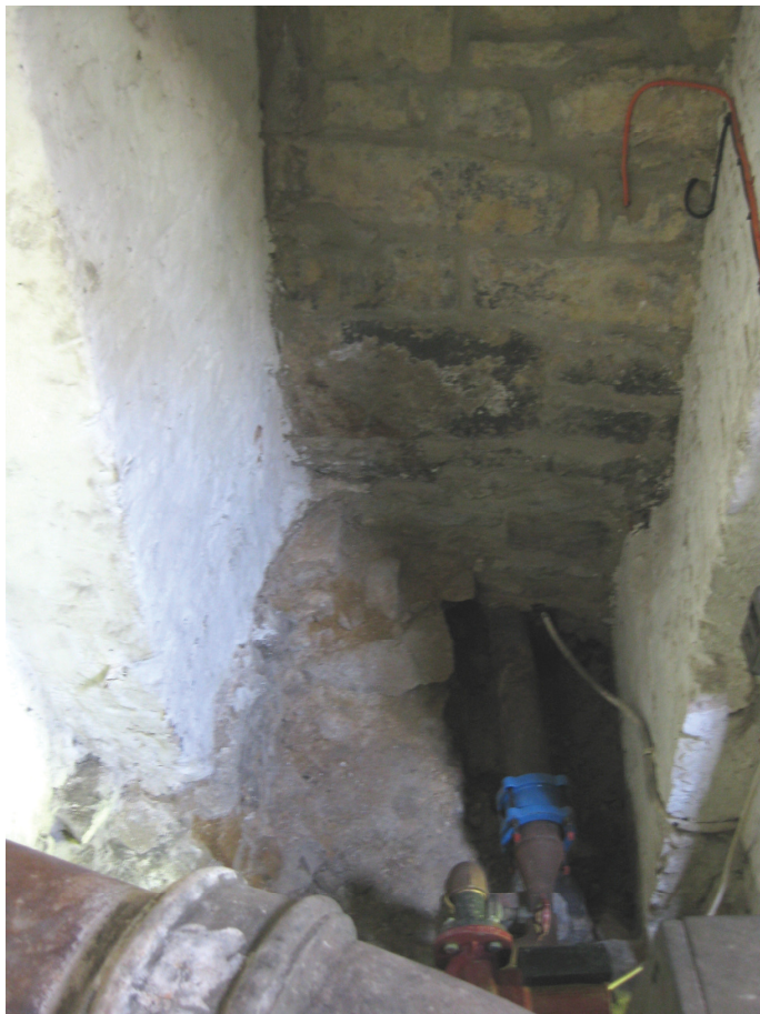
Plate 5 Detail of recess base, showing original wall core cut through by pipe duct
