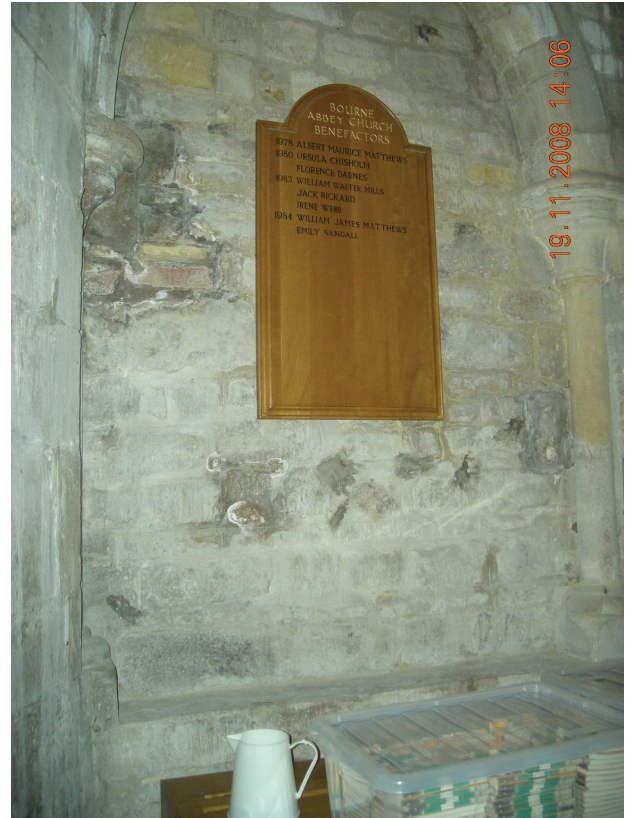
Plate 2 Blind arch located beneath the southwest tower, showing squared shelf of ashlar and different stonework for comparison
