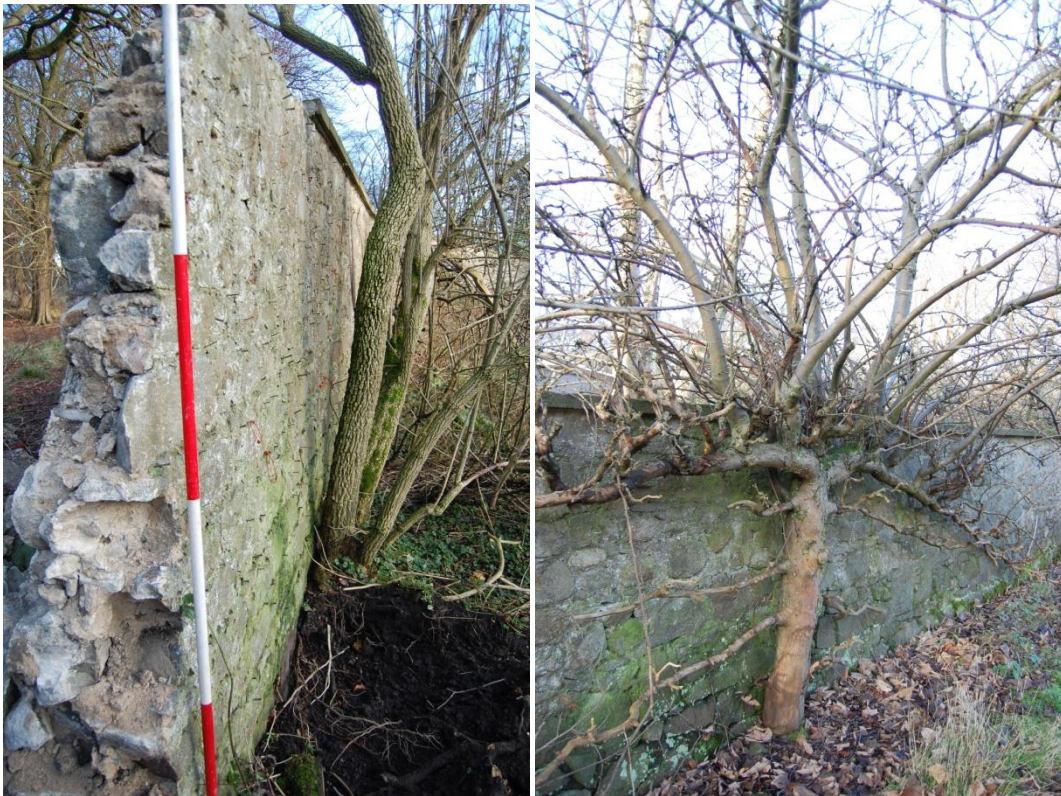
Figure 35 Area S3 North wall F30 showing nails for espalier of fruit trees (left) and remains of horizontal espalier (right)
