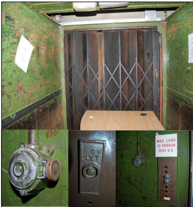
Illus 12 lift L1 (above) and lift controls (below)
