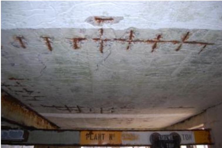
Illus 22 Building 6a: roof showing plank marks from shuttering and reinforcing bars rusting and appearing through the concrete
