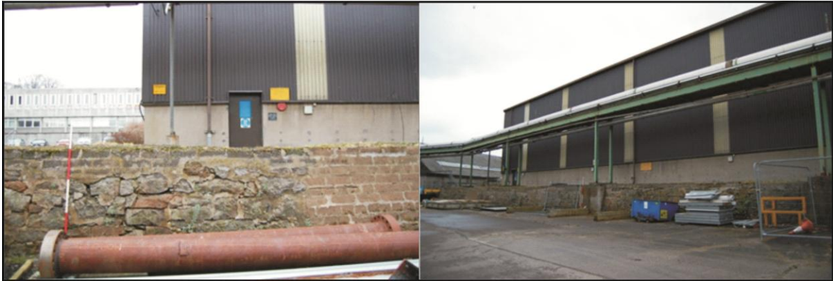
Illus 14 Building 3 (foreground left) with B19 and overground pipework (background; right detail of B3 facing south
