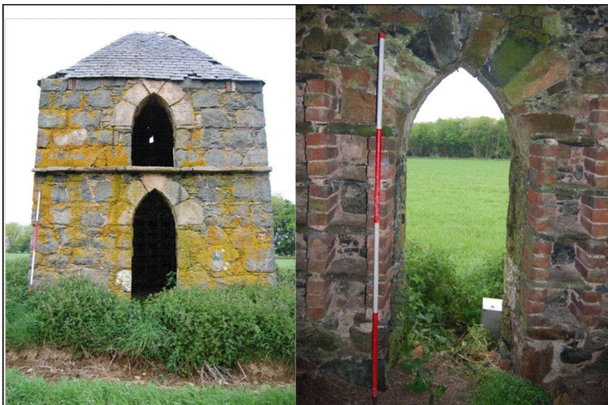
Illus 3 (left) South facade showing door 1 (below) and Window 1 (above) (right) Door 1 showing use of grey, pink and black granite and quartz blocks; note the nesting boxes surround the door
