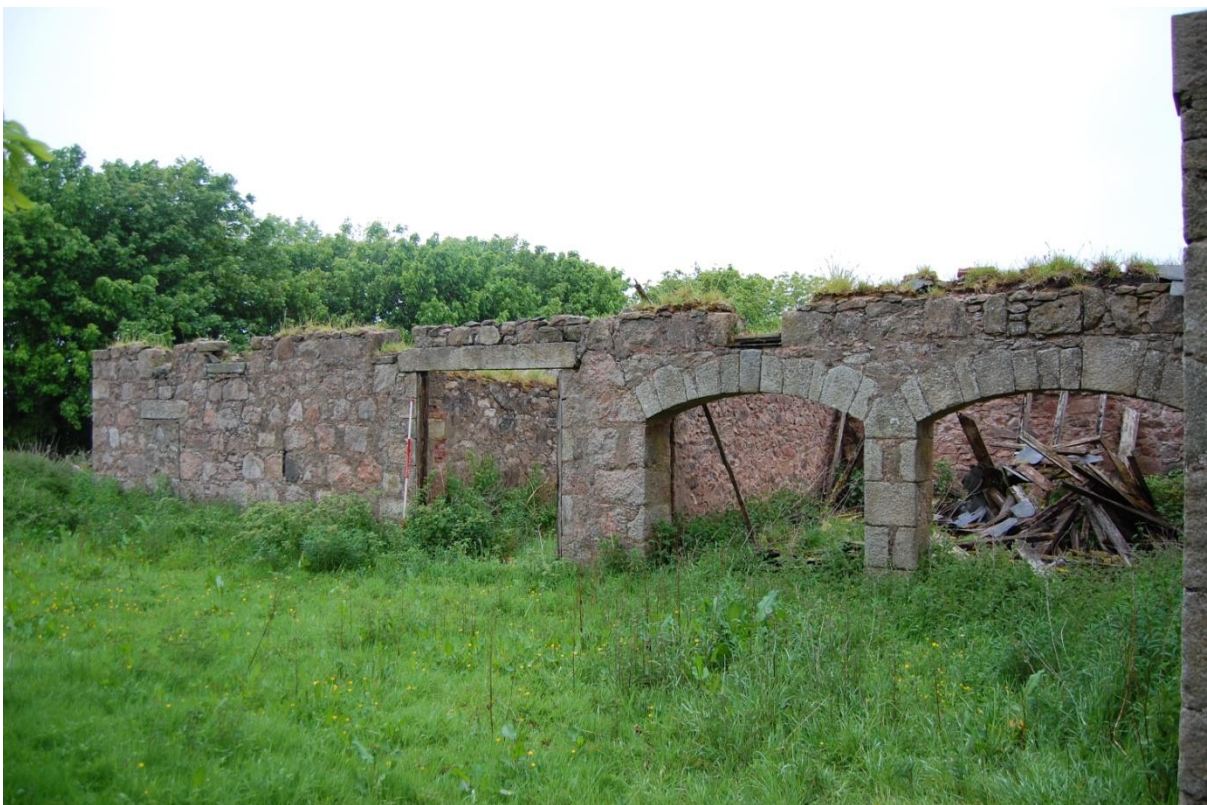
Illus 20 South wall of south wing with Door 12 (centre) and coach doors D12 and D13 (right)
