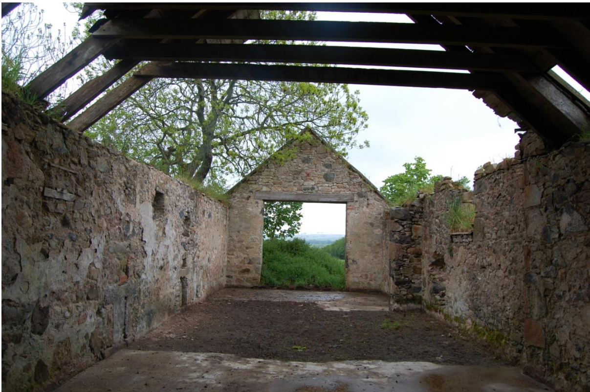
Illus 16 Room 8 showing apertures A1-A6 (left) and wall stub (middle right) the original south end of this room
