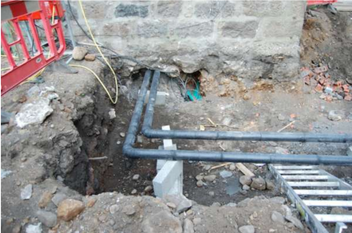
Illus 5 Trench for electricity cables; the level of the natural subsoil can be seen immediately below the foundation of the rear extension to 52 College Bounds (Section 1 Illus 2)
