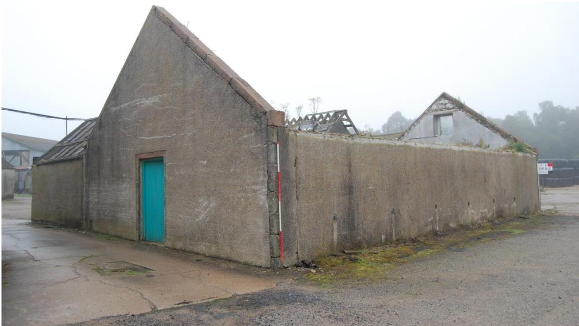
Illus 4 Room1 showing Door 2 (left) and ventilation pipes in east wall facing NW
