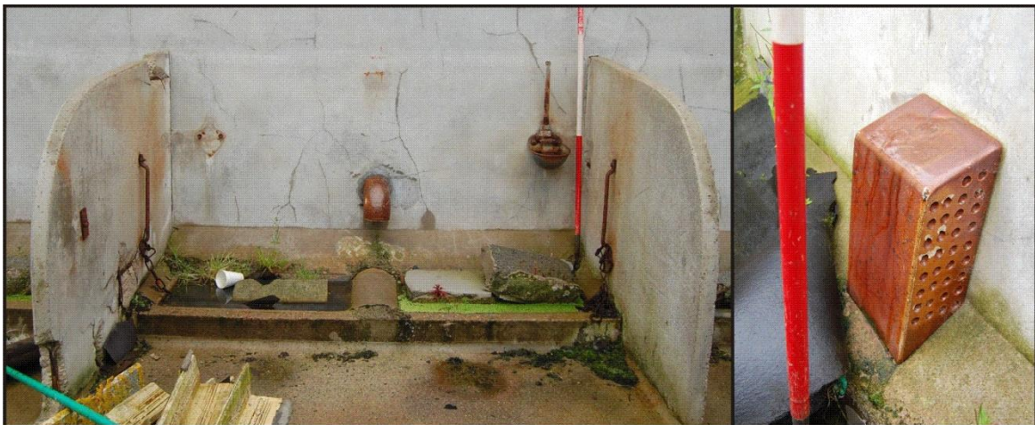
Illus 6 (left) reinforced concrete partitions, trough and fireclay pipes to external wall (right) fireclay ventilation through partition wall
