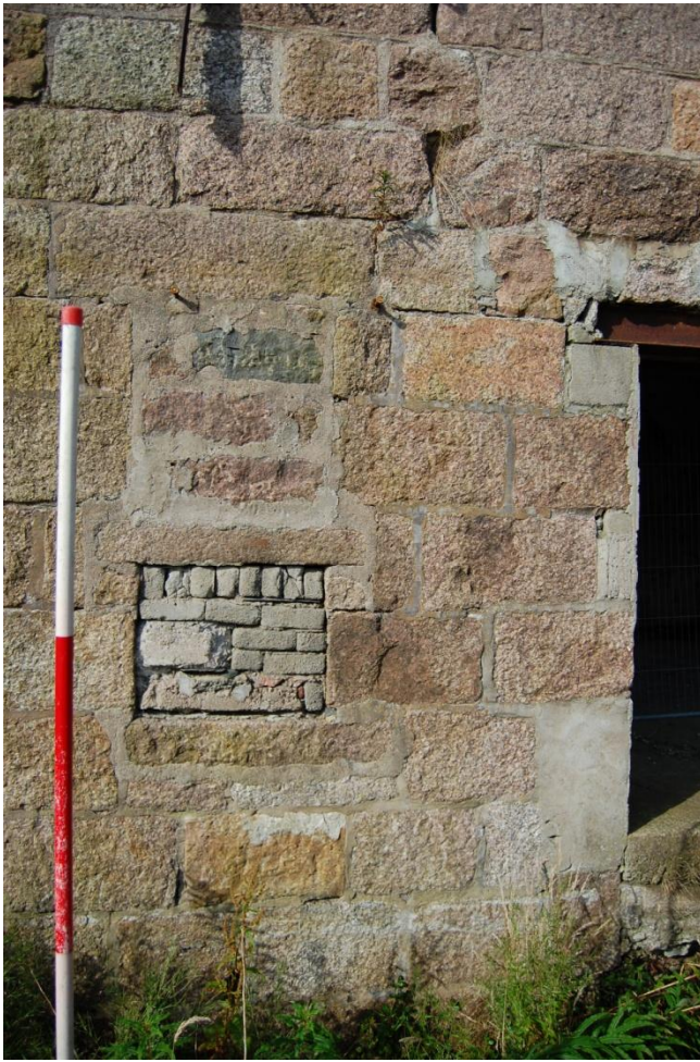
Illus 11 Room 4 east elevation detail showing threshing mill apertures W6 (above) W7 (bottom) and D14 (right).
