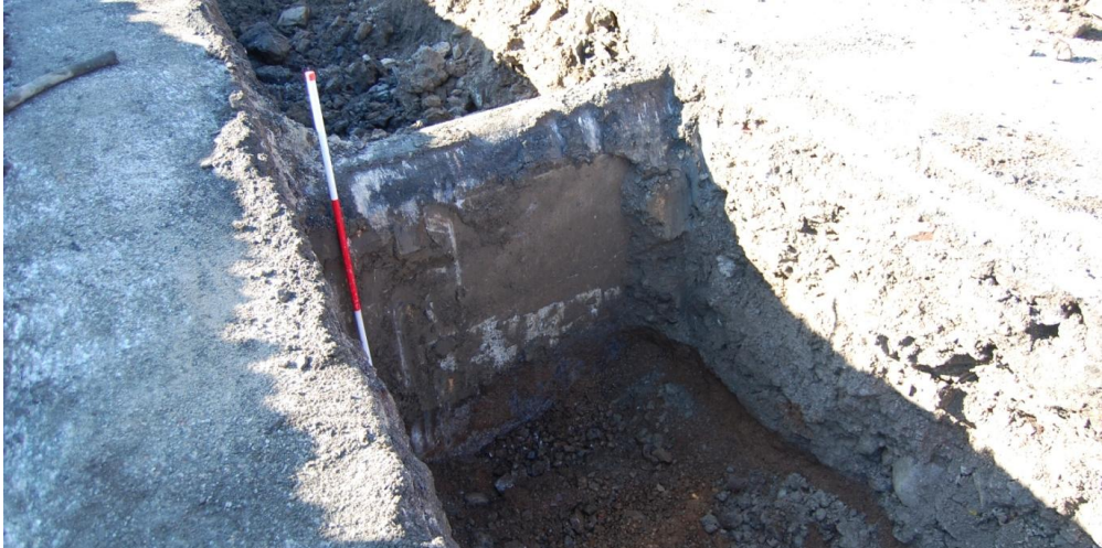
Illus 4 Shuttered poured concrete partition F1 within late 19th-century filter beds; facing WSW
