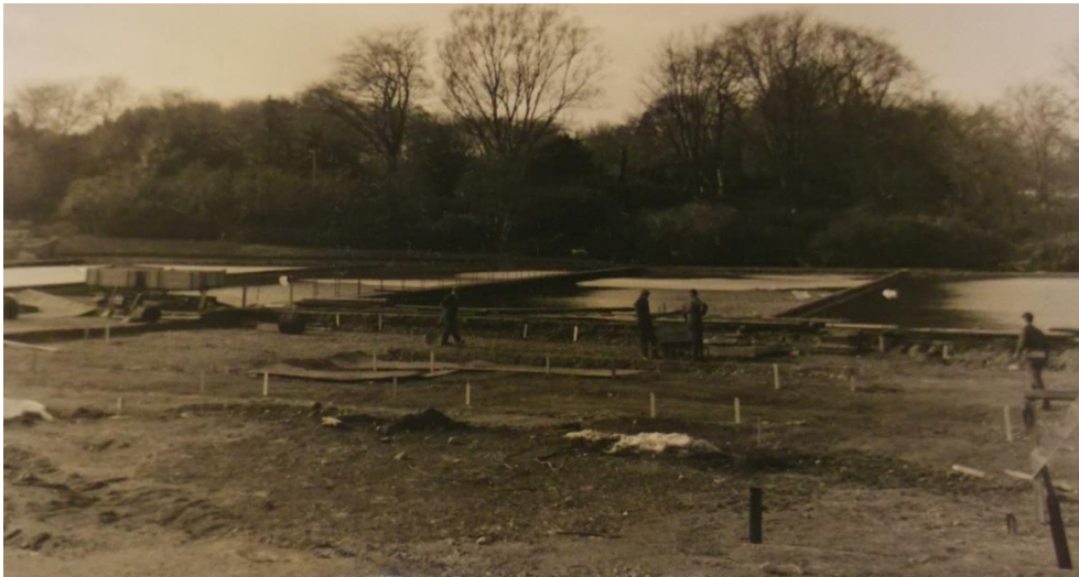
Illus 6 Chemical house and filters being constructed in 1947; the original late 19th-century filter beds can be seen in the background (copyright The Papeterie, Arjo Wiggins).
