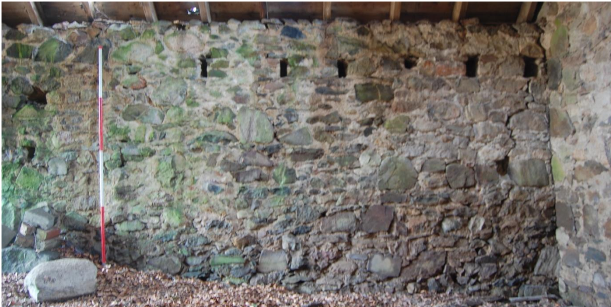
Illus 10 Building 1 interior of west wall showing beam slots F109 for mezzanine floor in north half of room; facing W
