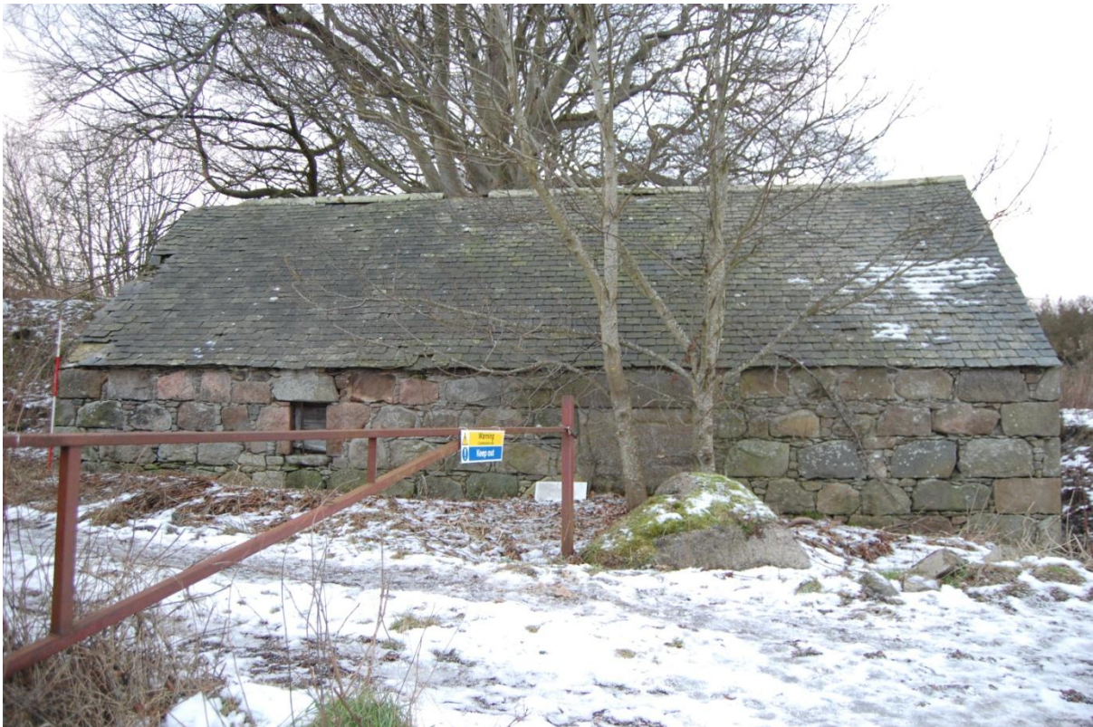
Illus 7 Building 1 east wall with Window 1 (left) and Door 1 (blocked; behind tree); facing W
