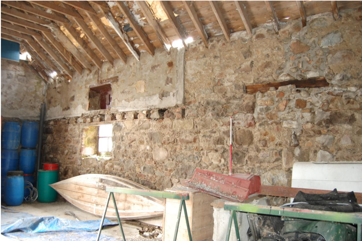
Illus 6 Room 2 west wall showing blocked aperture for mill mechanism (right) and beam slots for upper floor (left); facing SW.
