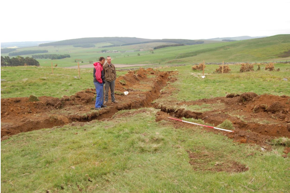
Illus 15 Cable trench junction to Base 1 (left) and Base 2 (right); facing SW
