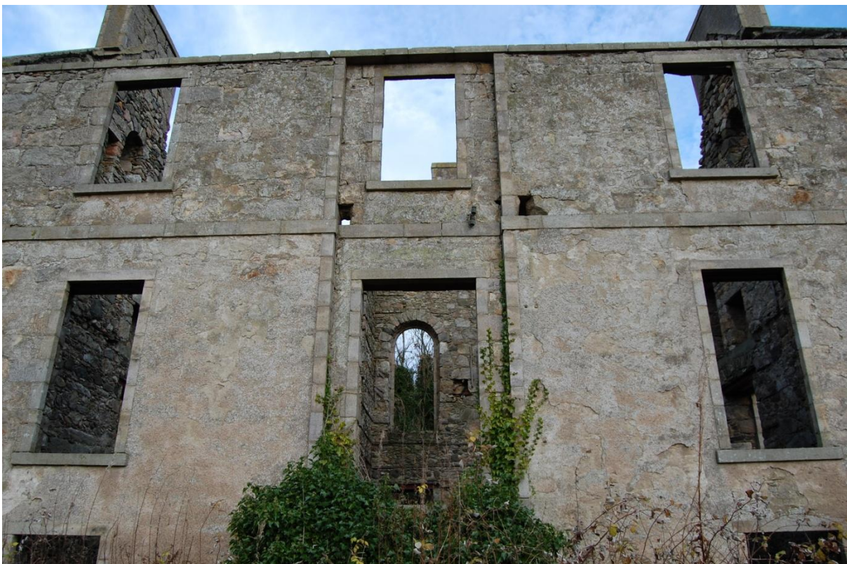
Illus 6 Front south facing facade with front door (bottom centre); the arched window in the north wall can be seen through the door aperture; facing north.
