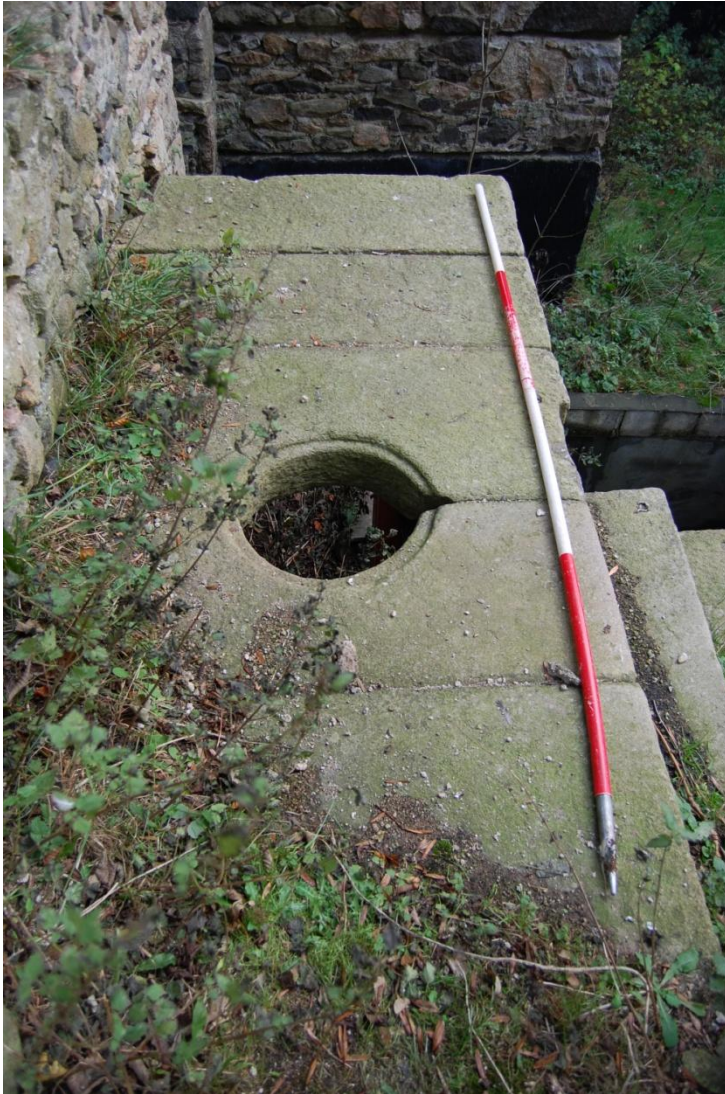
Illus 10 Granite threshold inside the back door which led into the stairwell to the basement; the original stairs would also have been set in this extension; facing east
