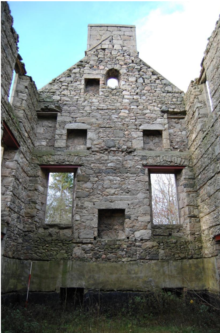
Illus 15 Interior of west gable showing one fireplace on ground floor, two on first floor and a small fireplace in the second floor attic room; lightwell windows can be seen at the bottom of the photo and also the tar waterproofing; facing west.
