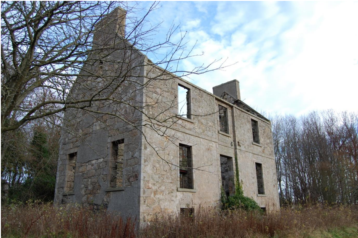
Illus 5 Frontage of house from NW showing recessed central bay with front door and upper window; lower window overgrown and visible from interior only; facing SW.
