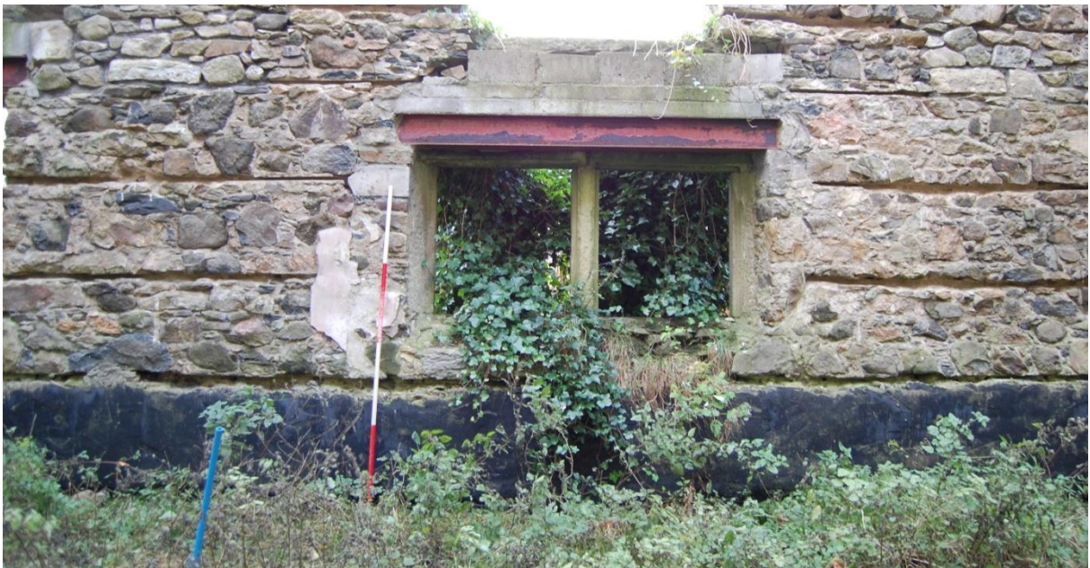
Illus 11 Lower ground floor window in centre of south wall under main front door with central mullion surviving; facing south.
