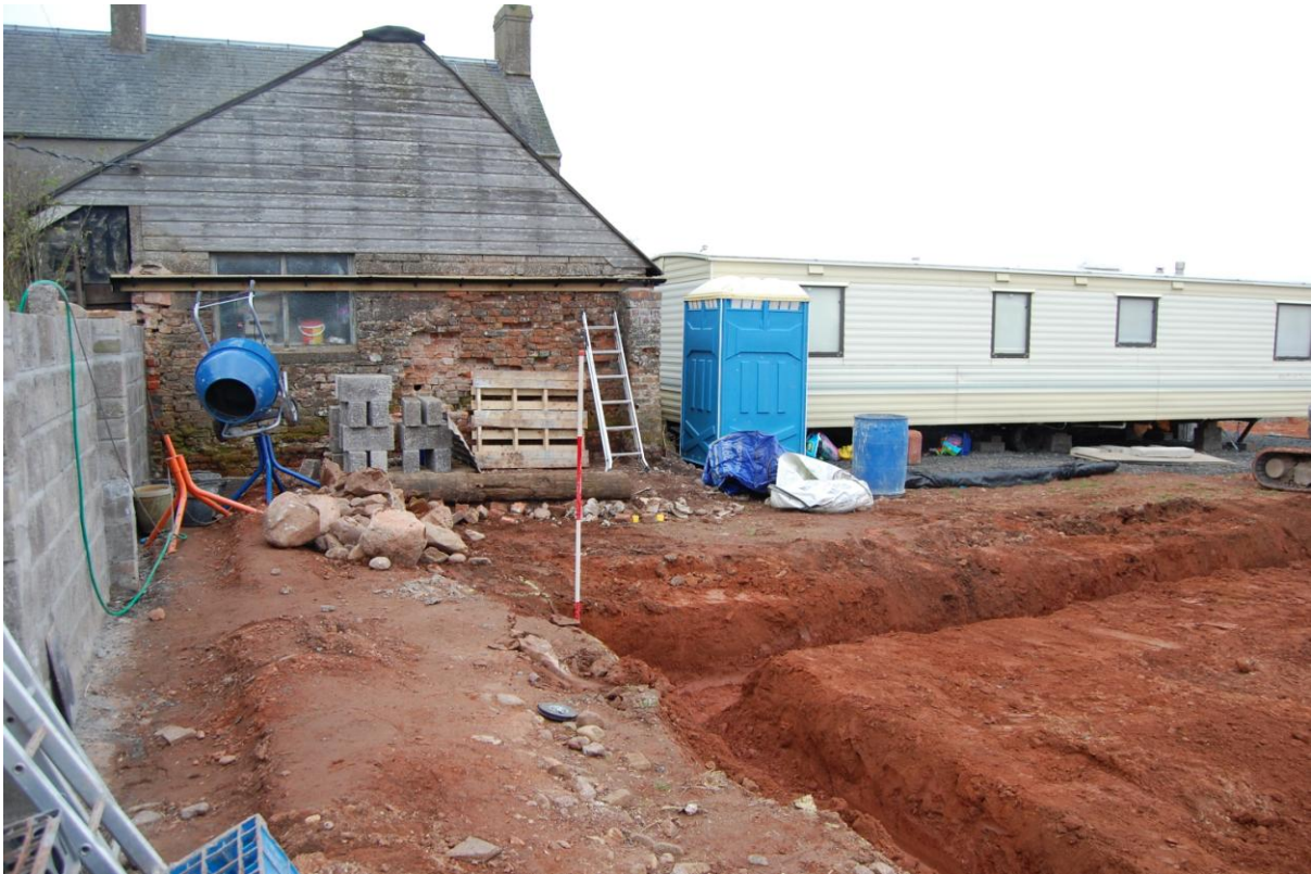
Illus 5 Foundation trenches for garage with hand-made brick building (outwith current development) in background; facing south
