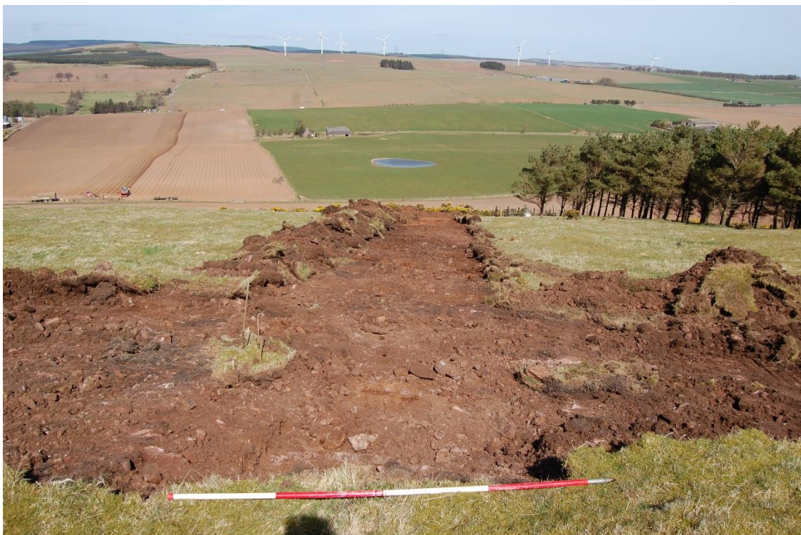
Illus 3 SW trench and turbine base showing shallow topsoil and rocky natural; facing NNW
