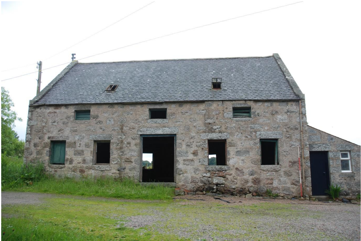
Illus 4 NW facing façade of Building 2 the granary with later extension (right); the date stone is above the central door
