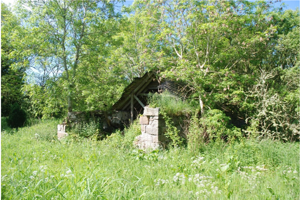
Illus 26 Building 7 east end showing poor condition and overgrown vegetation on the interior of the building; facing SW
