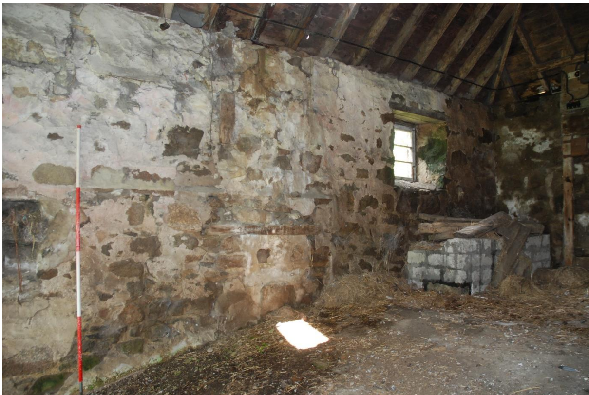
Illus 22 Interior of west wall showing infilled aperture (centre) possible location for former millwheel; facing NW
