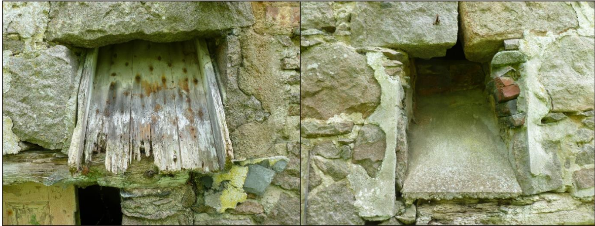
Illus 11 Wooden (north) grain chute (left) and southern concreted chute (right); facing SE
