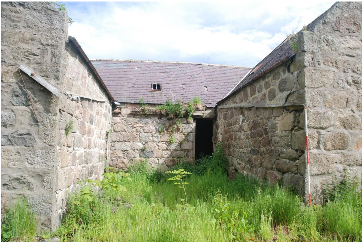
Illus 20 Courtyard on south side showing scar where building has been infilled in small courtyard (see Second Edition OS); facing N
