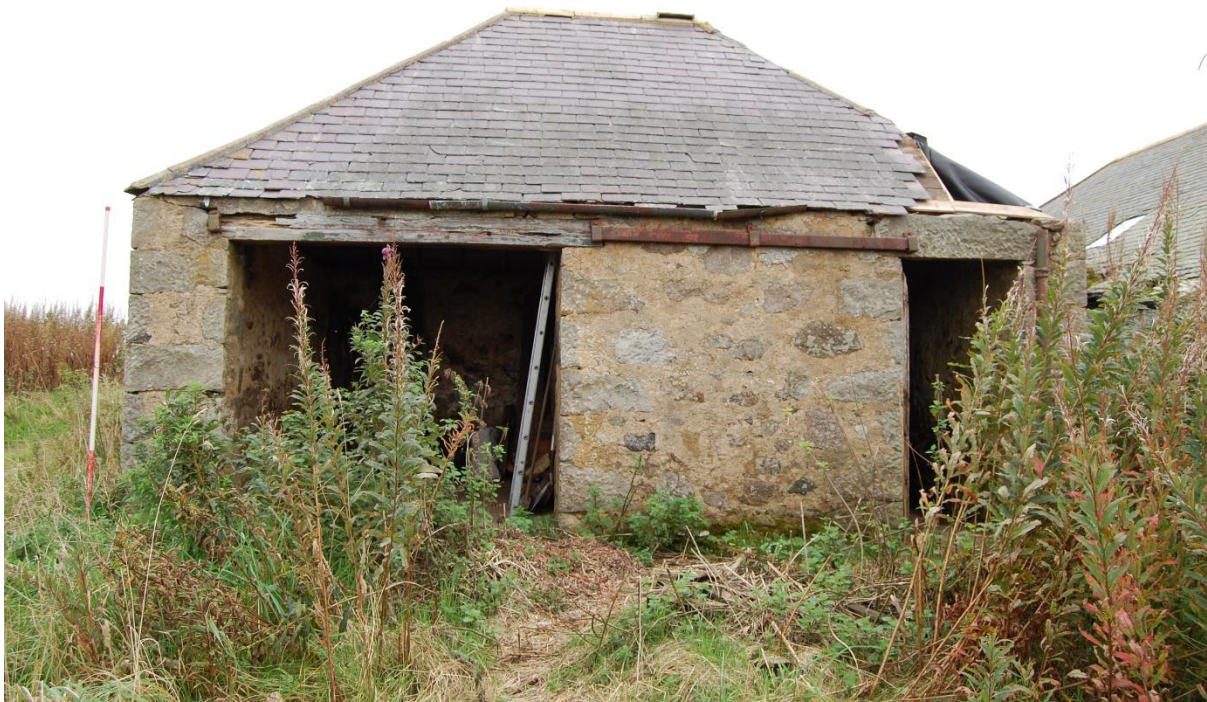
Illus 7 Cart shed west wall with Door D3 (left) and D4 (right)
