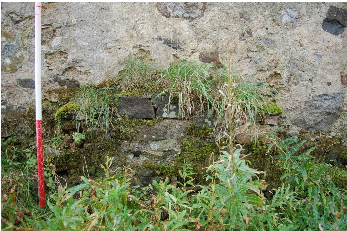
Illus 6 Mortared stone extension on north wall of steading where horse mill attached to the main building; F4 and F5 are heavily mortared on the exterior and not visible
