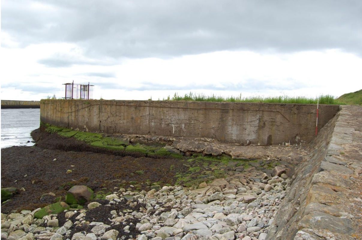
Illus 12 Skate's Nose Jetty from west showing substantial stone foundation raft; facing north-east
