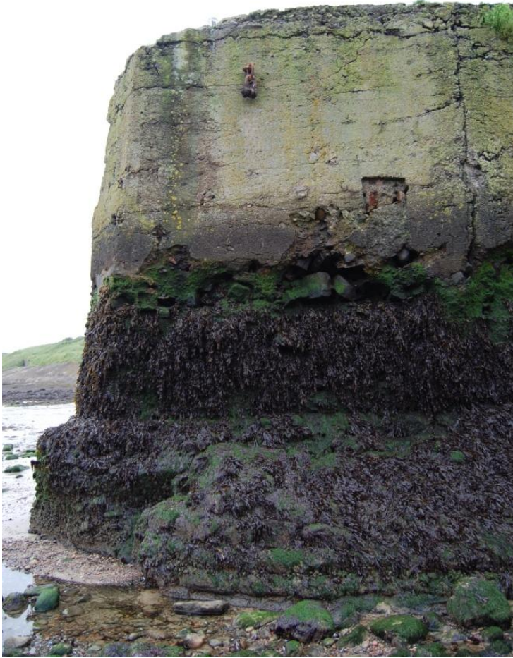
Illus 14 Skate's Nose Jetty: north end of the jetty showing layers of concrete, stone foundation and metal mooring rings; facing east.
