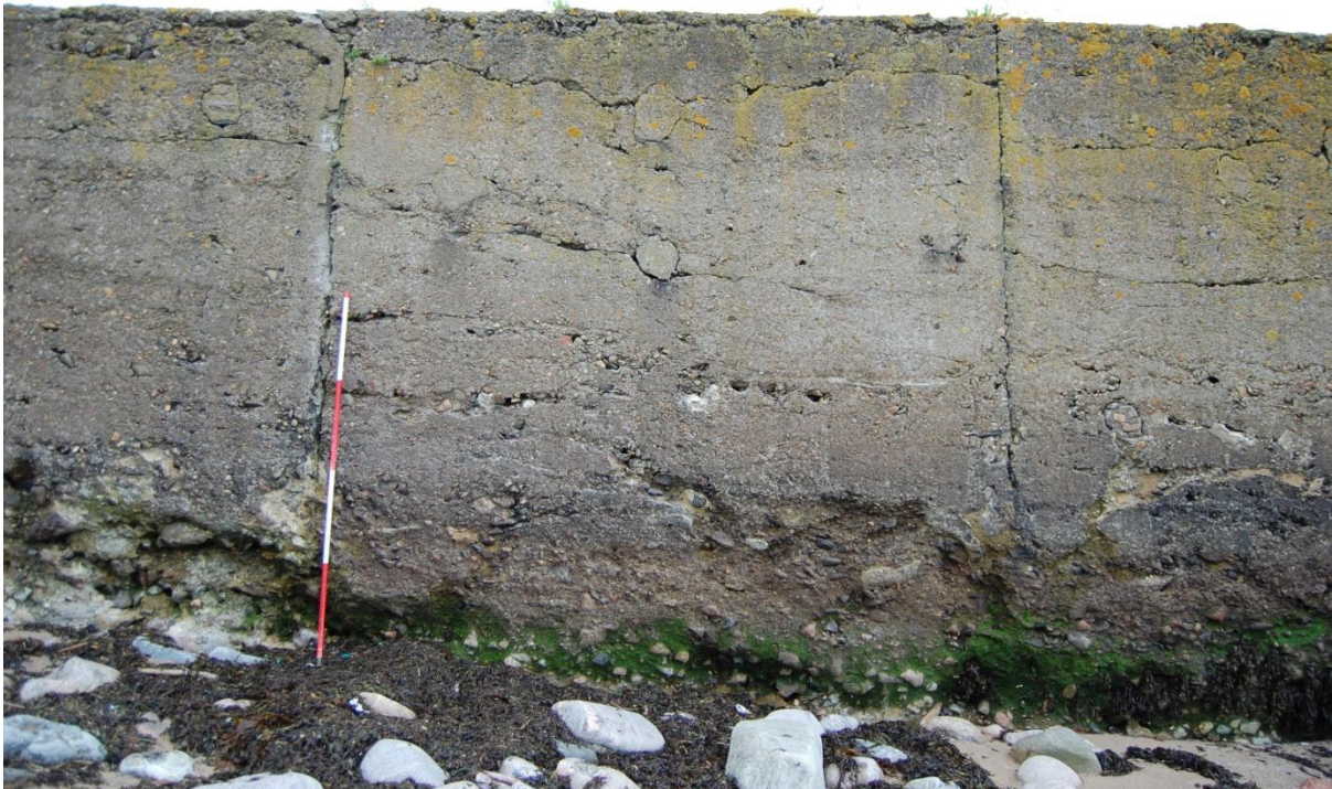
Illus 13 Skate's Nose Jetty East face of the jetty showing vertical pouring scars between each shuttered section of poured concrete and horizontal bands of concrete batches; facing west
