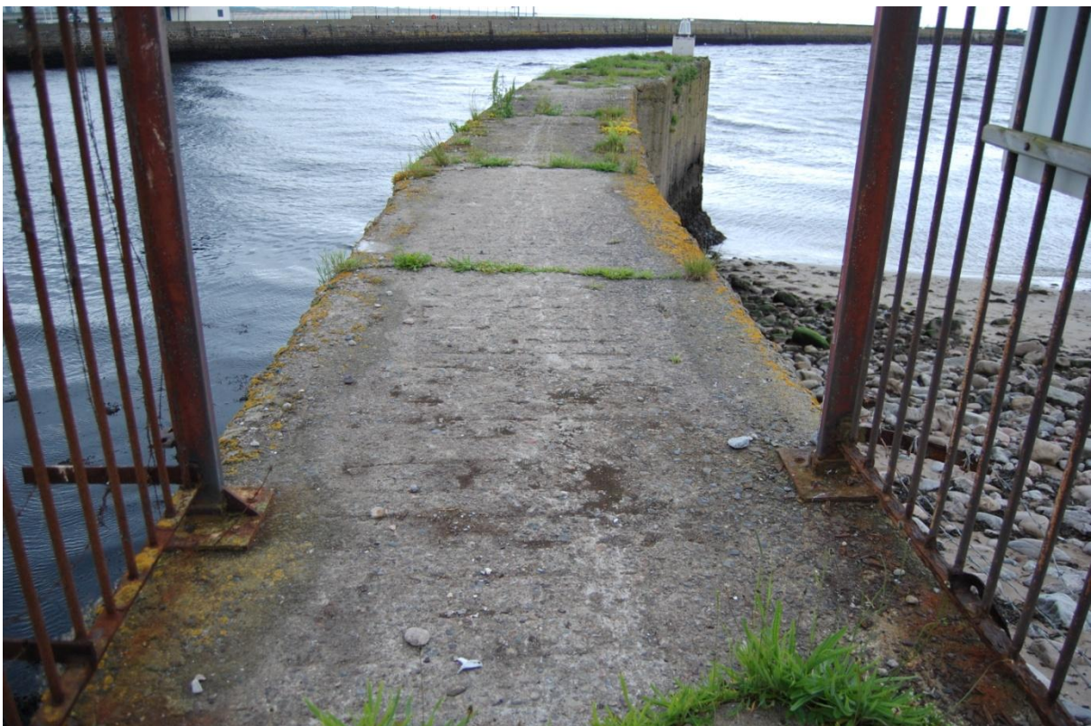
Illus 11 Skate's Nose Jetty showing area (behind metal barrier) to be demolished; facing north
