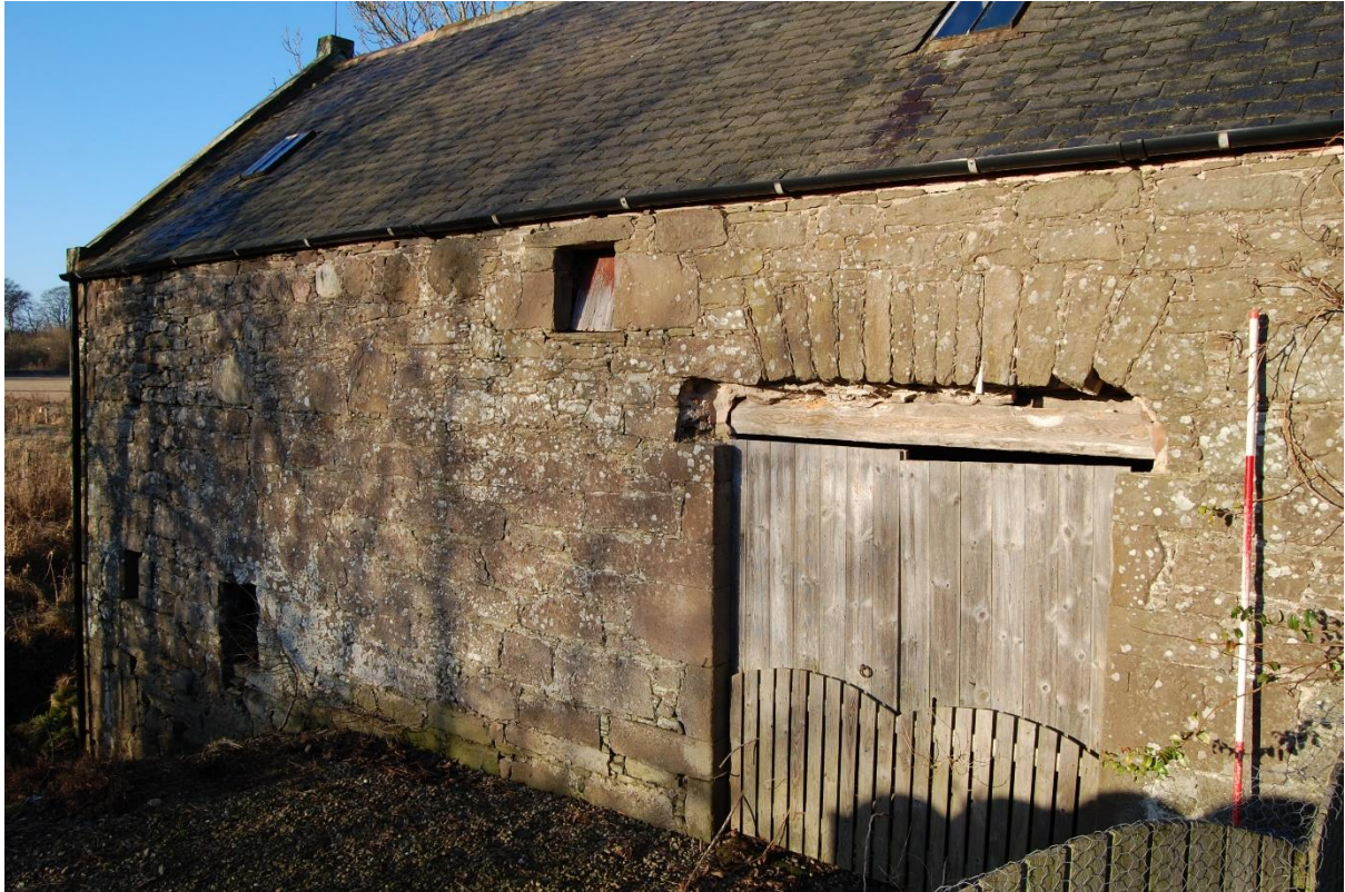
Illus 5 Phase 1 SE wall with lade (left) and Door D17 (right); facing W
