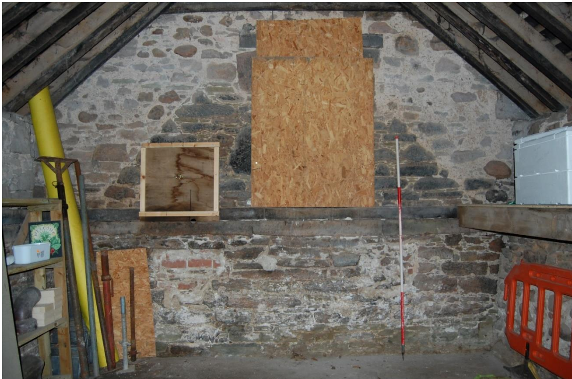
Illus 26 Room 2 exterior gable (now within room 1) showing Phase 1 gable F11 (centre) and Phase 2 gable and walling; facing SW
