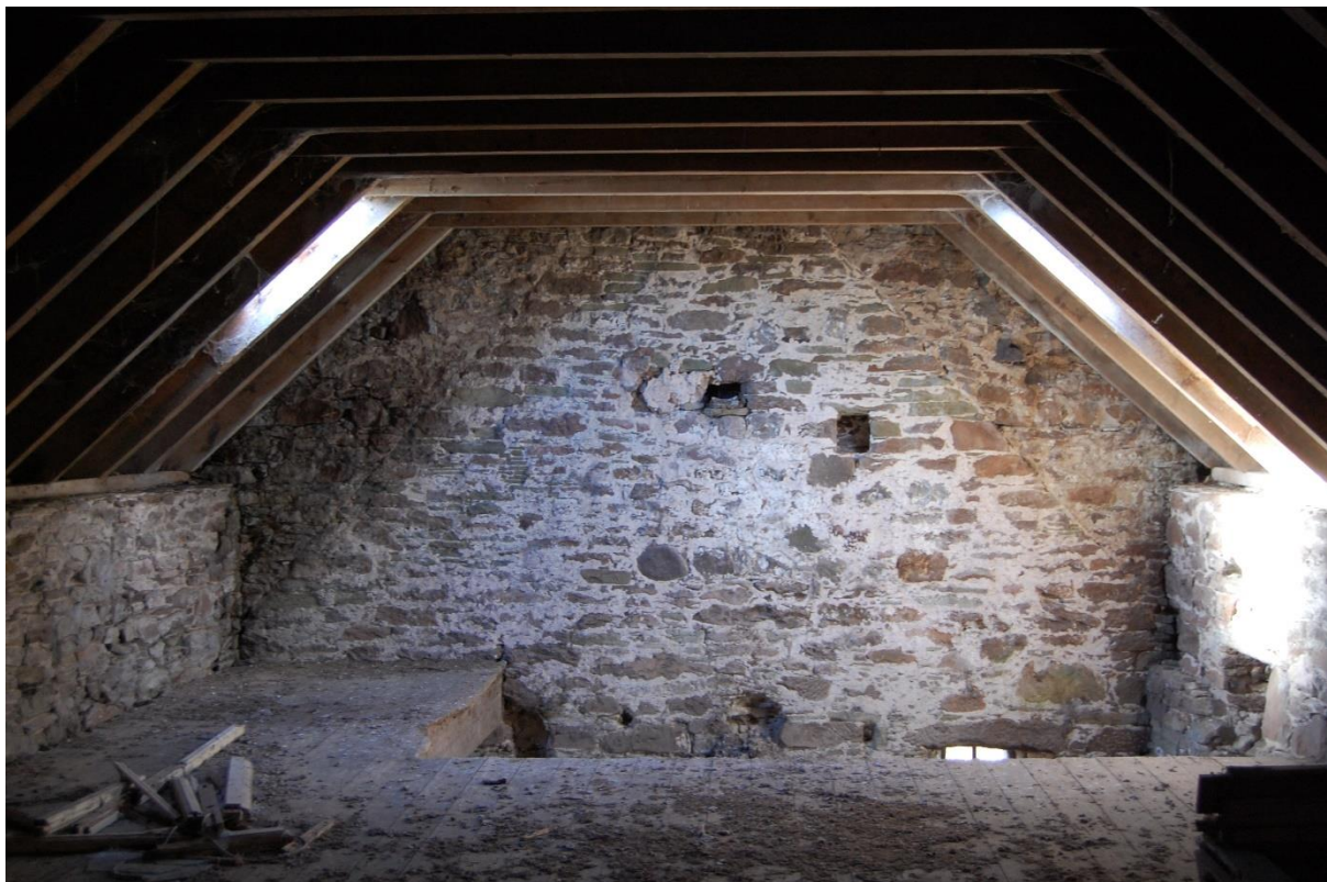
Illus 12 Interior of SW gable, not accessible and visible through a hole in plastic sheeting; facing SW
