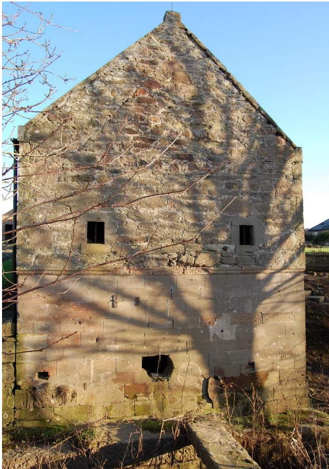
Illus 8 Phase 1 room 2 SW gable showing sandstone ashlar lower courses and sandstone rubble upper courses; facing NE
