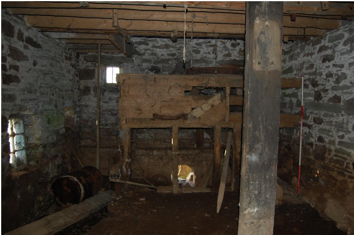
Illus 24 Room 2 interior SE gable with F1 aperture for mill wheel drive shaft (centre) and window W12 (top left) and wooden beam supports for upper floor; there is a thick layer of mud on the floor from a recent flood; facing SW
