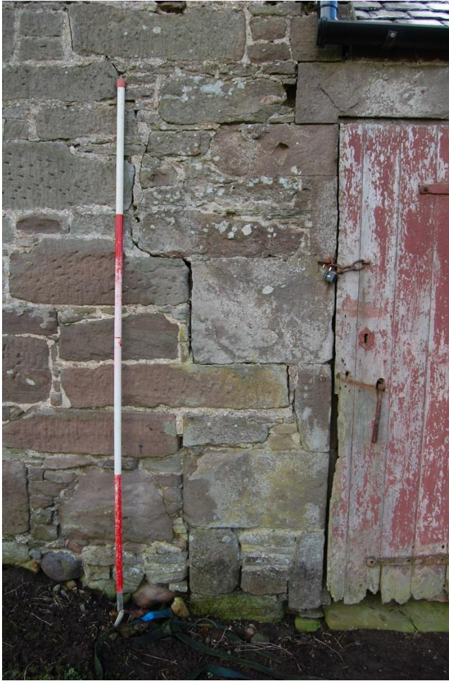
Illus 27 Phase 1 door D15 (right) and Phase 1 NE gable wall F19 (centre) built into Phase 2 wall (left); facing SE
