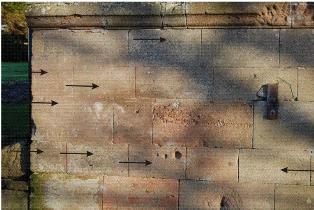
Illus 15 Detail of section of ashlar sandstone SW gable with at least eight mason's marks (arrowed); facing NE
