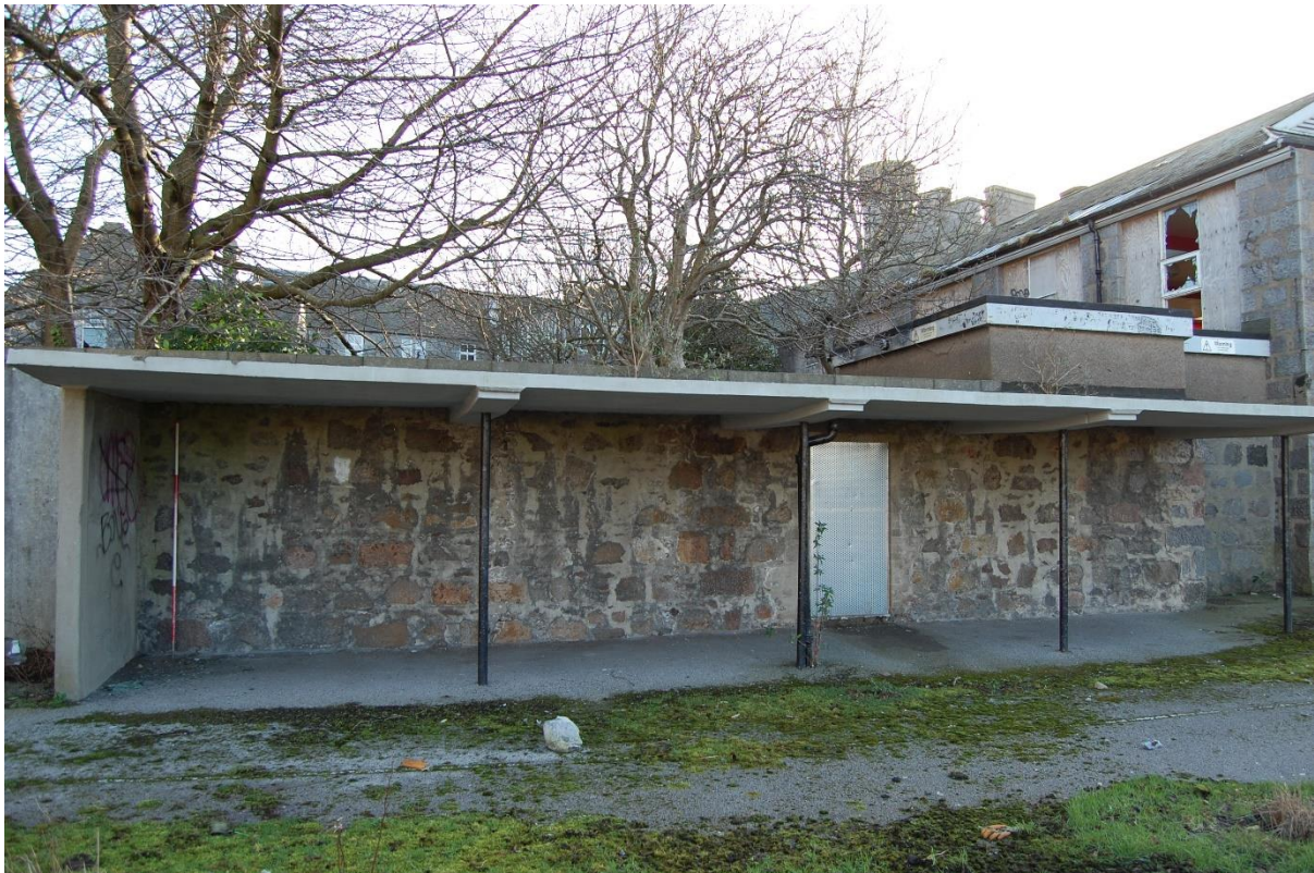
Illus 8 Building 2 open-sided shelter on the SE edge of the playground; facing SE
