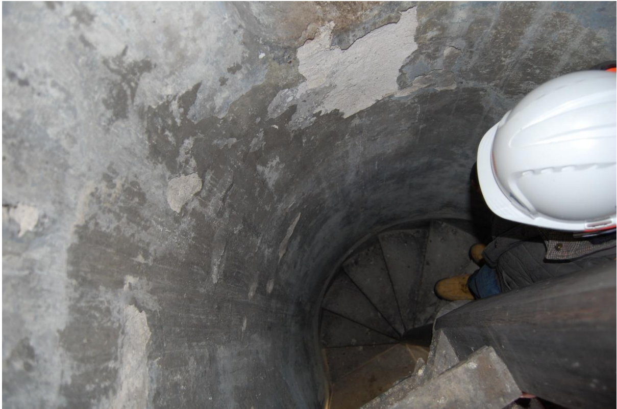
Illus 20 Building 6 tower stair turret showing narrow stair to roof; facing E
