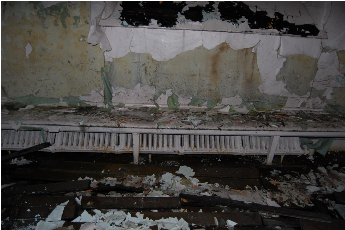
Illus 7 SE changing room showing radiators fuelled from adjacent boiler house; facing SE
