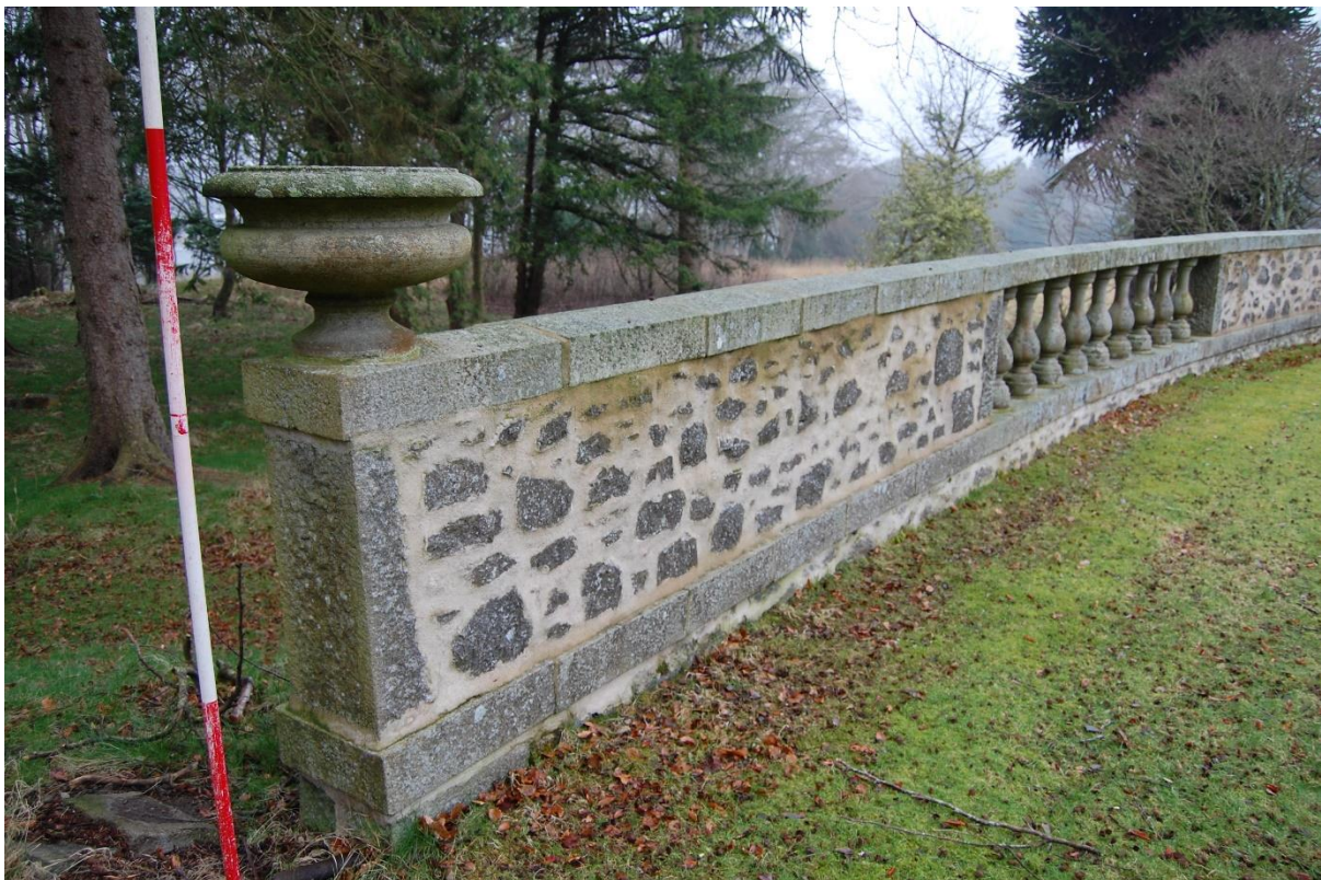
Illus 18 Wall 1 probably Phase 2; the garden was re-landscaped between the First and Second OS maps; facing SW.
