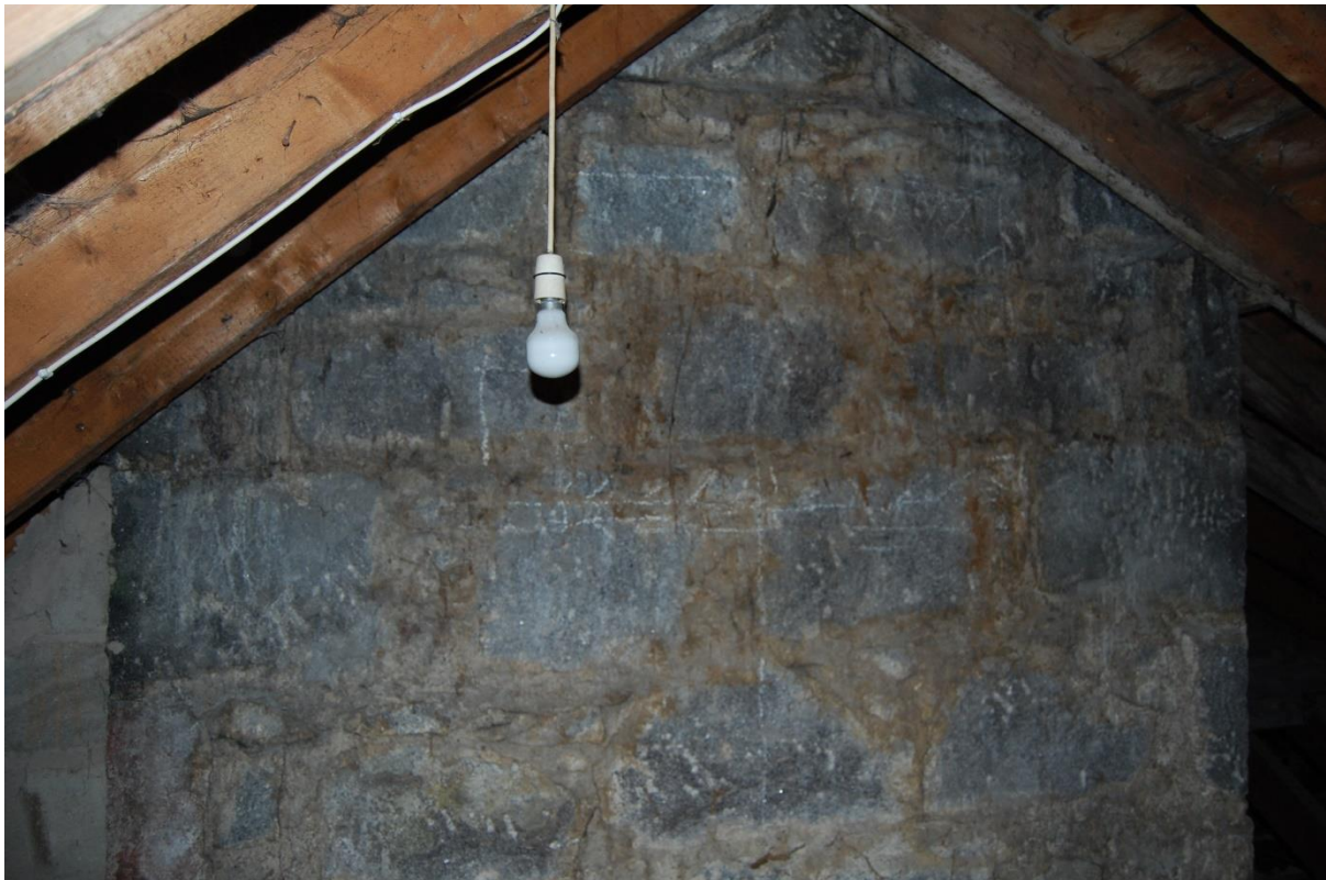
Illus 10 Exterior of Phase 1 gable chimney now built into Phase 2 loft space (above fireplace F6); facing SSE
