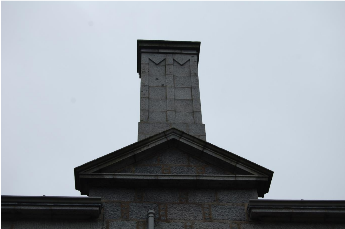
Illus 11 Detail of Phase 1 chimney stack design (Chimney 1; possibly replaced in Phase 2); facing ENE
