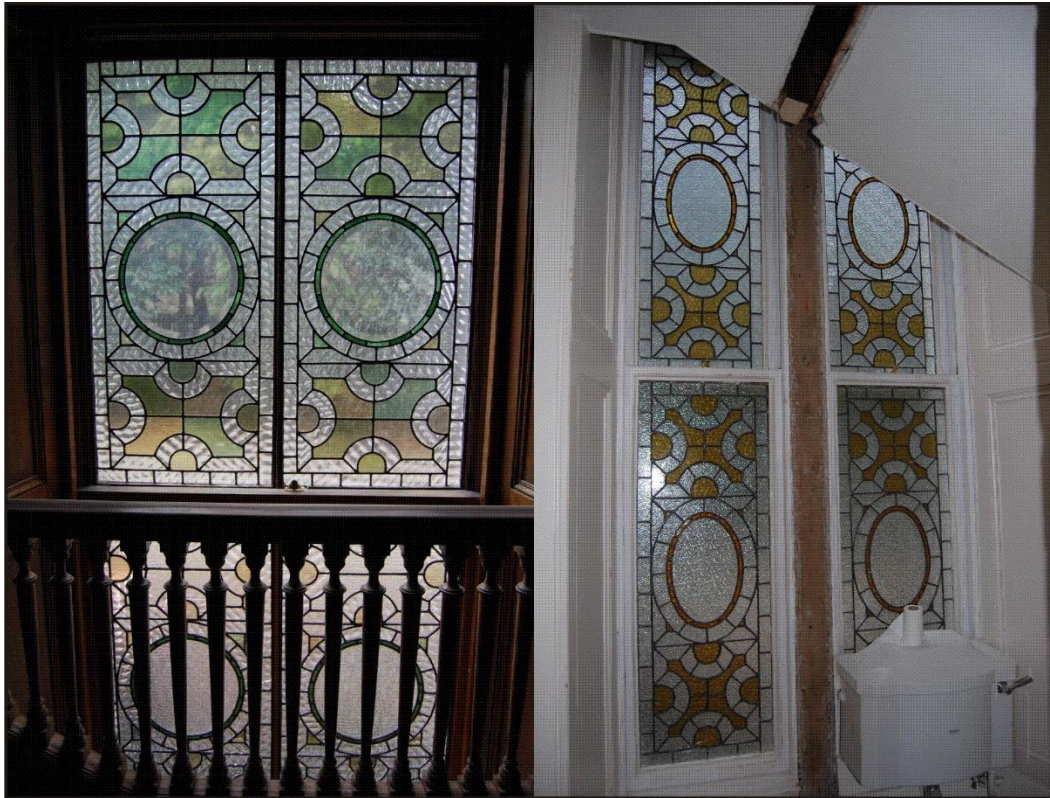
Illus 7 W13 (left) and W14 (Room 6 partially obscured by Phase 2 Stair 1); facing ENE
