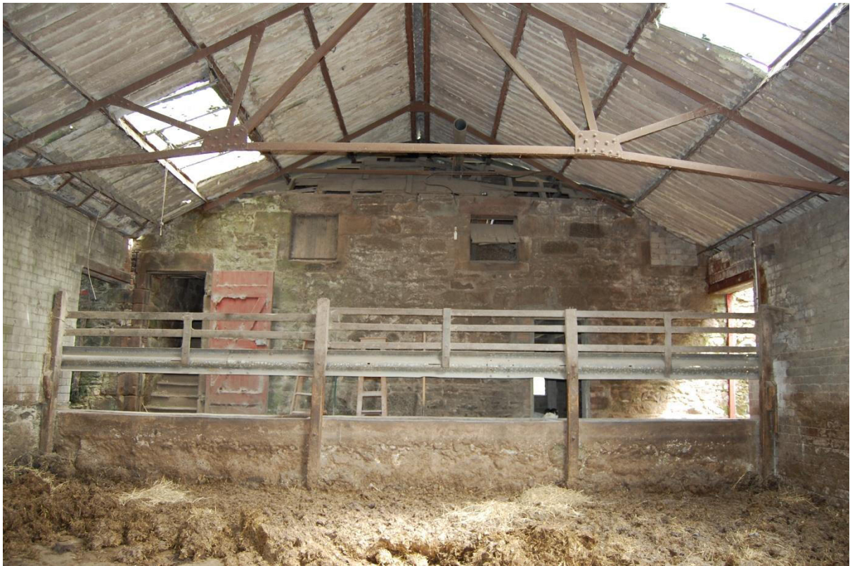
Illus 8 Phase 1 Room 10 D18 and D17 (below) Room 13 windows W17, 18, 19 (above) SW wall later built into cattle court Rooms 7/8; facing NE
