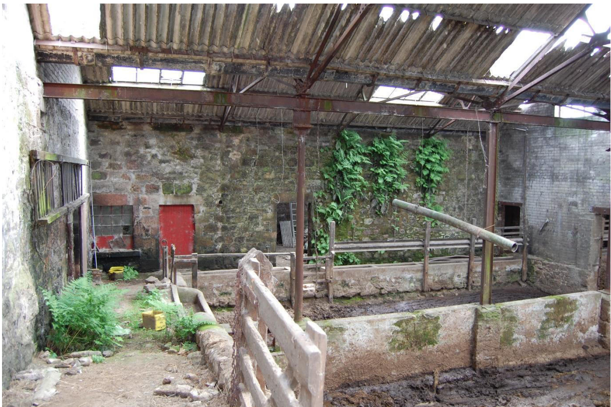
Illus 7 Phase 1 Room 9 SW wall built into later cattle court (Rooms 7 and 8); facing ENE
