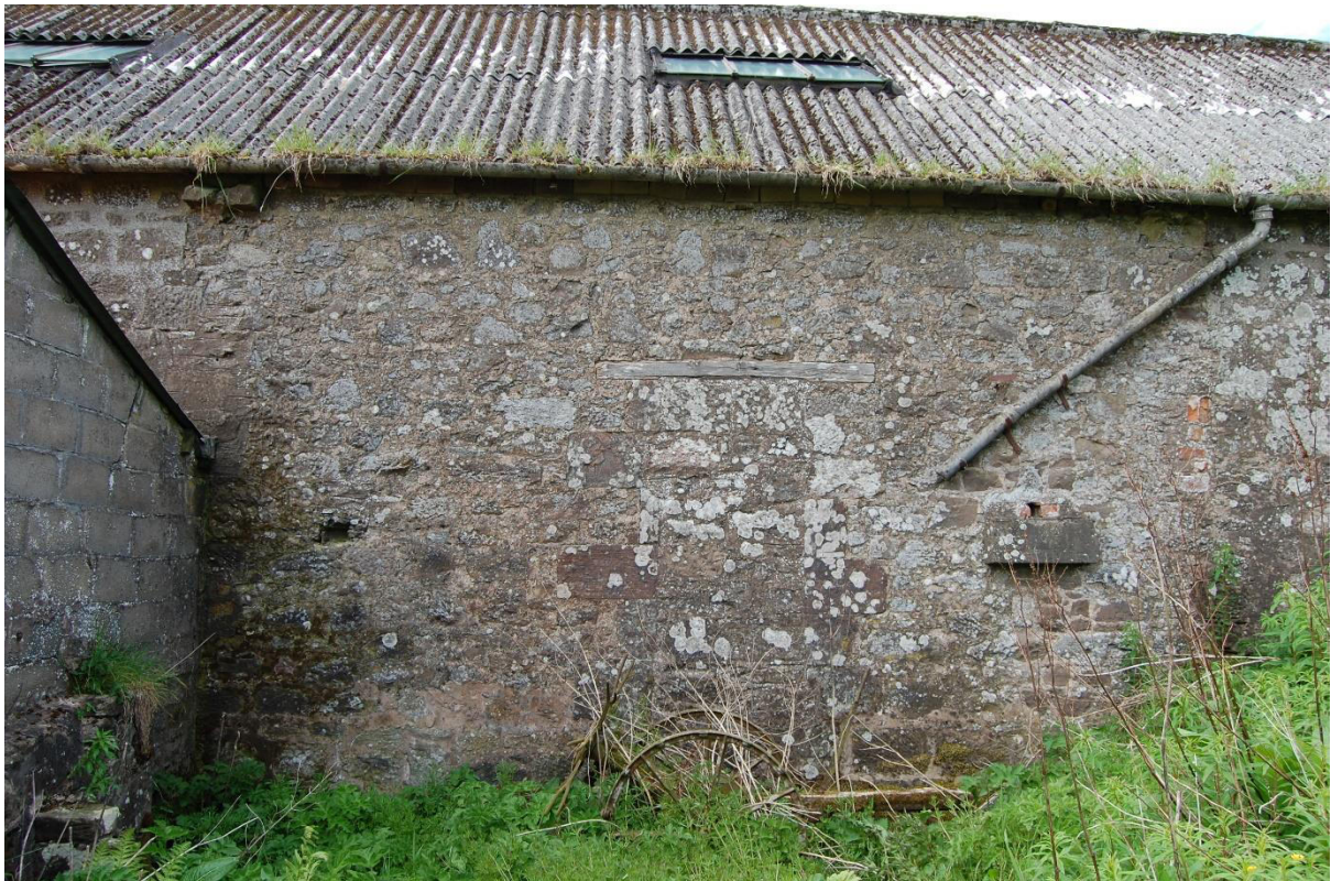
Illus 13 NE wall Room 9 with blocked door D7 (centre) and waterwheel fittings F5 and small aperture F6 (above); facing SW
