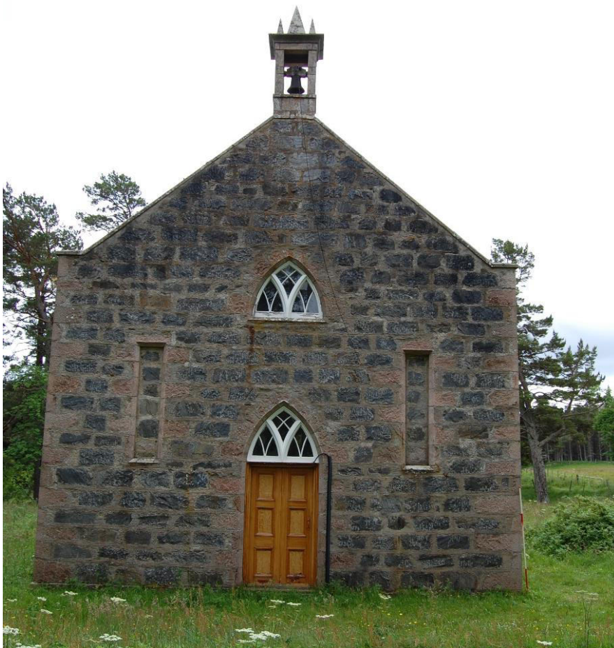
Illus 8 NNW gable with central door (1) first floor window (W2) and long narrow blocked windows (W1 and W3) with bell-cote above.
