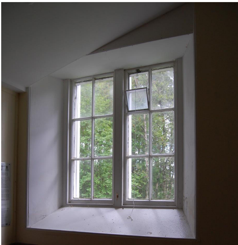
Illus 13 Window W7 lower section below gallery which bisected this originally larger window; facing ENE
