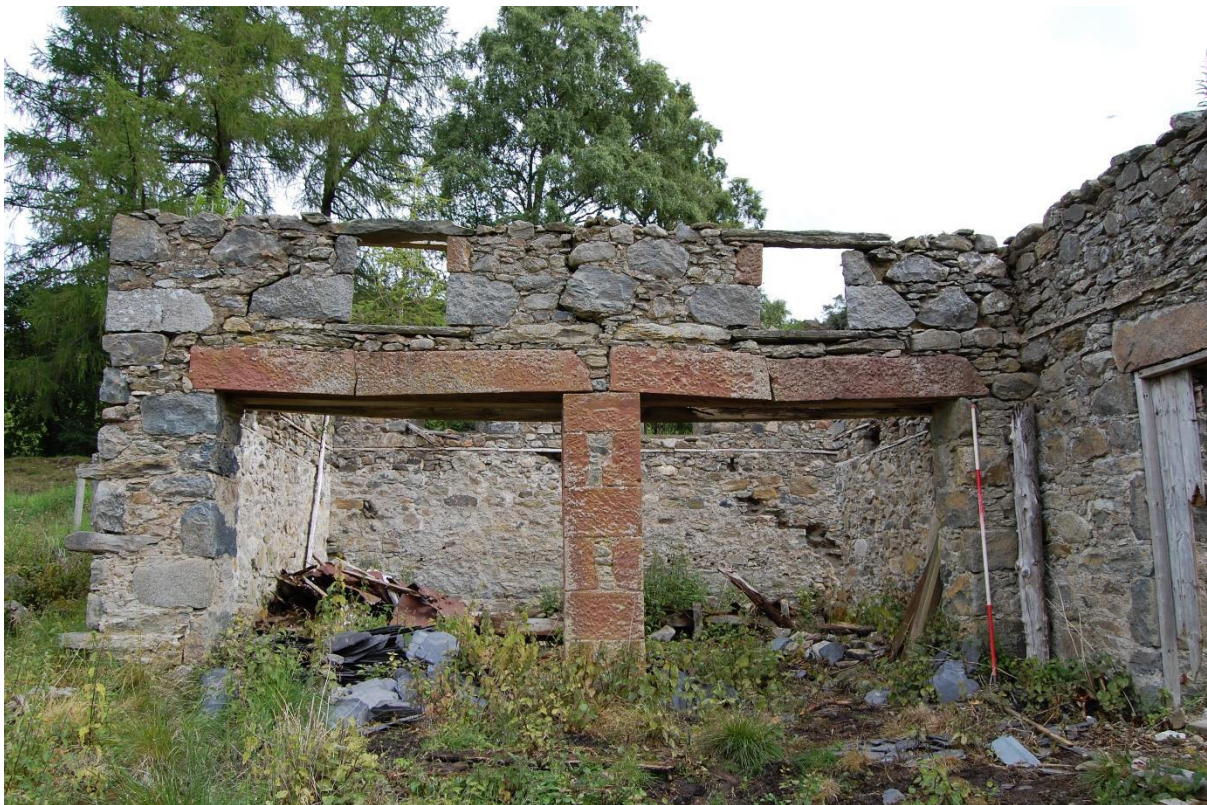
Illus 9 Cartshed Room 1 SW facade with Doors D3 (left) and D4 (right); facing NE
