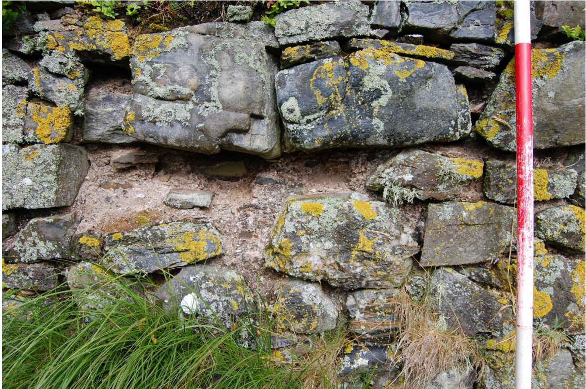
Illus 5 Interior E elevation with detail of missing stonework
