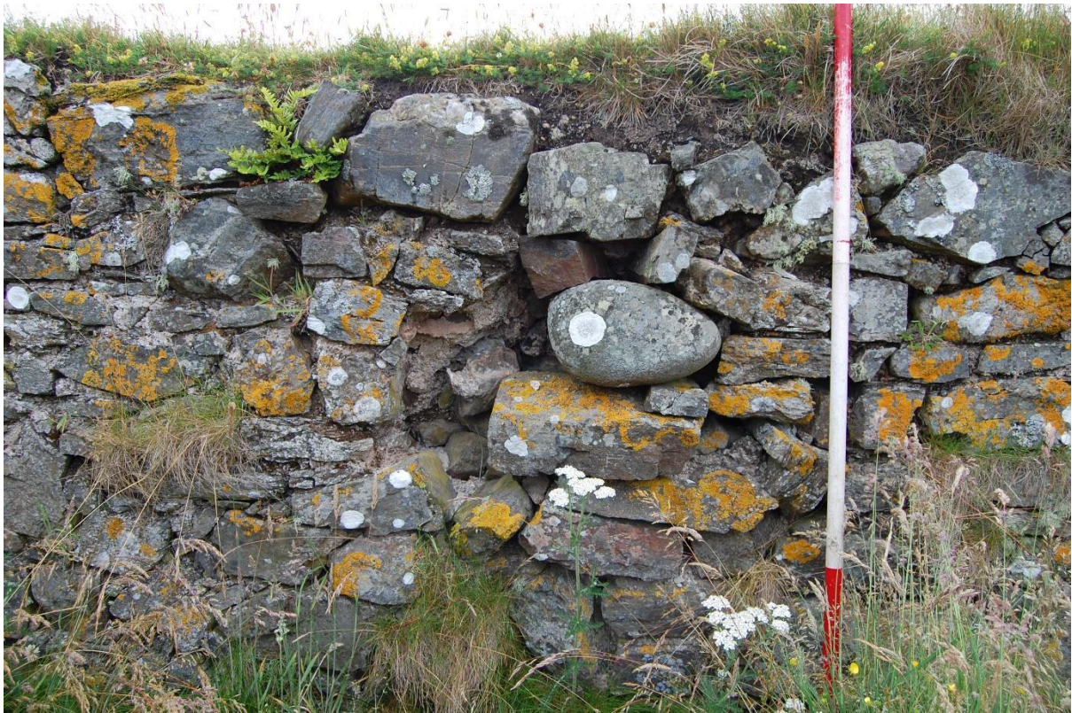
Illus 7 Interior E wall showing detail of bulge in wall where stones require to be removed, replaced and re-mortared
