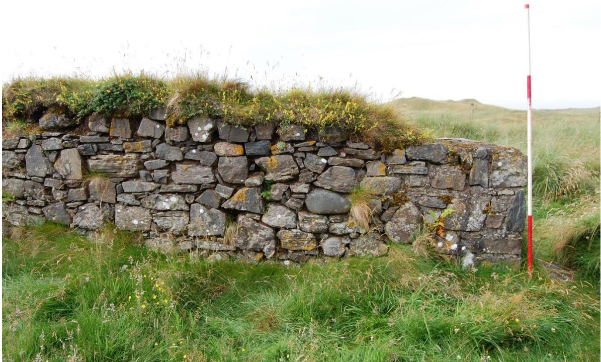
Illus 6 Interior S wall with South Door (right) showing mortared E jamb, vegetation on wall-heads and stones and pointing missing from wall
