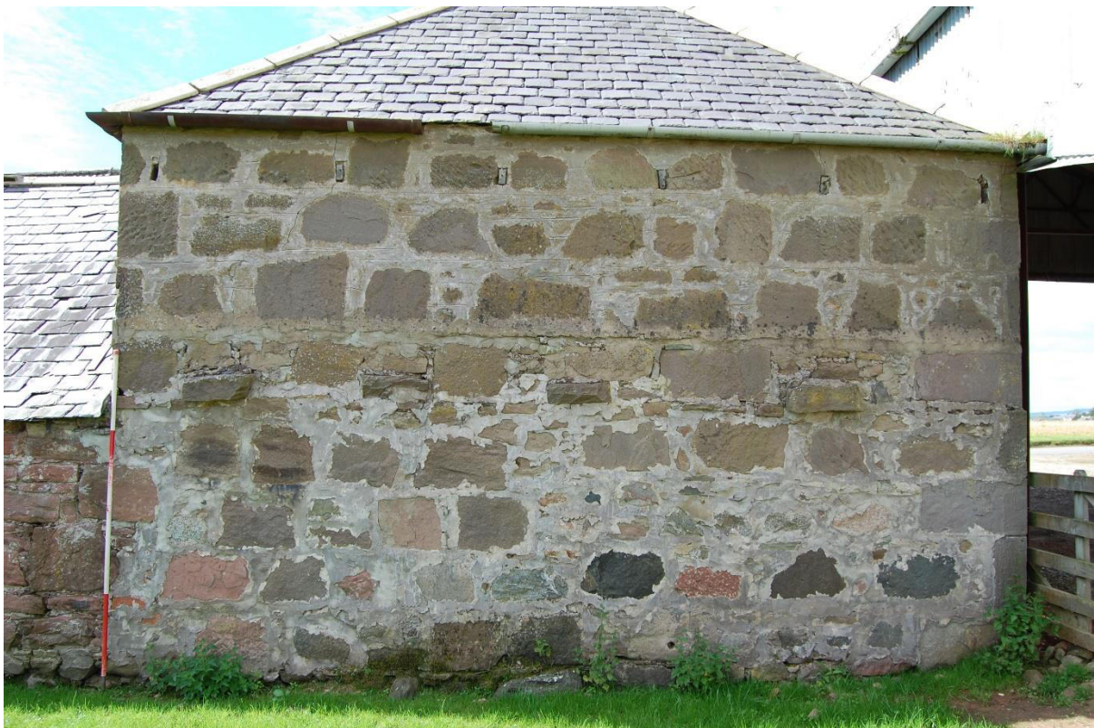
Illus 17 Room 3 NE wall showing joist holes (F20, top) and tying in stones (F21, centre) for building recorded on 3 rd Edition OS and demolished in the late 20 th century; facing SW
