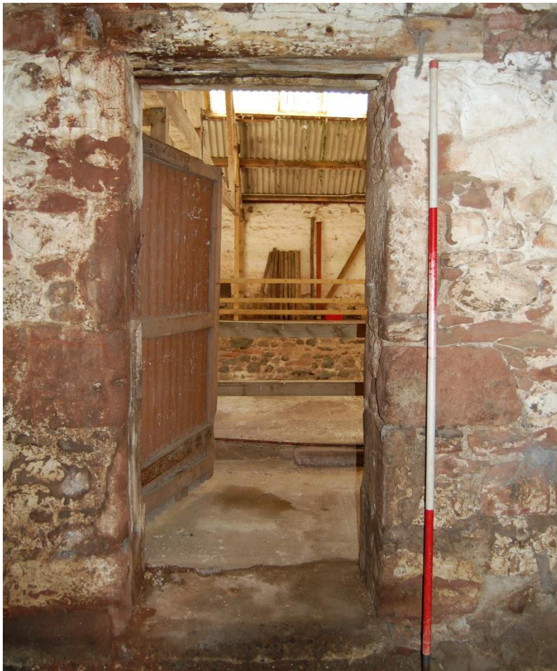
Illus 6 Room 5 door D15 NE façade showing old red sandstone jambs; facing SW
