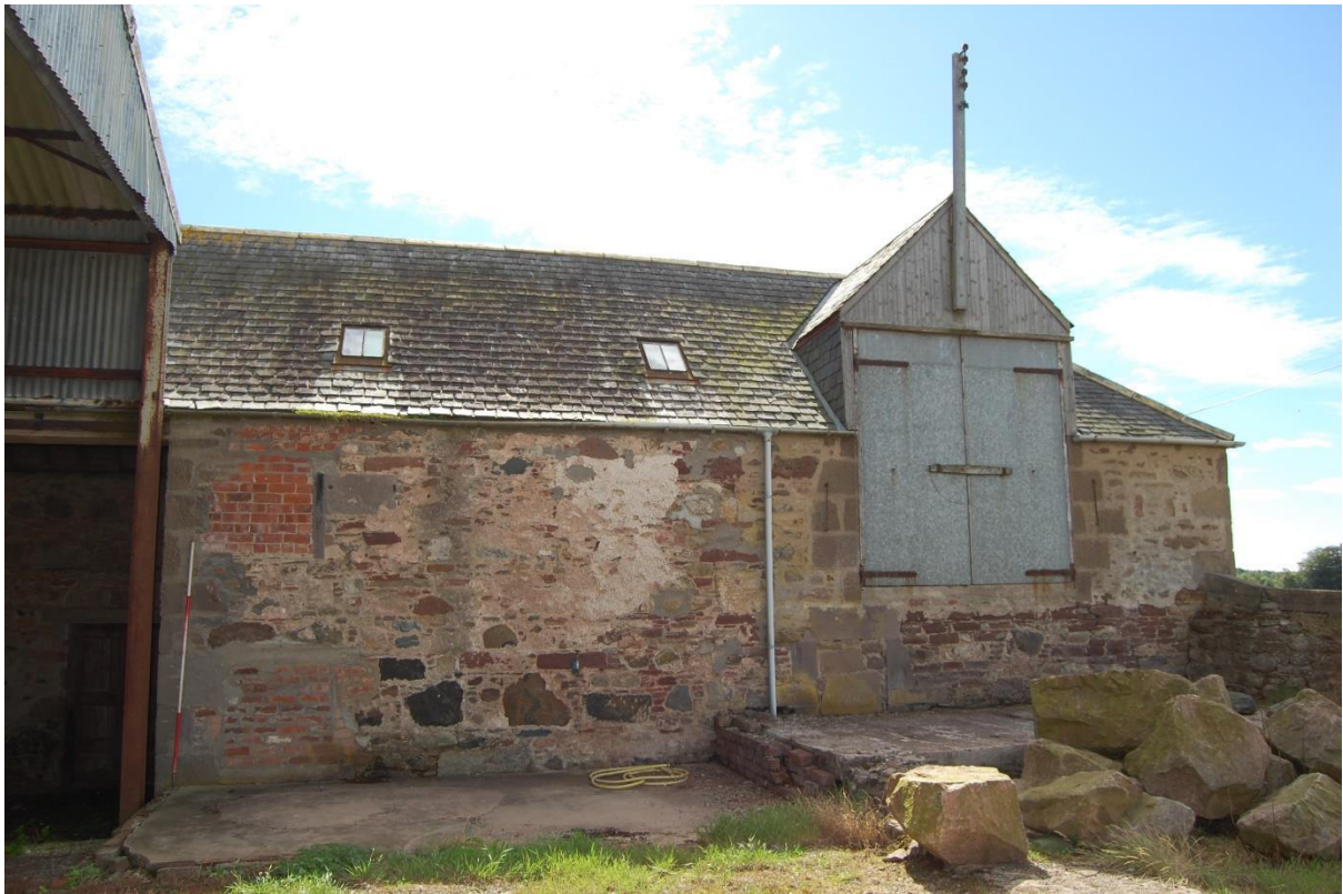
Illus 9 NW façade Room 3 showing probable former location of mill wheel with D16 (right) F3 (centre) and brick-blocked windows W17 and W11 (right of ranging rod) with Door D17 (left)
