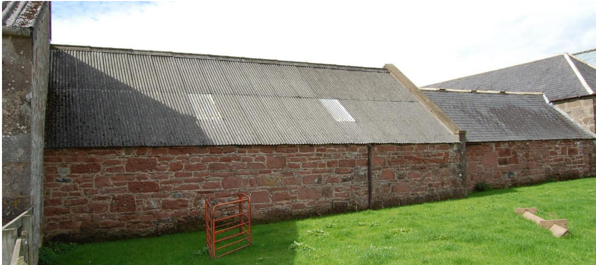
Illus 3 NE exterior walls Phase 1 Room 5 (left) Room 4 (right) showing red sandstone construction; facing WNW
