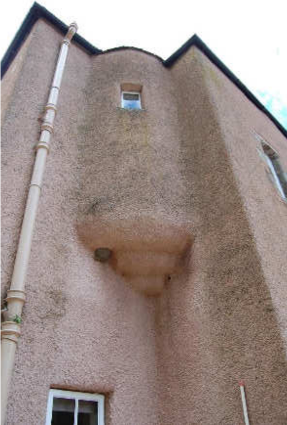
Illus 8 Exterior of corbelled turret stair F8 with W22 (top); facing NW
