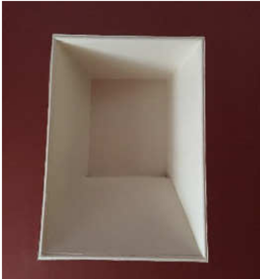
Illus 19 Window W31 on the stair between 1 st and 2 nd floors. This would have opened to the exterior of the SSE wall of the tower
