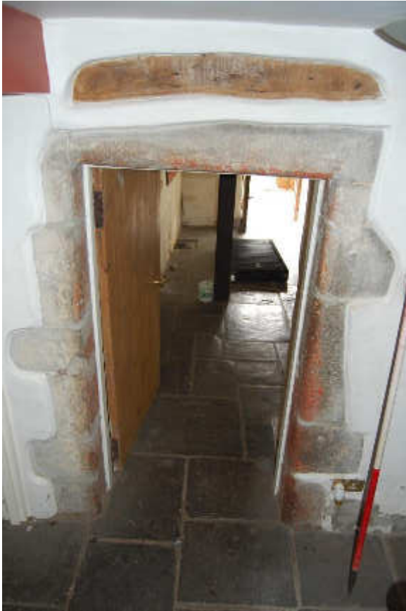
Illus 11 Door D6 ENE face leading from WSW door to gardens with grey sandstone mouldings; facing WSW
