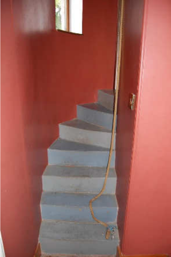
Illus 7 Stair turret F8; is this an original feature or a 19 th -century addition?; facing SSE
