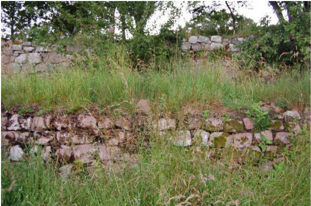
Illus 26 Overgrown and dilapidated terraced walled gardens between F11 and F12; facing NW
