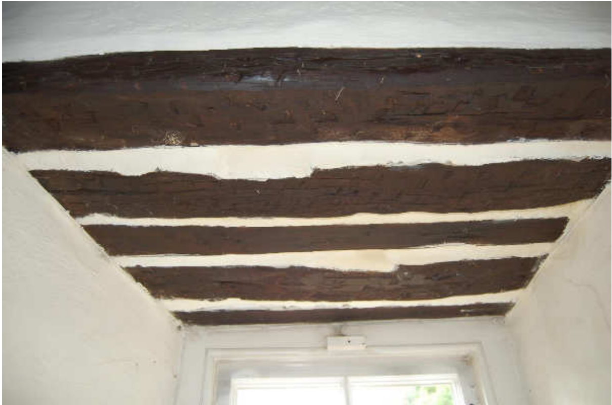
Illus 13 Detail of wooden beam lintel above window W3 showing thickness of wall; facing WSW
