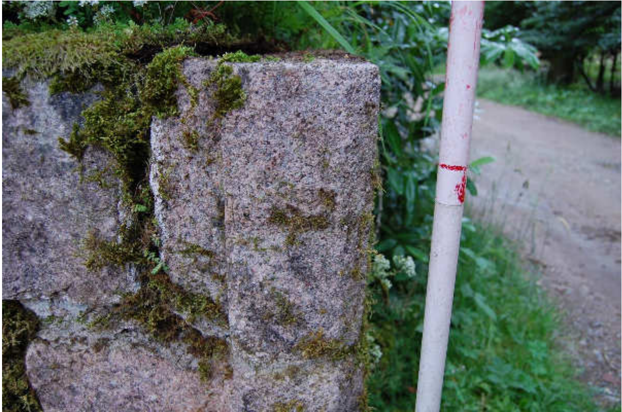
Illus 23 Chamfered pink sandstone gate jamb NE end SE wall of walled garden F10; the other jamb has been removed
