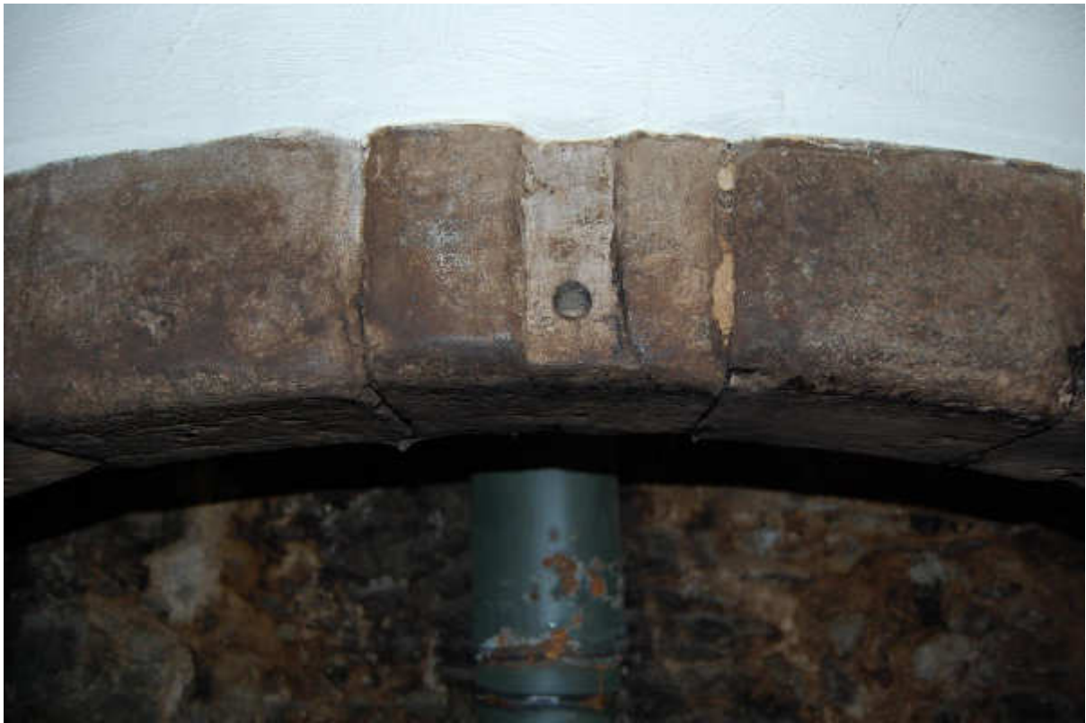
Illus 15 Inglenook fireplace F3 detail of central lintel of grey sandstone and recess for fittings; facing SSE
