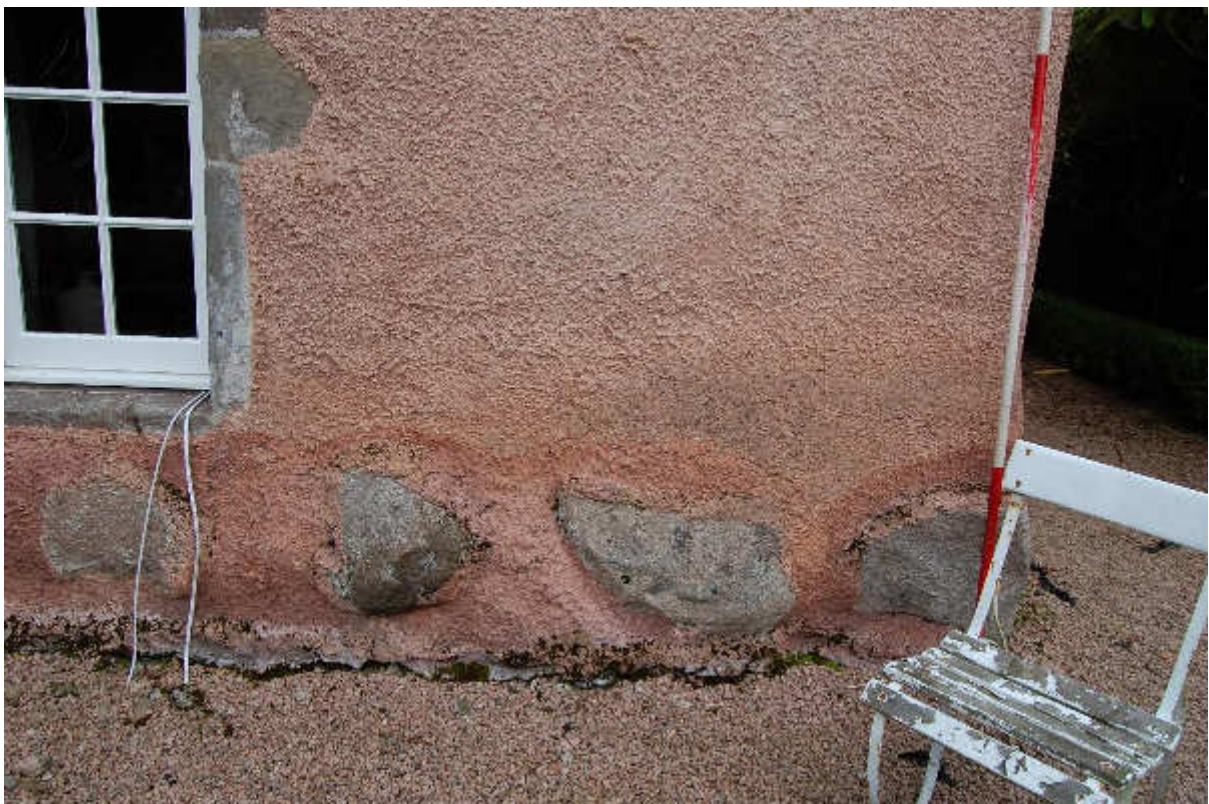
Illus 10 Large grey sandstone foundation (F4) at SW corner Phase 1 house; facing ENE
