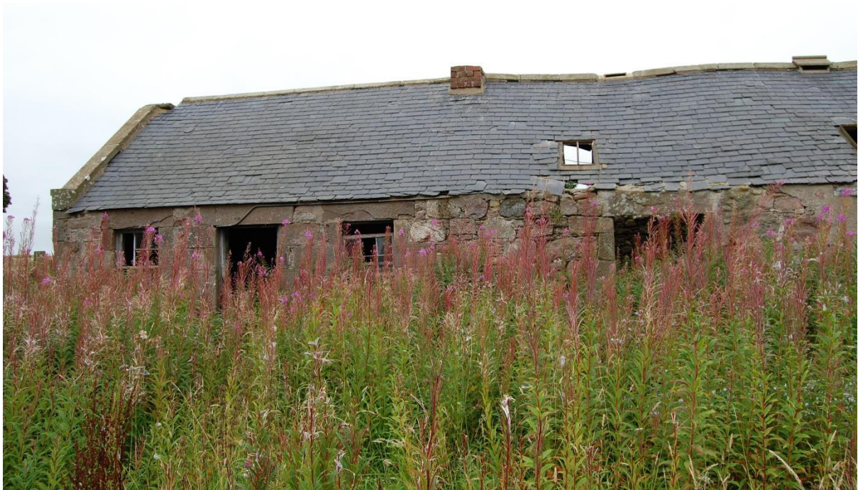
Illus 16 Building 5 SW façade showing overgrown state and poor condition of roof; facing SW
