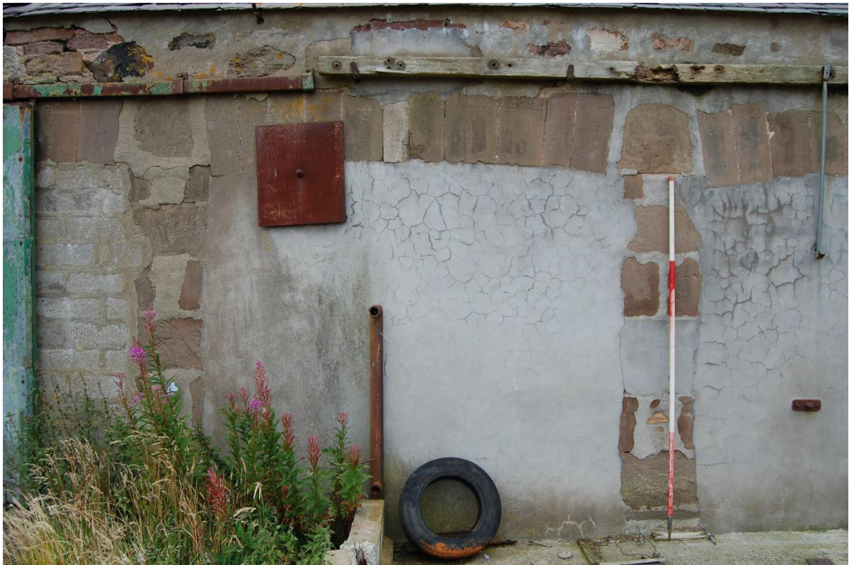
Illus 7 Cart door D16, one of four cart doors in SW wall Building 1; facing NE
